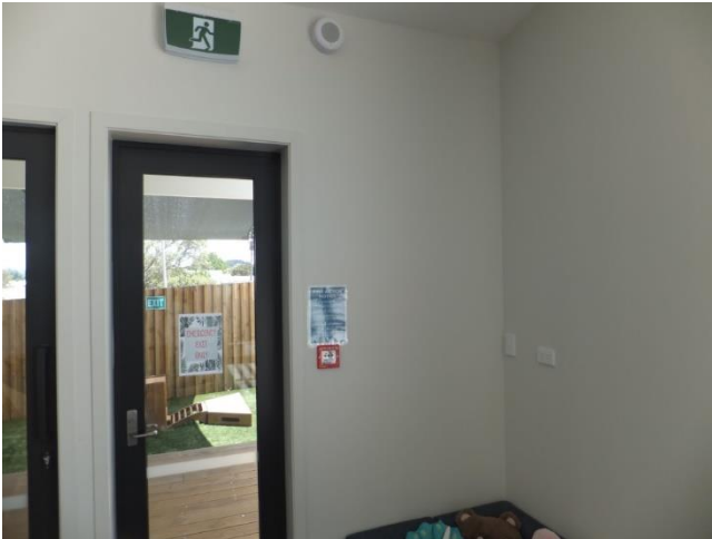
Illuminated exit sign and manual call point
