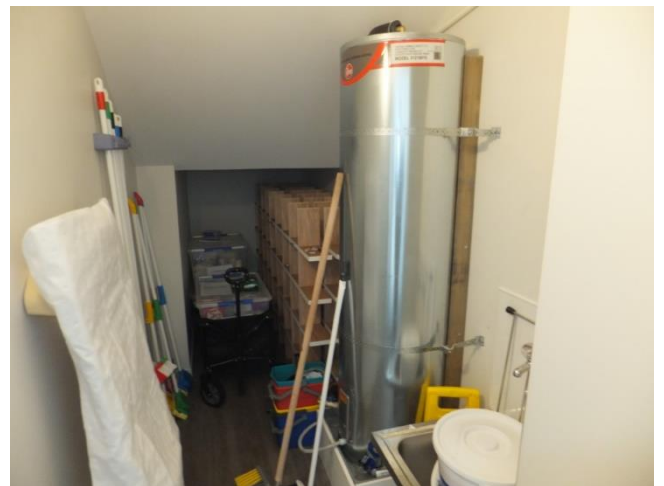
Hot water cylinder / generator
