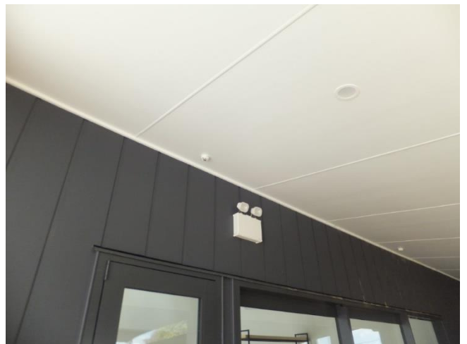
External general lighting and emergency lighting
