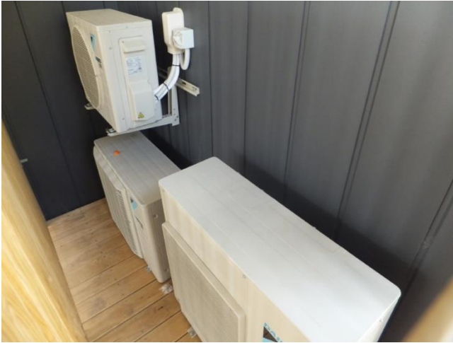
Outdoor split system AC units (condensers)
