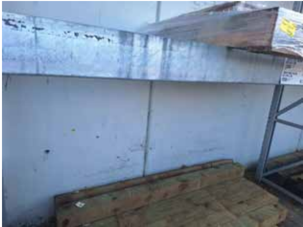
91. Widespread debonding of the sealant to the control joints of the concrete wall panels.
