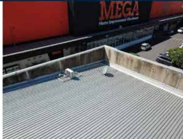
89. Extensive staining on the internal face of the concrete wall panels.
