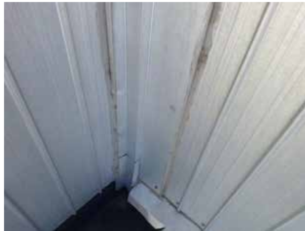
47. Localised debonding to the internal corner cappings of the profiled metal internal parapet sheets.
