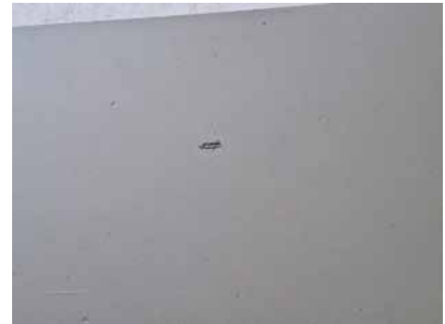
42. Localised exposed reinforcement bars to the concrete wall panels.
