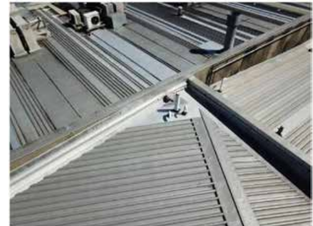
18. Deterioration of the sealant at the chased-in apron flashing.
