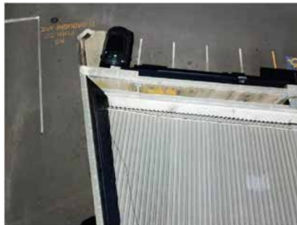
5. Staining on the single-plywood membranes at the internal gutters.
