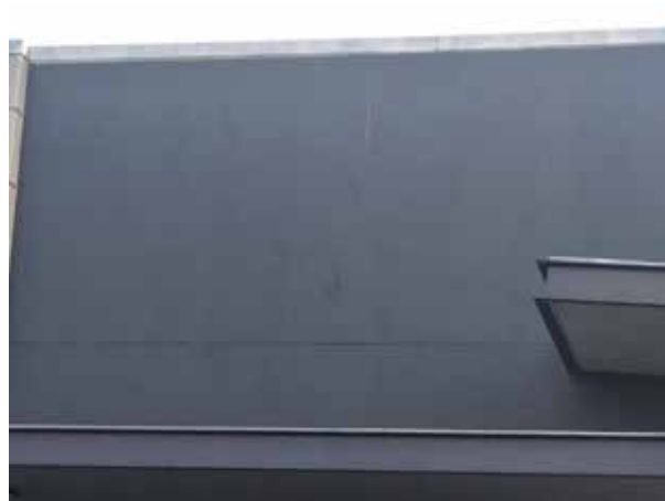
23. Localised blistering of the paint finish to the upper-level horizontal concrete wall panels.
