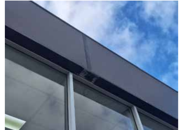
81. Sporadic areas of deterioration of the finish to the metal fascia sheets.
