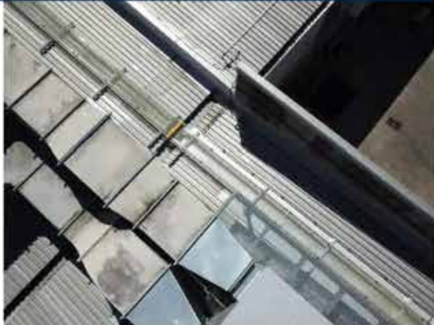
25. Staining and deterioration of the single-plywood membranes.
