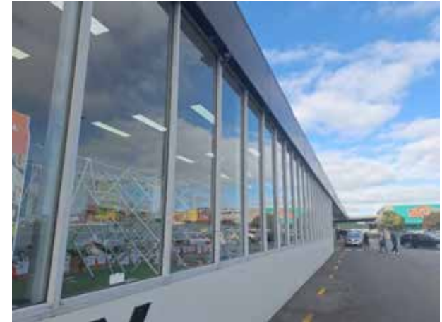
135. Sporadic areas of environmental staining to the aluminium shop front units.
