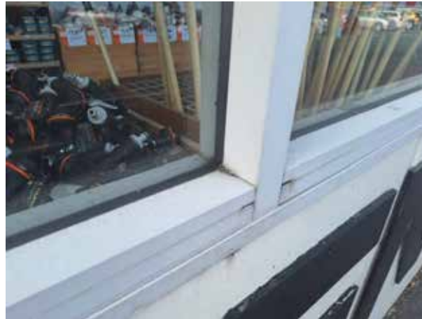
134. Sporadic areas of shrinkage to the glazing seals of the aluminium shop front units.
