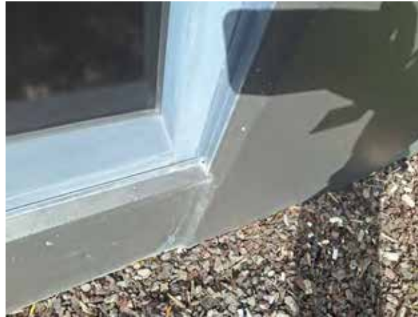
20. Sporadic areas of moisture run-marks to the external face of the concrete base emitting from the aluminium shop front units.
