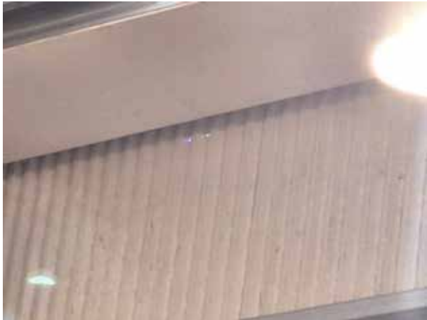
187. Sporadic areas of unsealed fixing or penetration centres to the profiled metal cladding sheets.
