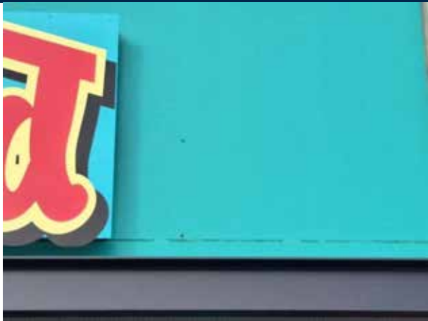
1. Sporadic areas of redundant fixing centres to the upper-level horizontal concrete wall panels.
