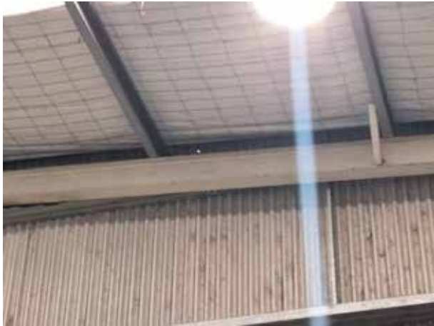
199. Sporadic areas of unsealed fixing or penetration centres to the profiled metal cladding sheets.
