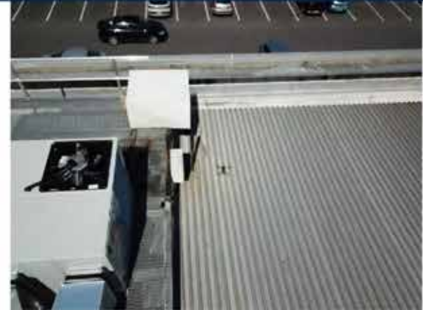
15. Extensive staining and discoloration on the metal walkway.
