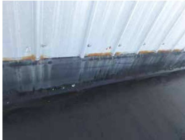
68. Widespread moisture run-marks and discoloration to the upstand of the synthetic rubber sheets.
