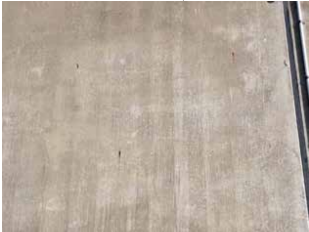
22. Sporadic areas of corrosion staining to the concrete wall panels. The corrosion staining appears to be leaching from the reinforcement bars of the concrete wall panels.
