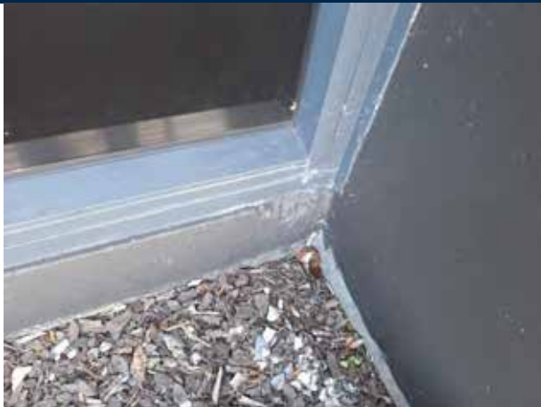
1. Sporadic areas of minor deterioration and spalling to the external face of the concrete base.
