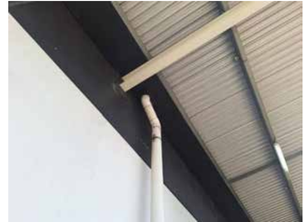
66. Sporadic areas of corrosion to the downpipe brackets of the plastic downpipes.
