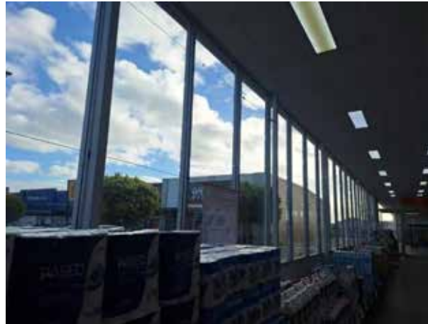
188. Sporadic areas of soil staining to the internal face of the aluminium shop front units.
