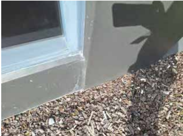
10. Sporadic areas of moisture run-marks to the external face of the concrete base emitting from the aluminium shop front units.
