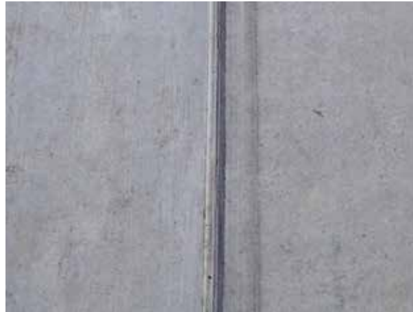
26. Sporadic areas of debonding and cracking to the sealant at the control joints of the concrete wall panels.
