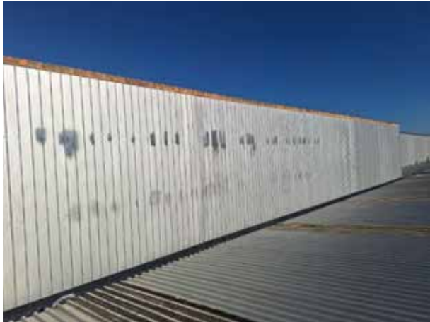
37. Localised area of discolouration to the profiled metal internal parapet sheets.
