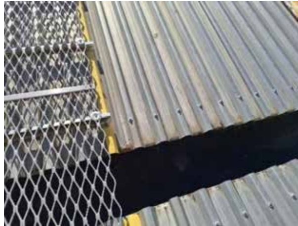
8. Localised corrosion to the sheet edge of the profiled metal roof sheets.
