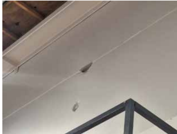
86. Localised deterioration of the edge to the upper-level horizontal concrete wall panels.
