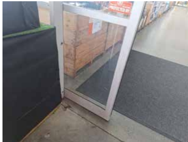
137. Sporadic areas of environmental staining to the aluminium shop front units.
