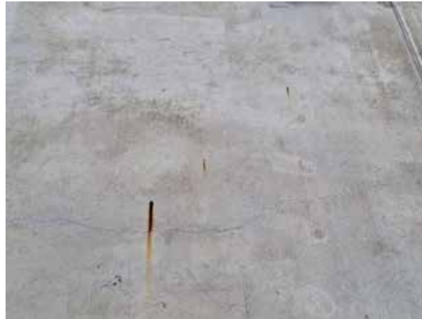
44. Sporadic areas of corrosion staining to the concrete wall panels. The corrosion staining appears to be leaching from the reinforcement bars of the concrete wall panels.
