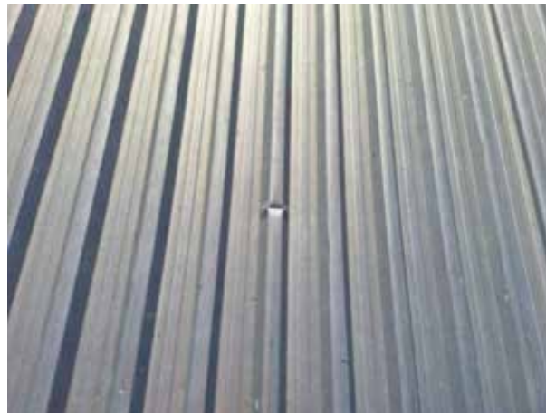
17. Sporadic areas of indentations to the profiled metal roof sheets.
