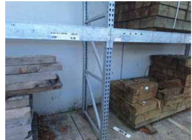
90. Sporadic areas of lichen and vegetation growth to the concrete wall panels at the eastern elevation. The Tenant's racking was installed at this location.
