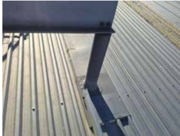
11. Sporadic areas of distortion to the fit-over flashings.
