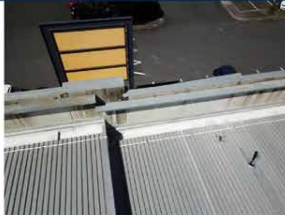
101. Staining and minor uplift to the single-plywood membrane sheets.
