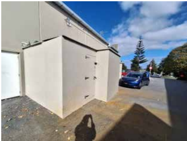
82. Sporadic areas of environmental staining to the plant shed.
