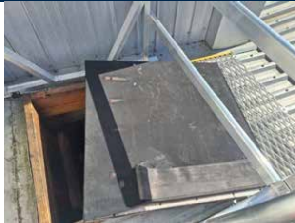
2. Localised partial detachment to the roof hatch.
