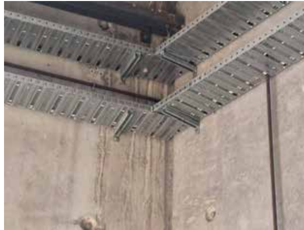
92. Localised moisture run-marks staining to the concrete wall panels and corrosion to the steel beam. This is emitting from the steel beam or internal gutters.
