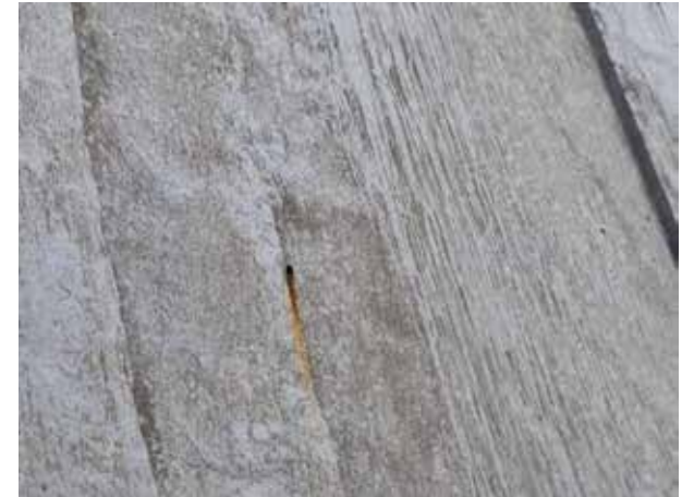
33. Sporadic areas of corrosion staining to the concrete wall panels. The corrosion staining appears to be leaching from the reinforcement bars of the concrete wall panels.
