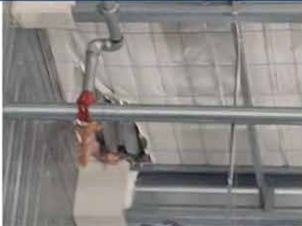
37. A localised tear to the roof underlay.
