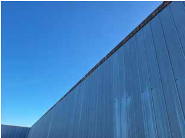
22. Sporadic areas of discolouration to the profiled metal internal parapet sheets.
