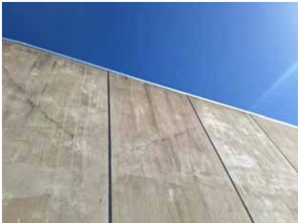
28. Localised area of diagonal surface cracking to the concrete wall panels.
