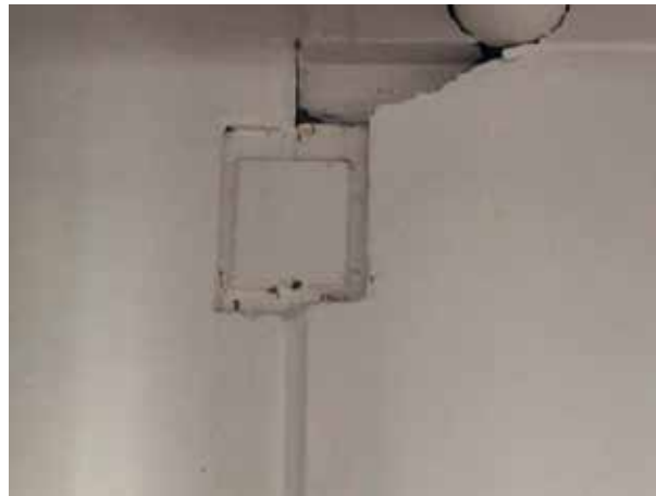
89. Widespread corrosion to the steel embedded plates of the concrete wall panels.
