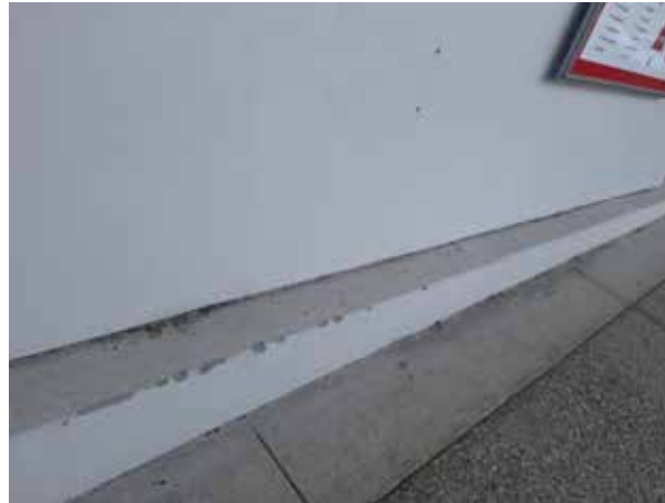
14. Sporadic areas of abrasions and impact damage to the concrete nib walls.
