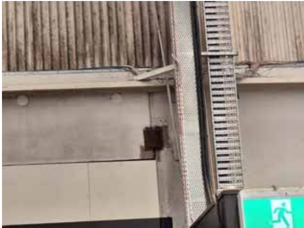
193. Localised corrosion to the steel embedded plates within the concrete wall panels.
