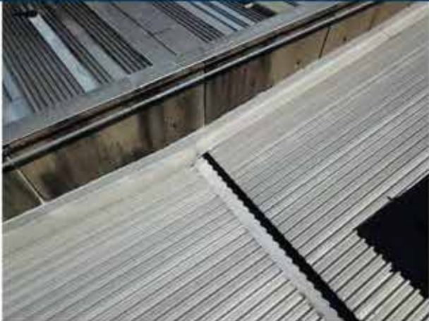
19. Undulation to the single-plywood membrane sheets and distortion to the apron flashings.
