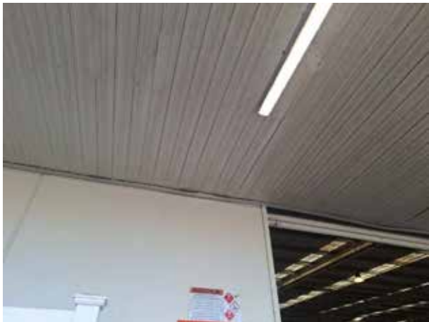
154. Sporadic areas of distortion of the metal trim to the underside of the canopy.
