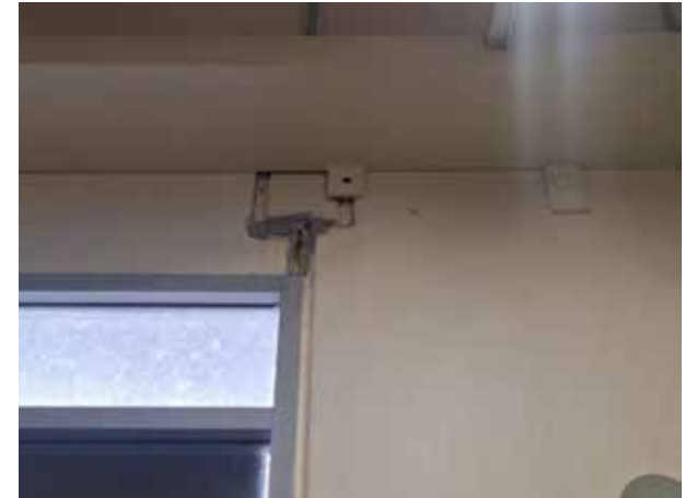
90. Sporadic areas of previous repairs to the control joints and steel embedded plates within the concrete wall panels.
