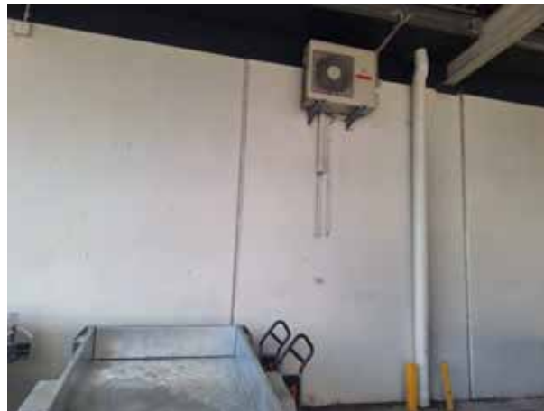
83. Widespread debonding of the sealant to the control joints of the concrete wall panels.
