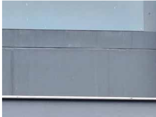
53. Sporadic areas of discolouration to the upper-level horizontal concrete wall panels and emitting from the joint.
