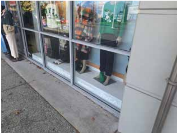
55. Sporadic areas of environmental staining to the aluminium shop front units.
