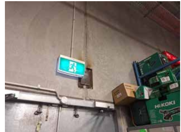
78. Widespread corrosion to the steel embedded plates of the concrete wall panels.
