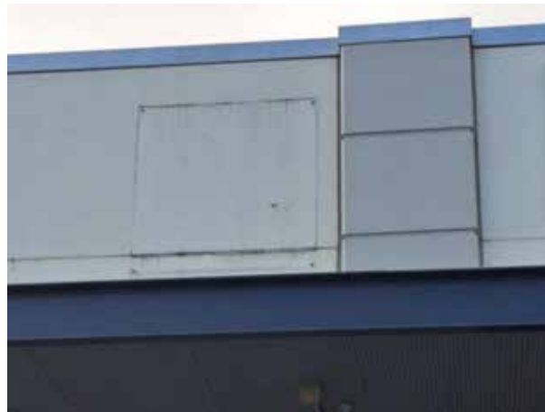
17. Localised removed fixture to the upper-level horizontal concrete wall panels.
