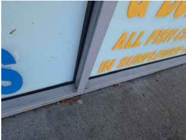
61. Sporadic areas of environmental staining to the aluminium shop front units.
