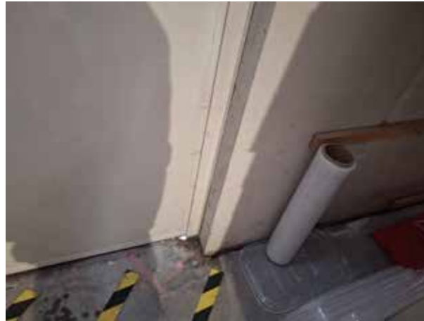
176. Sporadic areas of separation between the concrete floor slabs and concrete wall panels at the metal panelled hinged doors.
