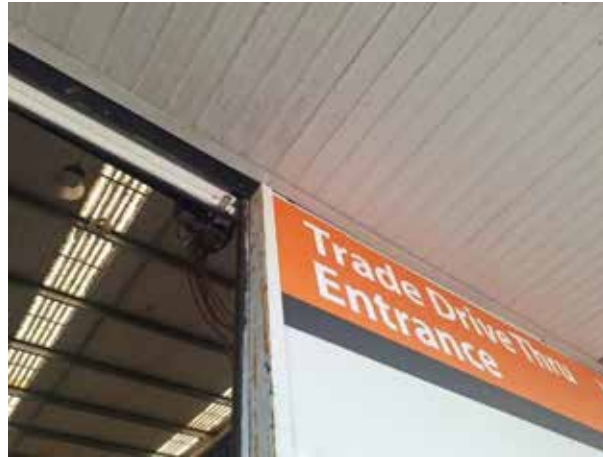
140. Widespread corrosion to the metal opening cappings.
