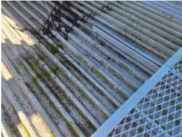
10. Sporadic areas of environmental staining to the roof.
