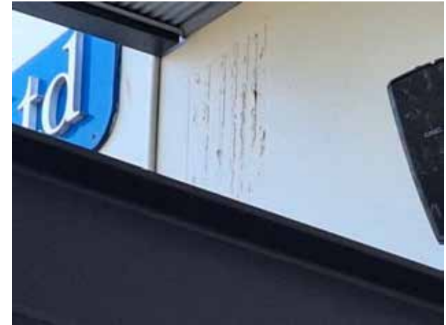
21. Localised residue staining to the upper-level concrete wall panels.
