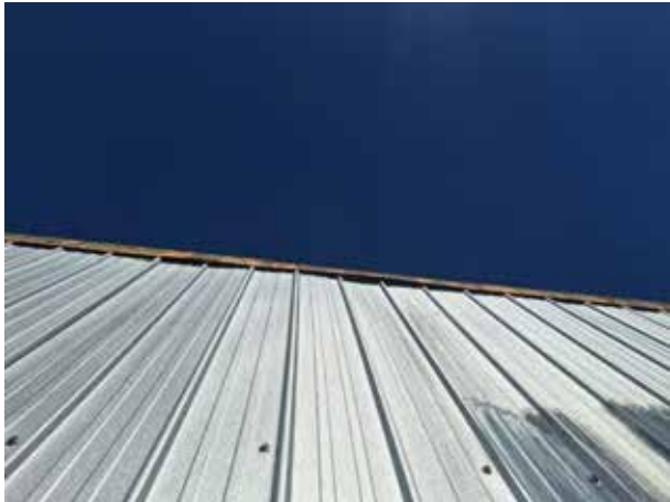
43. Localised area of discoloration to the profiled metal internal parapet sheets.
