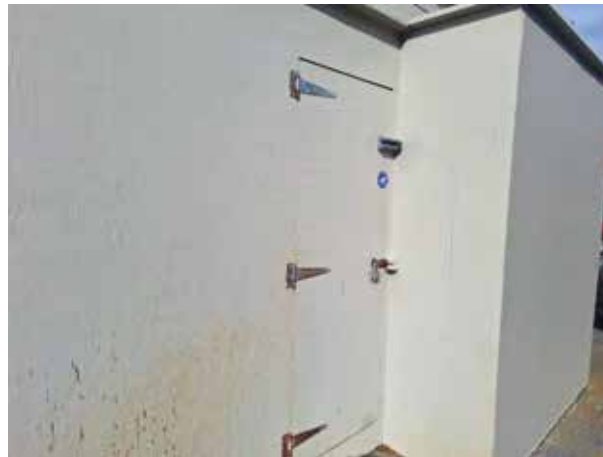
83. Widespread corrosion to the door brackets.
