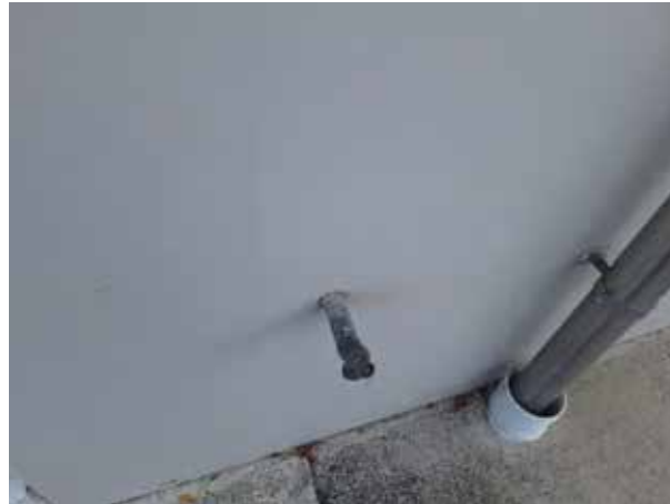
17. Sporadic areas of unsealed tap outlets to the concrete wall panels.
