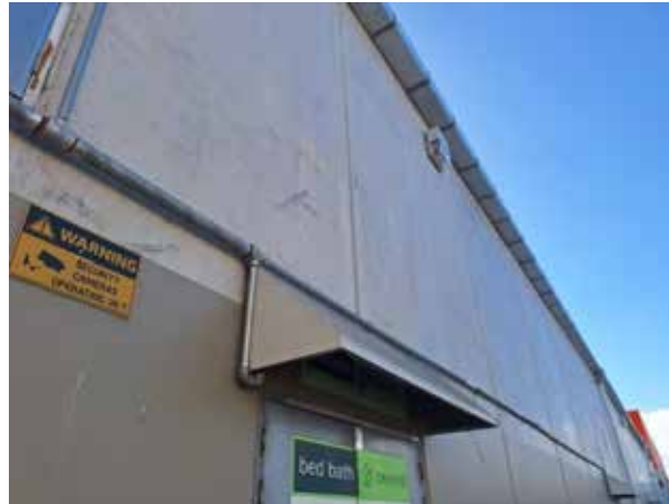
71. Sporadic areas of distortion to the metal door awnings.
