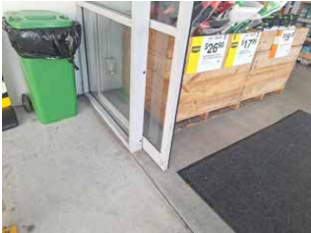
133. Localised abrasions to the automatic sliding doors.
