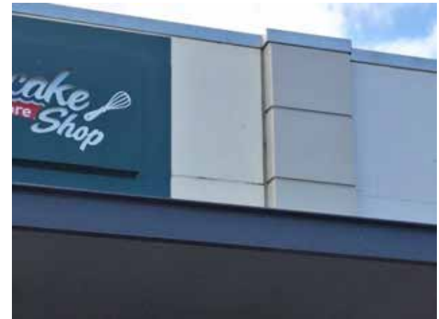
18. Sporadic areas of debonding and discolouration to the joint of the upper-level horizontal concrete wall panels.
