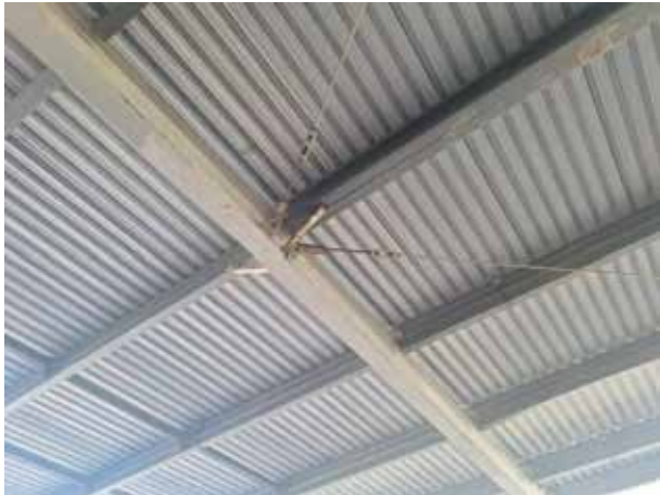
163. Sporadic areas of discolouration and corrosion to the steel canopy frame.
