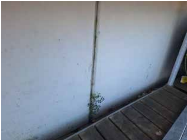
94. Sporadic areas of lichen and vegetation growth to the concrete wall panels at the eastern elevation. The Tenant's racking was installed at this location.
