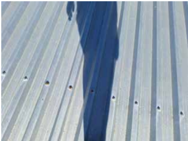
34. Widespread corrosion to the fixings of the profiled metal roof sheets.
