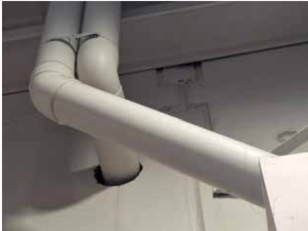
91. Localised unsealed pipe penetration to the concrete wall panels.
