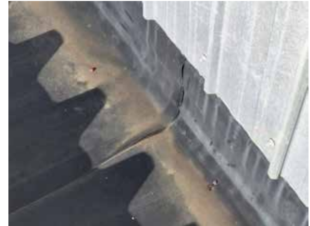
75. Localised minor deboning to the synthetic rubber membrane sheets.
