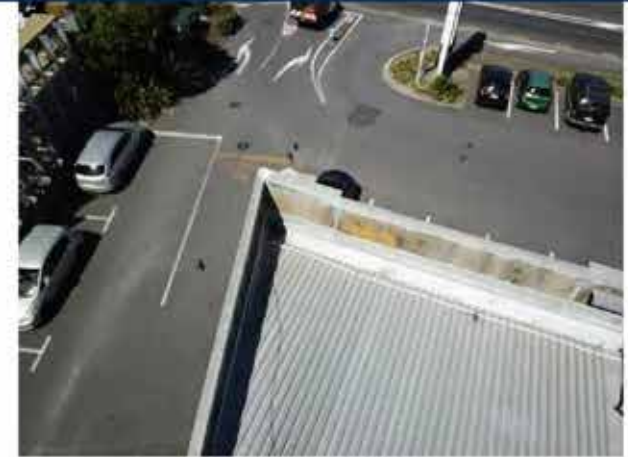
3. Staining on the metal parapet cappings.
