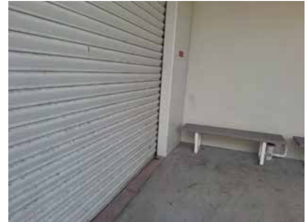
132. Sporadic areas of environmental staining to the metal roller shutter door.
