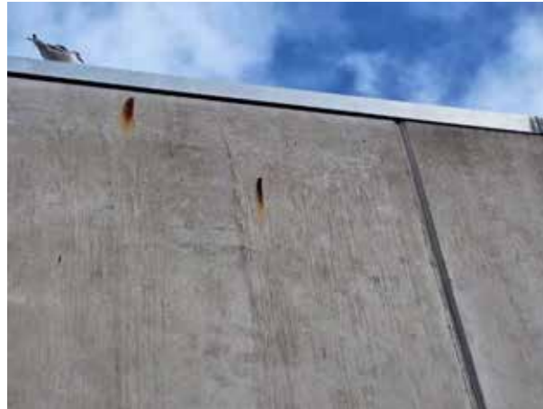
29. Sporadic areas of corrosion staining to the concrete wall panels. The corrosion staining appears to be leaching from the reinforcement bars of the concrete wall panels.
