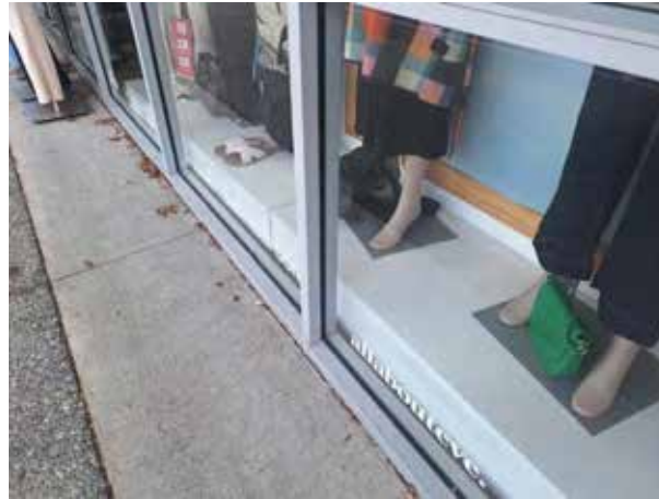
56. Sporadic areas of environmental staining to the aluminium shop front units.
