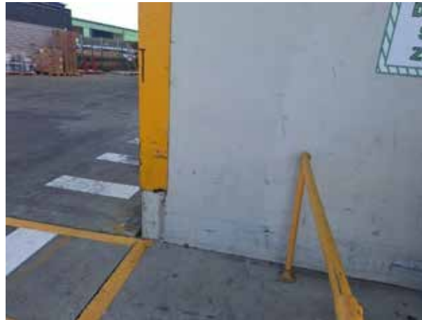
98. Widespread deterioration of the finish to the lower half of the concrete wall panels.
