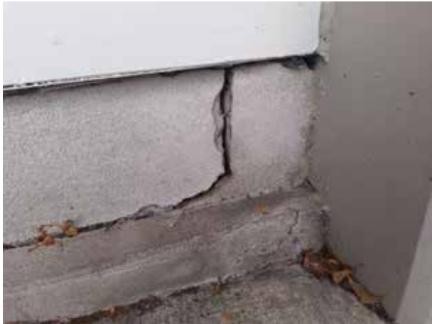
13. Localised cracking to the external face of the concrete base.
