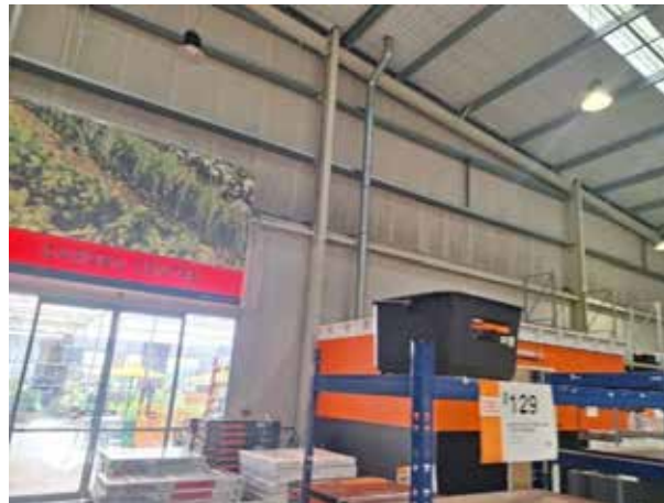
173. Widespread soil staining to the internal side of the elevations.
