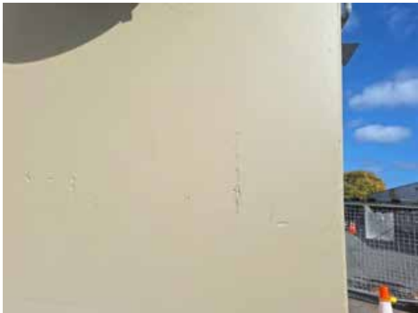
46. Sporadic areas of deterioration and spalling to the concrete wall panels.
