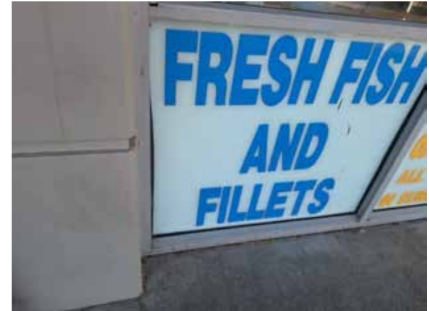
60. Localised partial detachment to the glazing seal from the aluminium shop front units.
