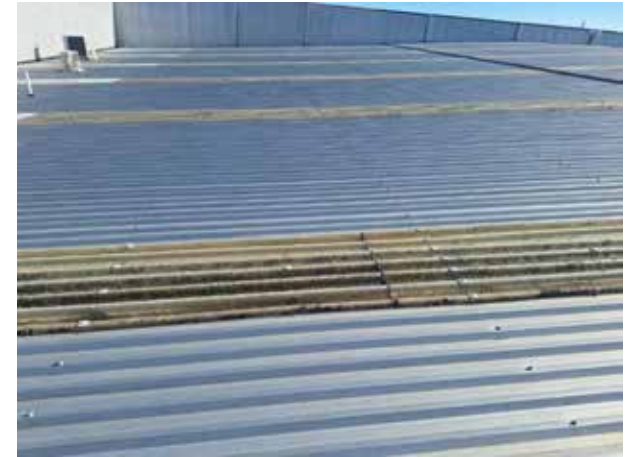
9. The fibreglass sheets were in an aged condition.
