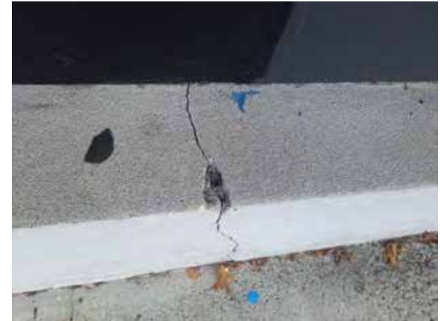
9. Localised cracking to the concrete nib walls.
