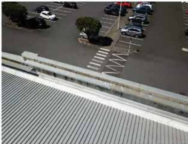
98. Staining and minor uplift to the single-plywood membrane sheets.
