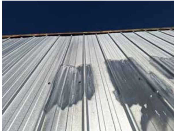
44. Localised area of discoloration to the profiled metal internal parapet sheets.
