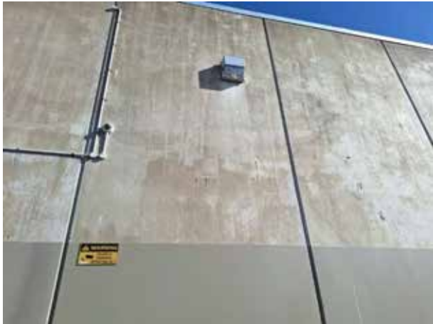
25. Widespread staining and discolouration to the concrete wall panels.
