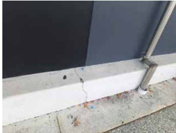
8. Localised cracking to the concrete nib walls.
