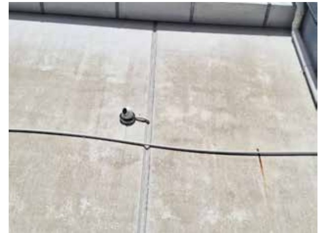
36. Sporadic areas of debonding of the sealant to the control joints of the concrete wall panels.
