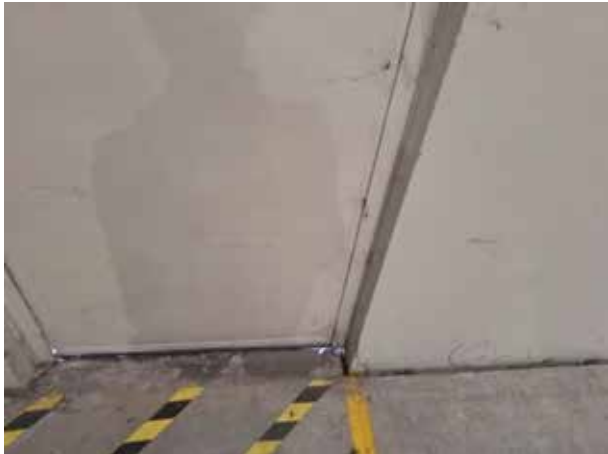
184. Sporadic areas of separation between the concrete floor slabs and concrete wall panels at the metal panelled hinged doors.
