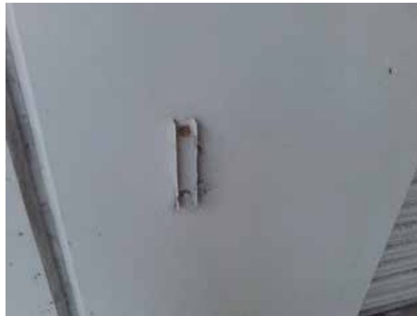
77. Localised corrosion to the fixings of the metal bracket.
