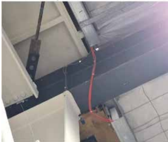
109. A localised tear to the roof underlay, adjacent to a cable penetration.
