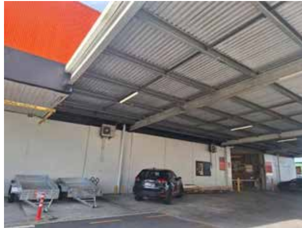
158. Sporadic areas of discolouration and corrosion to the steel canopy frame.
