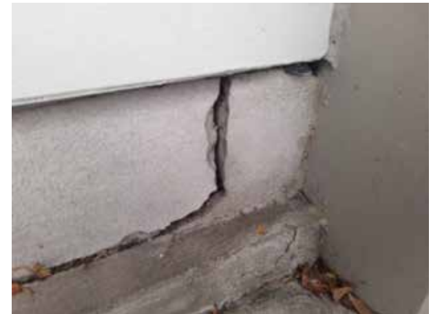
12. Localised cracking to the external face of the concrete base.
