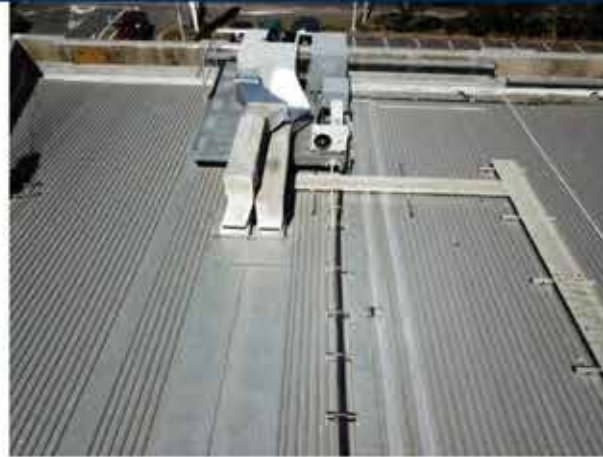
2. Areas of staining on the fit-over flashings.
