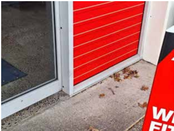
52. Sporadic areas of scuff marks and abrasions to the aluminium shop front units.
