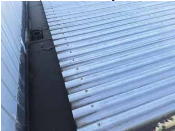
28. Widespread corrosion to the fixings of the profiled metal roof sheets.
