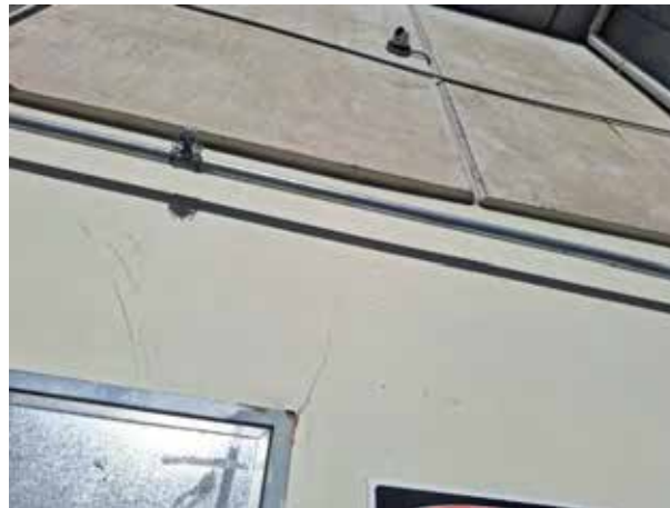
35. Localised area of cracking to the fibre-cement cladding sheets.
