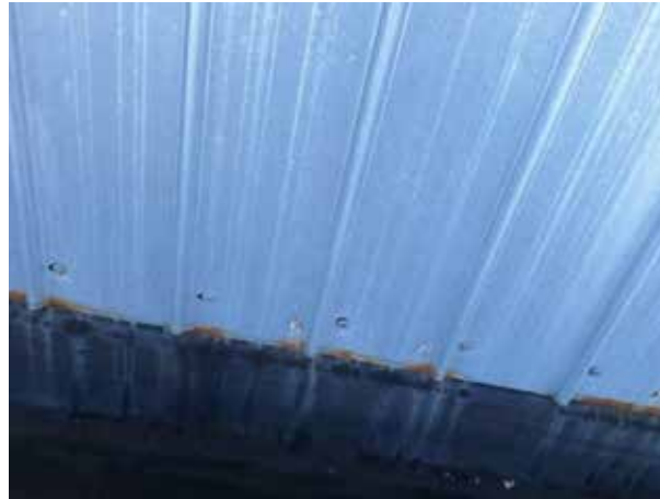
26. Sporadic areas of corrosion to the base of the profiled metal internal parapet sheets. The base of the sheets was in close proximity to the upstand of the internal gutter.
