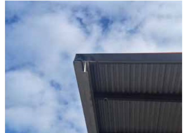
165. Sporadic areas of distortion to the metal barge cappings of the canopy.
