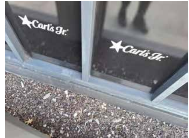
15. Widespread fading to the powder coated finish of the aluminium shop front units.
