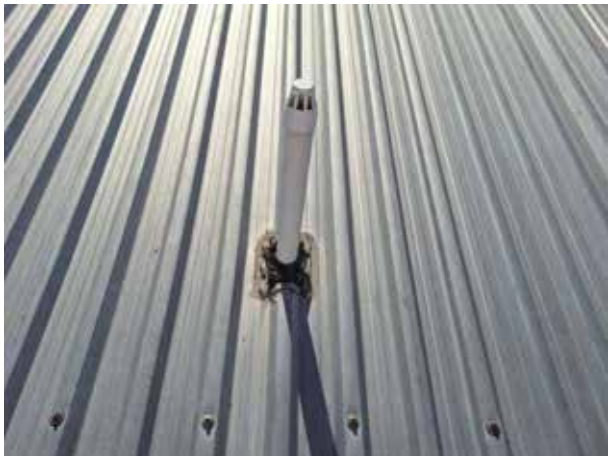
46. The sealant to the vent penetrations was in an aged condition.
