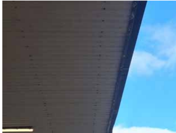
146. Widespread environmental staining to the underside profiled metal canopy sheets.
