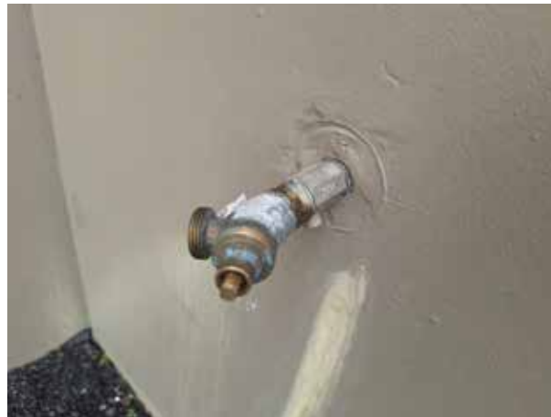
41. Localised minor deterioration to the sealant of the tap outlet.
