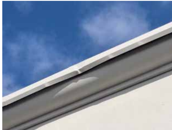
5. Localised distortion to the metal barge cappings.
