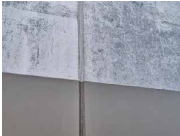
44. Sporadic areas of debonding of the sealant to the control joints of the concrete wall panels.
