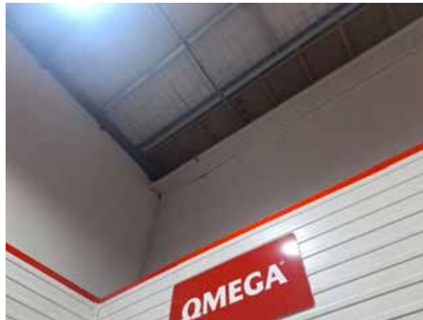
95. Widespread corrosion to the steel embedded plates of the concrete wall panels.
