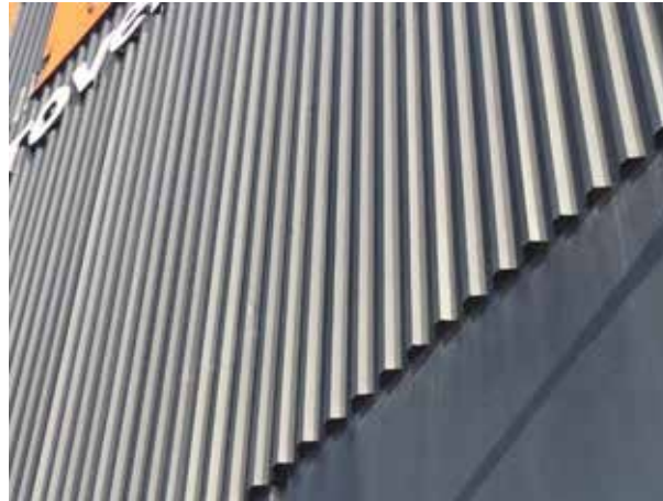
116. Localised indentation to the profiled metal cladding sheets.
