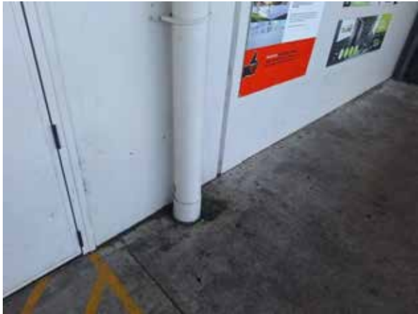
64. Sporadic areas of scuff marks to the plastic downpipes.
