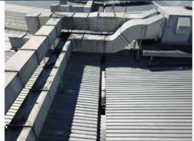
21. Extensive staining on the single-plywood membrane sheets.
