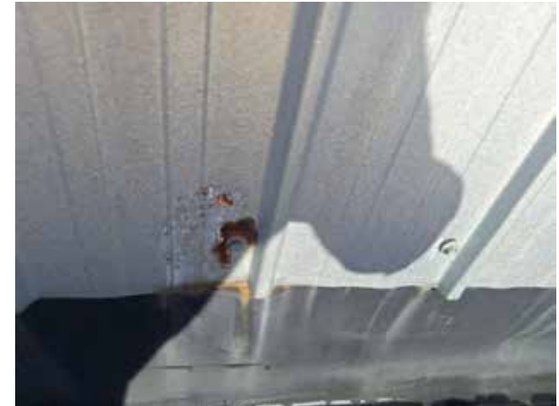
42. Localised extensive corrosion to the profiled metal internal parapet sheets adjacent to a fixing centre.
