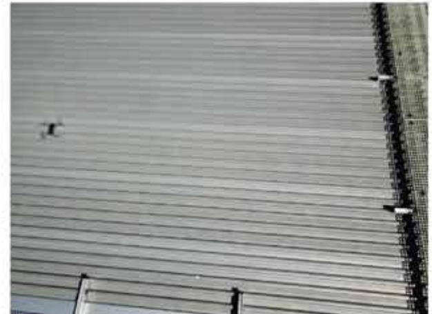
24. Corrosion to the roof sheets' fixings and washers.
