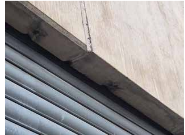
39. Localised spalling and exposed corroded reinforcement bars to the concrete wall panels above an opening.
