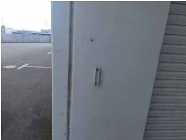
76. Localised corrosion to the fixings of the metal bracket.
