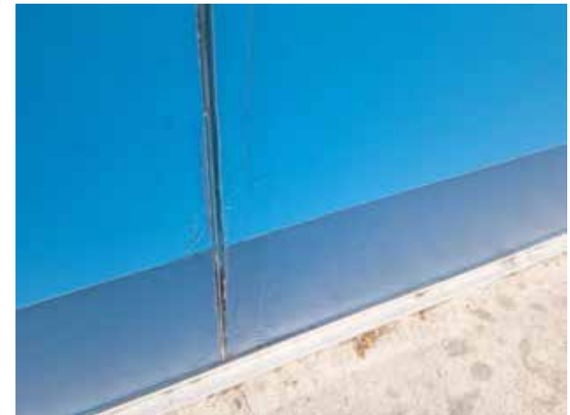
72. Localised debonding of the glazing film to the aluminium shop front units.
