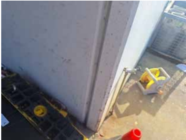
103. Sporadic areas of abrasions, deterioration and spalling to the concrete wall panels.
