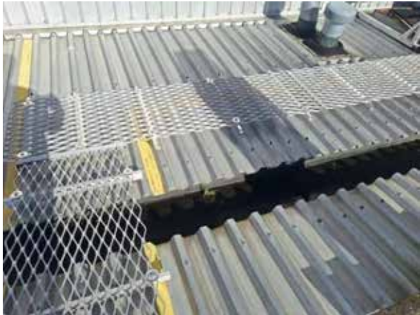
73. Localised vegetation growth to the internal gutters.
