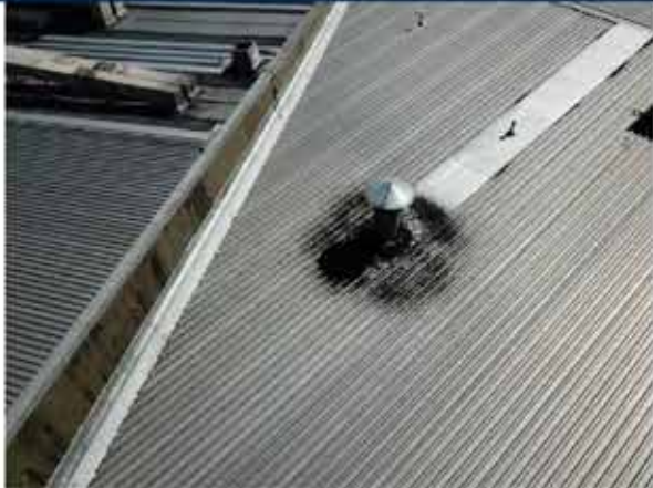
13. Extensive staining and discoloration on the sheets adjacent to a vent penetration.
