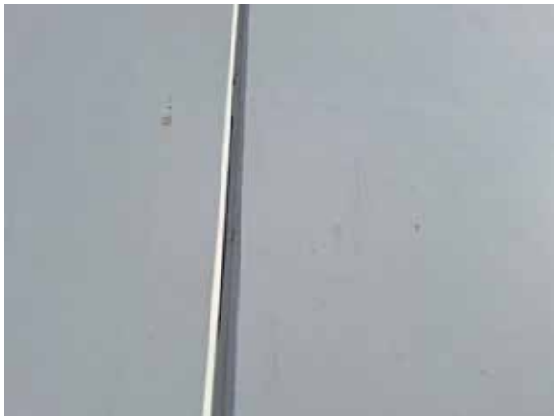
124. Widespread debonding of the sealant to the control joints of the concrete wall panels.
