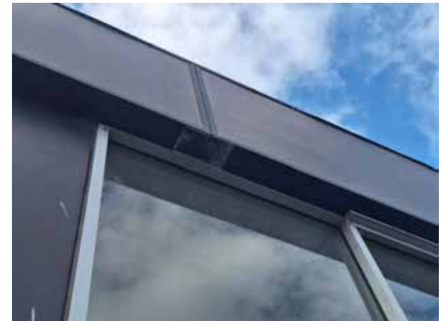
150. Sporadic areas of deterioration of the finish to the metal fascia sheets.
