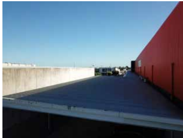
167. Widespread environmental staining to the canopies.
