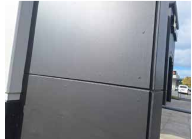
12. Sporadic areas of popping fixings to the fibre-cement cladding sheets.
