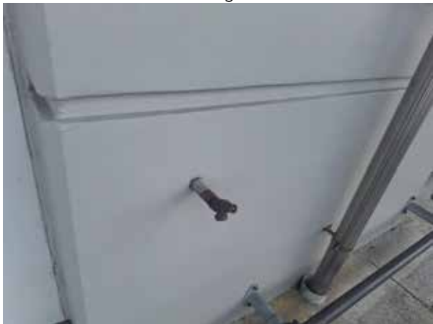
10. Sporadic areas of unsealed tap outlets to the concrete wall panels.
