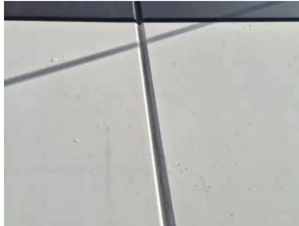
113. Widespread debonding of the sealant to the control joints of the concrete wall panels.
