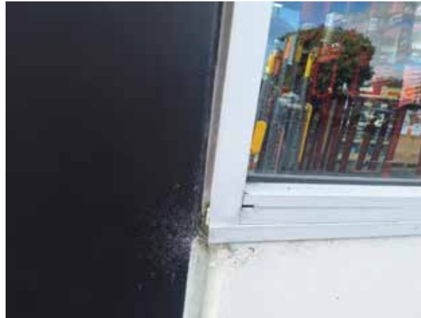
80. Localised mould growth and minor deterioration of the sealant between the concrete wall panel and aluminium shop front units.
