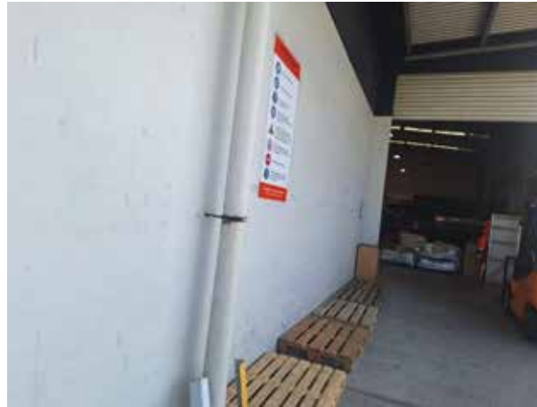
65. Sporadic areas of corrosion to the downpipe brackets of the plastic downpipes.
