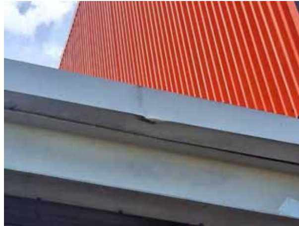
164. Sporadic areas of distortion to the metal barge cappings of the canopy.
