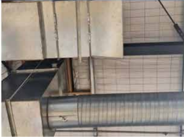
61. Minor wrinkling of the roof underlay adjacent to a large penetration (Bed Bath and Beyond).
