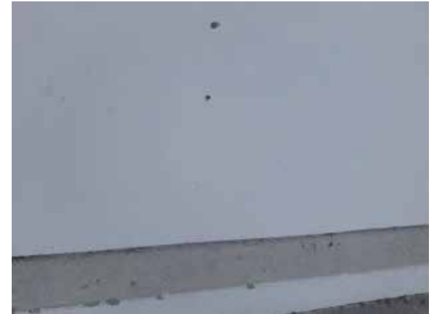
15. Sporadic areas of abrasions and impact damage to the concrete nib walls.
