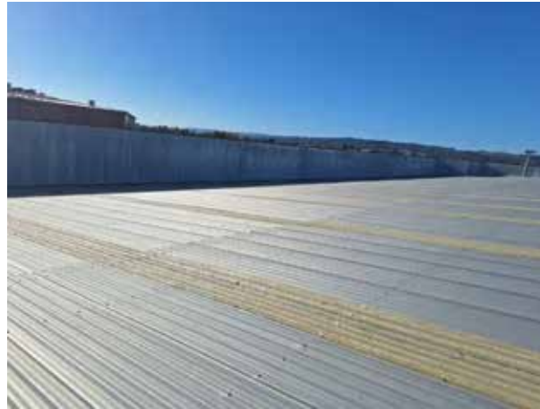
20. The fiberglass sheets were in an aged condition.
