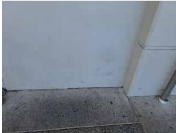
20. Sporadic areas of deterioration of the paint finish to the elevations.
