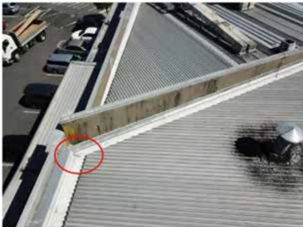
16. Discolouration and residue to the mitre joint of the internal gutters.
