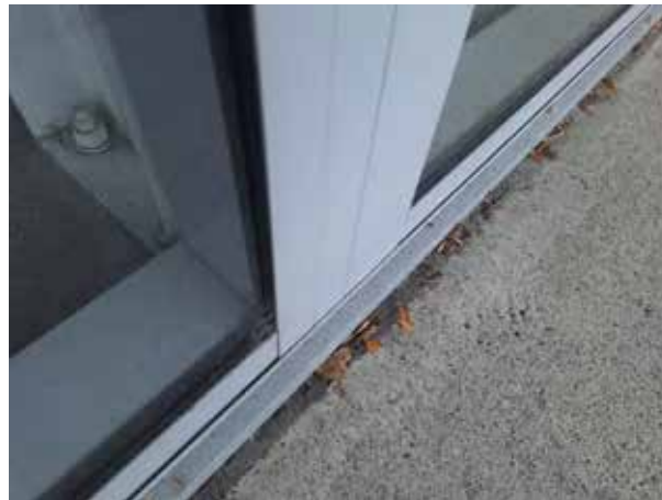
71. Sporadic areas of minor shrinkage of the glazing seals to the aluminium shop front units.
