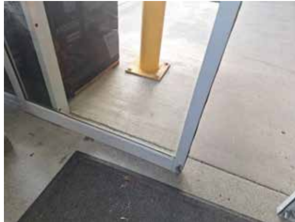
191. Localised abrasions to the internal face of the automatic sliding doors.
