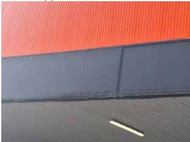
148. Sporadic areas of impact damage and distortion to the metal fascia canopy sheets.
