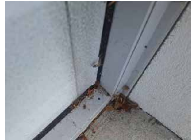
57. Sporadic areas of minor shrinkage of the glazing seals to the aluminium shop front units.
