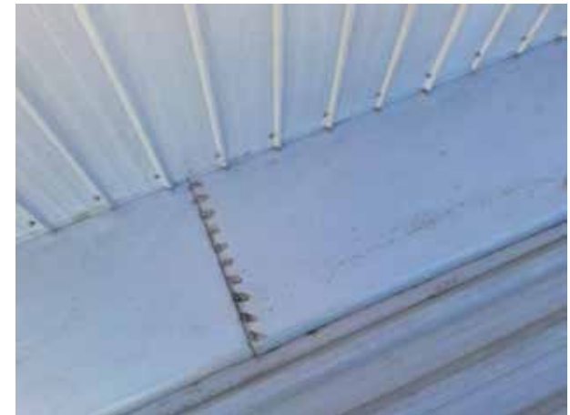
48. Widespread sealant applied to the fixings of the apron flashings.
