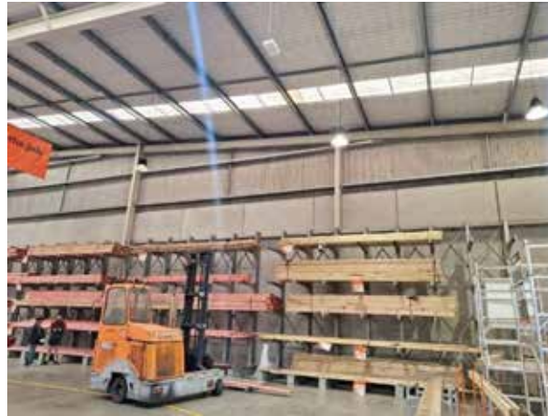
197. Widespread soil staining to the internal side of the elevations.
