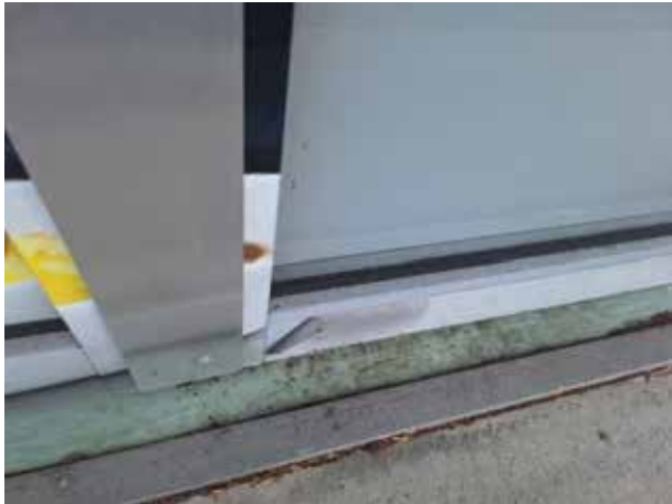
58. Sporadic areas of minor shrinkage of the glazing seals to the aluminium shop front units.
