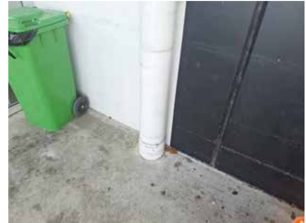
63. Sporadic areas of scuff marks to the plastic downpipes.
