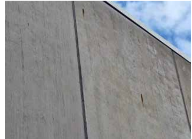
30. Sporadic areas of corrosion staining to the concrete wall panels. The corrosion staining appears to be leaching from the reinforcement bars of the concrete wall panels.
