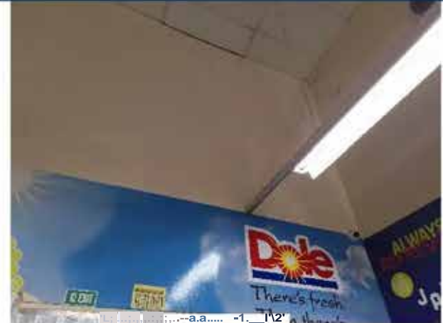
27. Moisture run-marks on the painted plasterboard wall linings (Fruit World).
