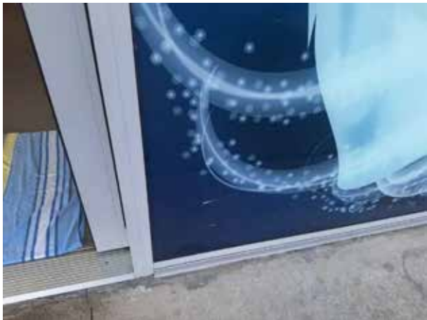
70. Sporadic areas of environmental staining to the aluminium shop front units.
