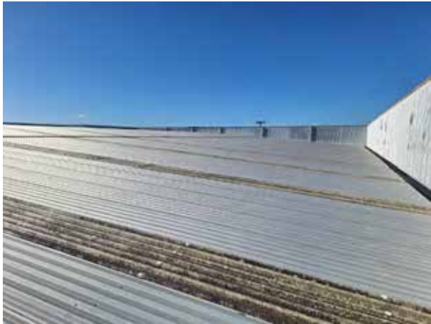
58. The fibreglass sheets were in aged an condition.
