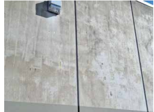
24. Widespread staining and discolouration to the concrete wall panels.
