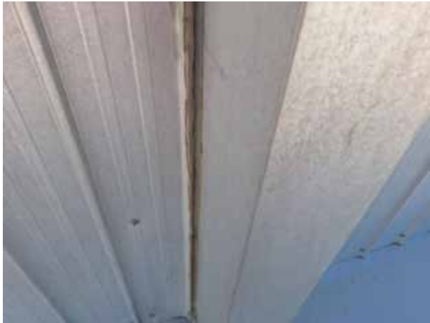
49. Localised debonding to the cappings sheets of the profiled metal internal parapet sheets.
