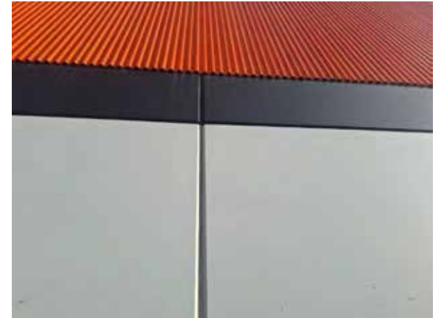
105. Widespread debonding of the sealant to the control joints of the concrete wall panels.
