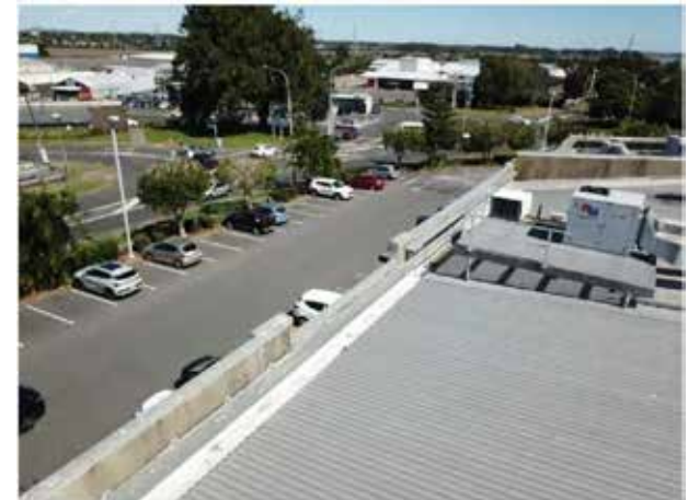
12. Staining on the metal capping and the internal face of the concrete wall.
