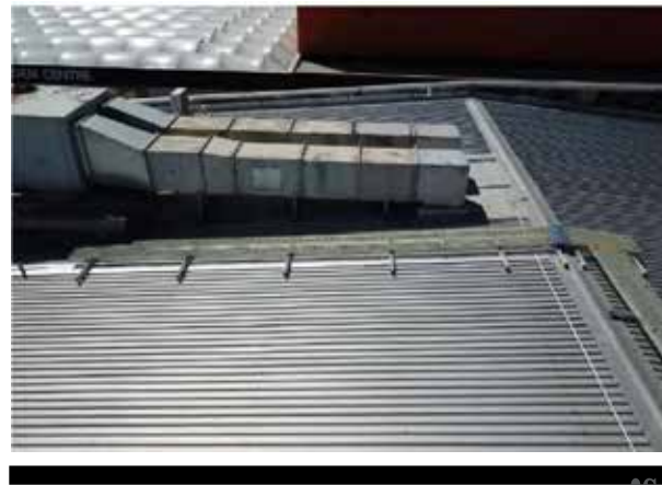
86. Environmental staining on the profiled metal roof sheets.
