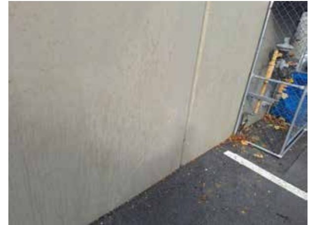
51. Localised surface corner cracking to the base of the concrete wall panels at the western elevation.
