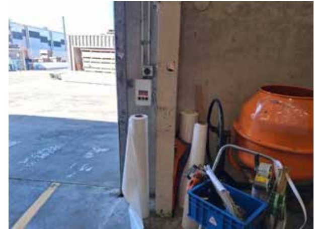
204. Sporadic areas of scuff marks and deterioration of the finish to the steel portal frame.
