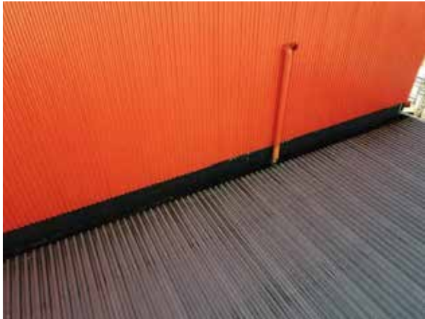
169. Widespread environmental staining to the internal gutter of the canopies.
