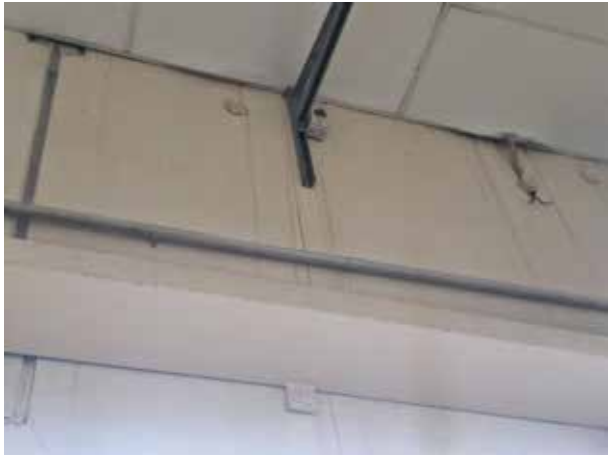
88. Widespread moisture run-marks staining to the concrete wall panels within a tenancy. There was plant equipment installed within the ceiling void.
