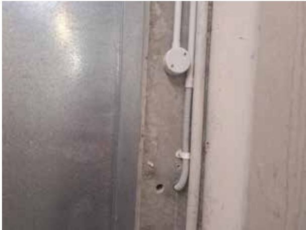
85. Sporadic areas of redundant penetration centres to the concrete wall panels.
