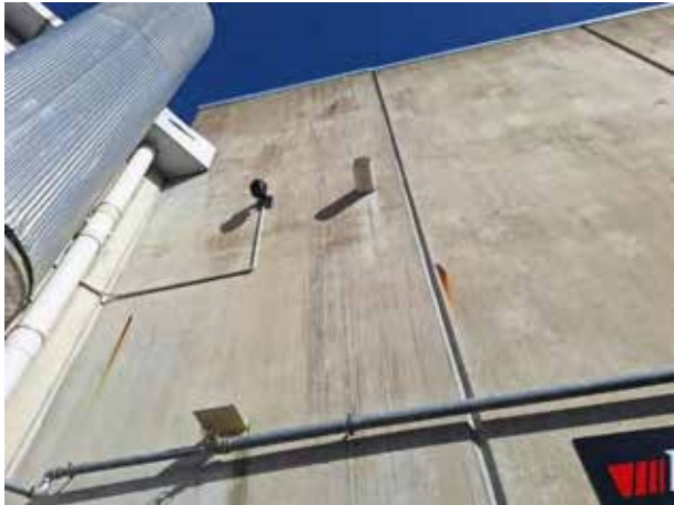
37. Widespread staining and discolouration to the concrete wall panels.
