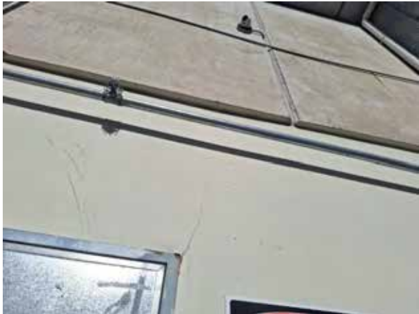
64. Sporadic areas of discolouration and corrosion to the galvanised steel hinged doors.
