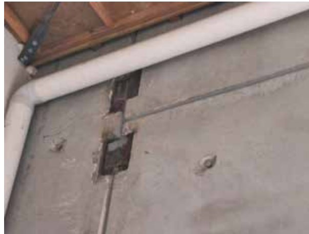
74. Widespread corrosion to the steel embedded plates of the concrete wall panels.
