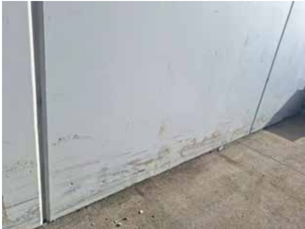
112. Widespread deterioration of the finish to the lower half of the concrete wall panels.
