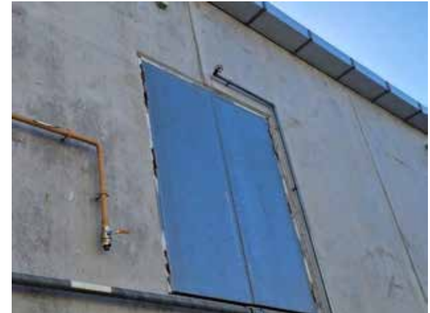
66. Sporadic areas of discolouration and corrosion to the galvanised steel hinged doors.
