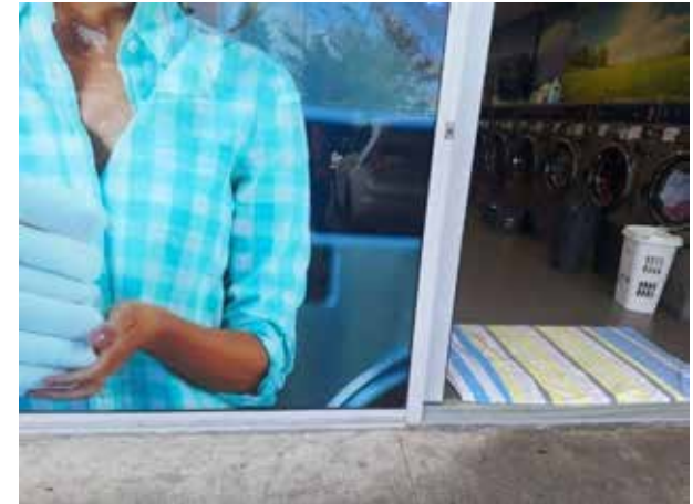
69. Sporadic areas of environmental staining to the aluminium shop front units.
