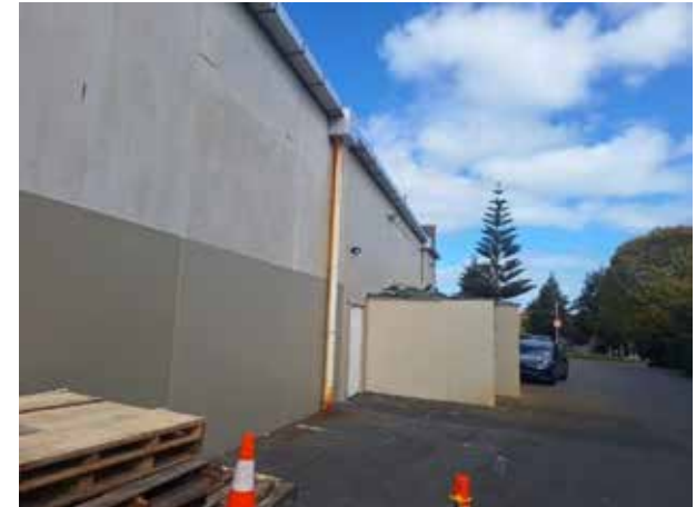
81. Localised extensive staining to the external metal gutter and to the downpipe.
