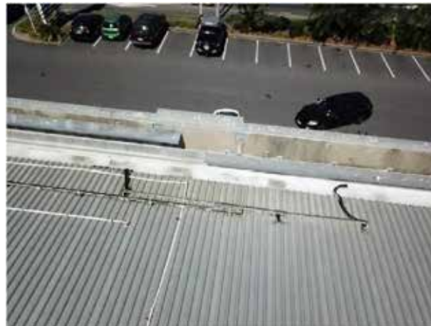
11. Deterioration of the sealant at the apron flashing.
