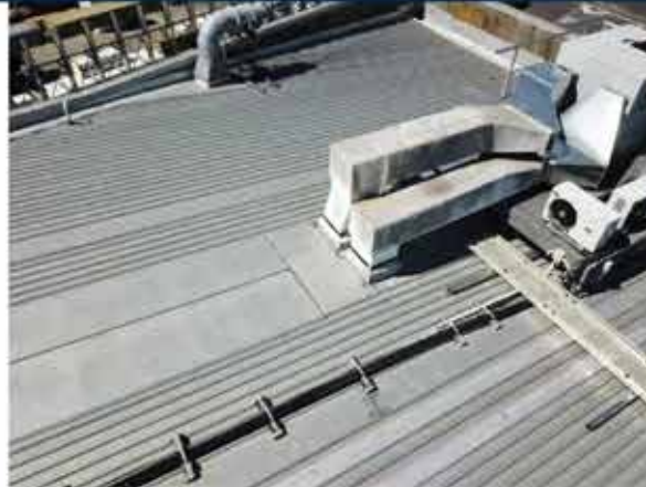
8. Extensive sealant applied to the fit-over flashings and kerb penetrations.
