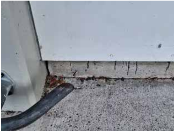
13. Localised area of residue staining to the external face of the concrete base and behind the fibre-cement cladding sheets.
