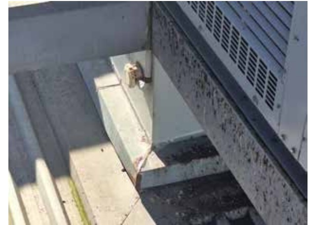
12. Localised corrosion to the ventilation ducting.
