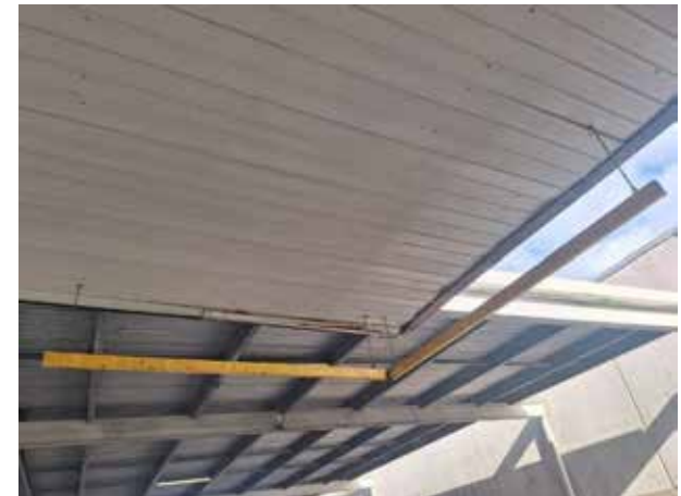
156. Localised corrosion to the metal perimeter trim of the underside of the canopy.
