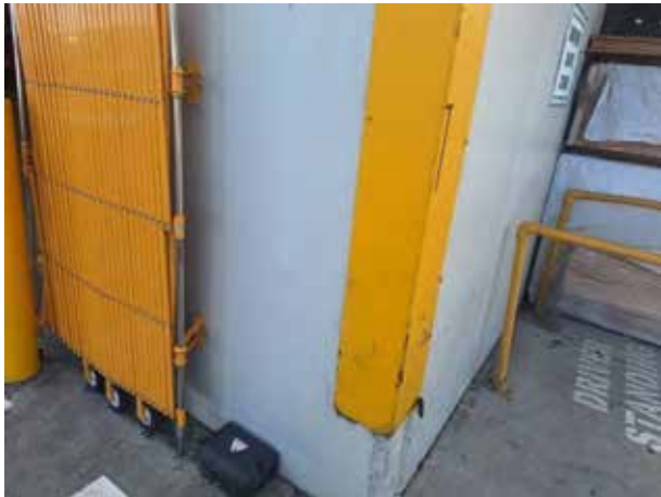
97. Sporadic areas of abrasions and deterioration of the finish to the metal corner cappings of the concrete wall panels.
