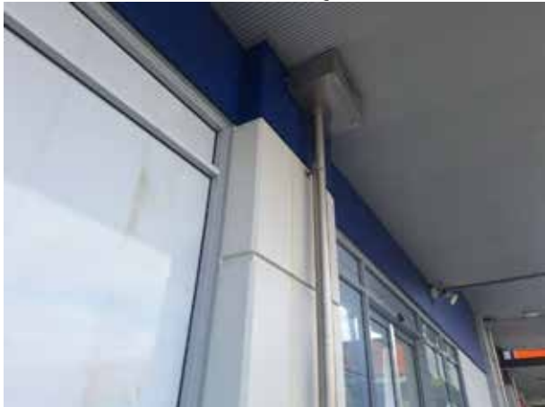
16. Localised corrosion run-off staining to the concrete wall panels emitting from the adjacent stainless-steel downpipe.
