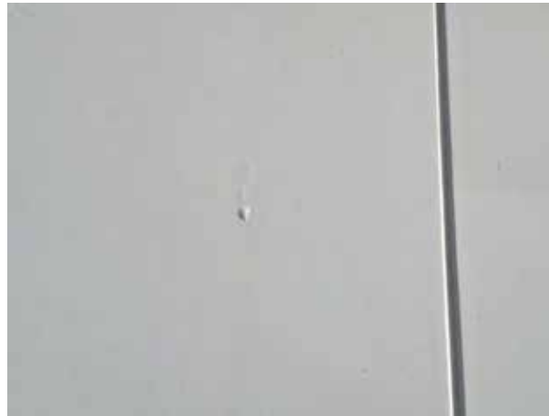
122. Widespread deterioration of the finish to the lower half of the concrete wall panels.
