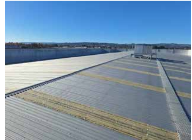
15. The fibreglass sheets were in an aged condition.
