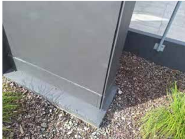
11. Sporadic areas of deterioration of the finish to the fibre-cement cladding sheets.
