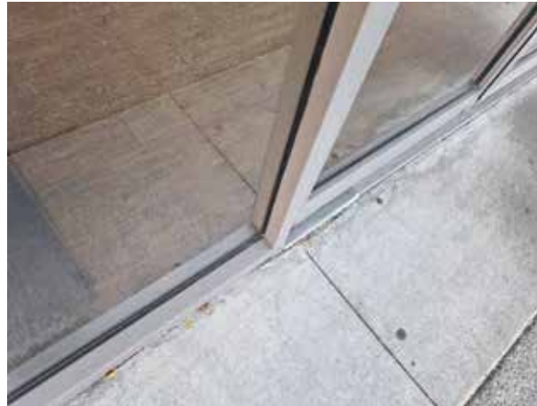
56. Sporadic areas of minor shrinkage to the glazing seals of the aluminium shop front units.
