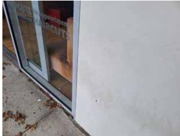
14. Sporadic areas of deterioration of the paint finish to the elevations.
