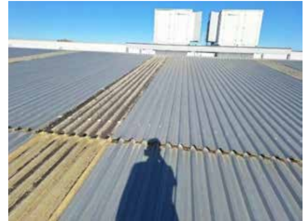
33. Widespread dirt build-up to the stepped junction of the profiled metal roof sheets.
