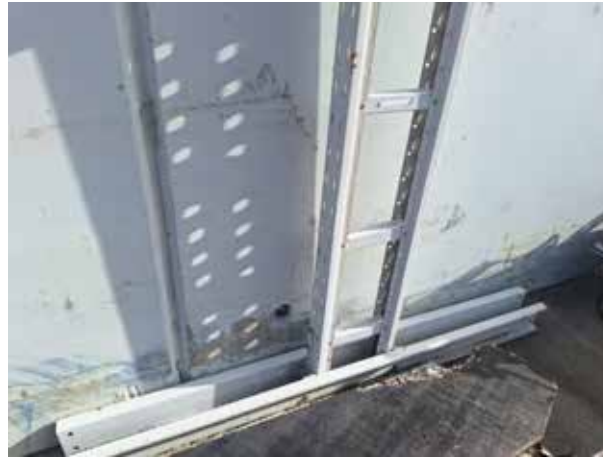
110. Sporadic areas of unsealed penetration centre to the concrete wall panels.
