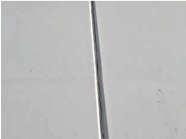
115. Widespread debonding of the sealant to the control joints of the concrete wall panels.
