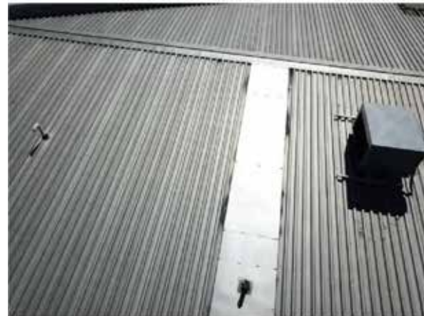
17. Extensive staining and discoloration adjacent to the fit-over flashings.
