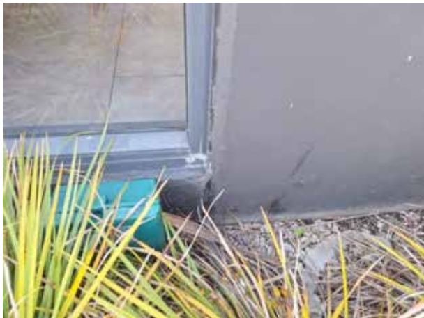
16. Sporadic areas of moisture run-marks to the external face of the concrete base emitting from the aluminium shop front units.
