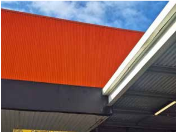
157. Sporadic areas of impact damage and distortion to the metal fascia canopy sheets.
