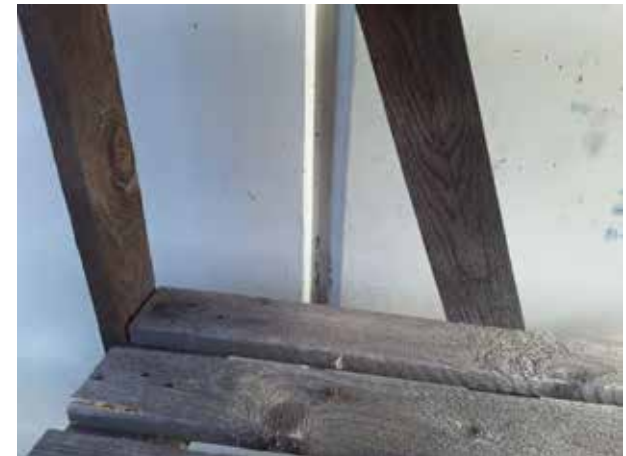
120. Widespread debonding of the sealant to the control joints of the concrete wall panels.
