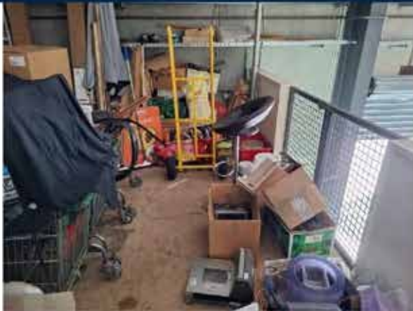
55. Staining on the plywood flooring below a penetration (Fruit World).
