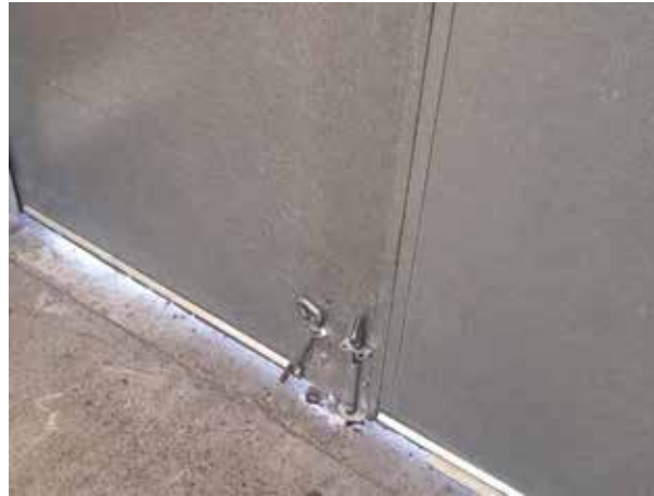
86. Sporadic areas of damage to the door bolt of the galvanised steel hinged doors.
