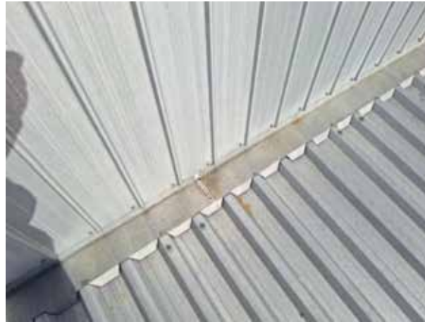
62. Widespread sealant applied to the joints of the apron flashings.
