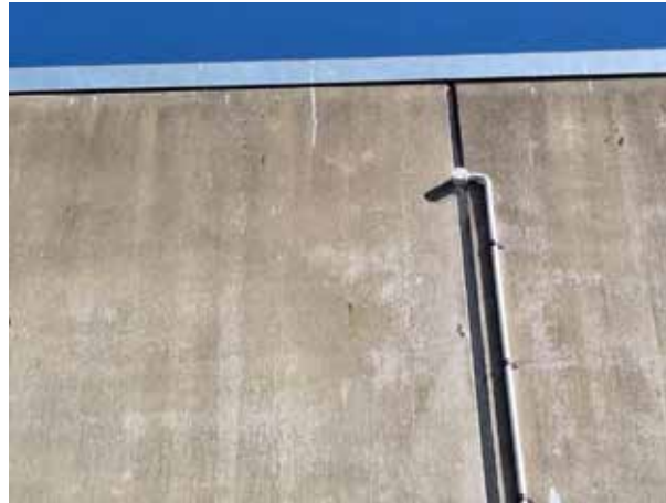
23. Sporadic areas of corrosion staining to the concrete wall panels. The corrosion staining appears to be leaching from the reinforcement bars of the concrete wall panels.
