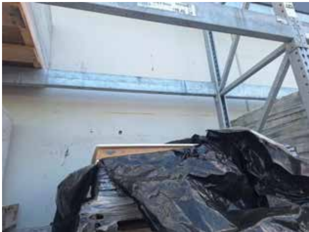
88. Widespread deterioration of the finish to the lower half of the concrete wall panels.
