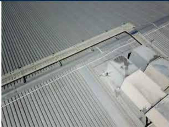
88. Corrosion to the kerb penetrations and sealant applied to the fit-over flashings and the ridge cappings.
