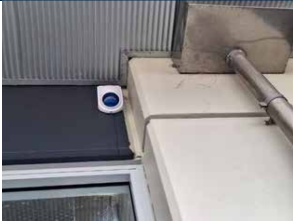
1. Localised moisture run-mark to the concrete wall panel as a result of a leak from the security alarm.
