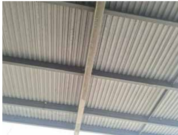
161. Sporadic areas of discolouration and corrosion to the steel canopy frame.
