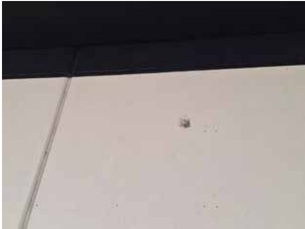
85. Sporadic areas of abrasions, deterioration and spalling to the concrete wall panels.
