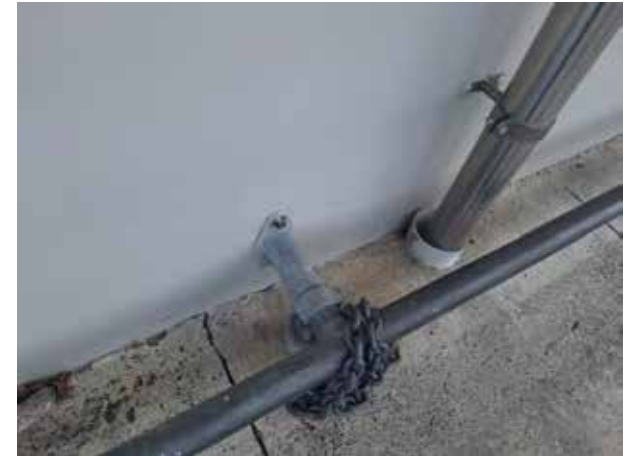
75. Sporadic areas of corrosion to the fixings of the metal bumper rails.
