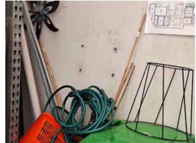
129. Localised fixings to the concrete wall panel at the western elevation.
