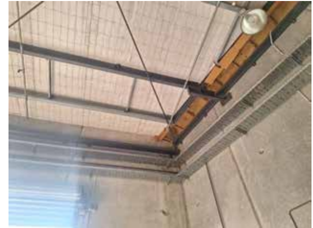
93. Localised moisture run-marks staining to the concrete wall panels and corrosion to the steel beam. This is emitting from the steel beam or internal gutters.
