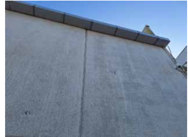
45. Sporadic areas of debonding of the sealant to the control joints of the concrete wall panels.
