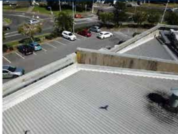
14. Staining on the metal capping and the internal face of the concrete wall.
