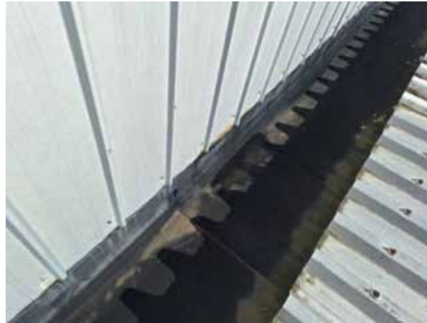
74. Widespread staining and dirt build-up to the internal gutters.
