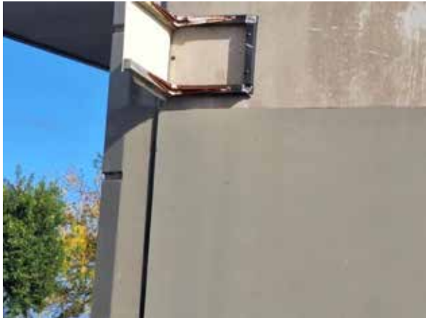
70. Widespread corrosion to the steel frame of the signage to the concrete wall panels.
