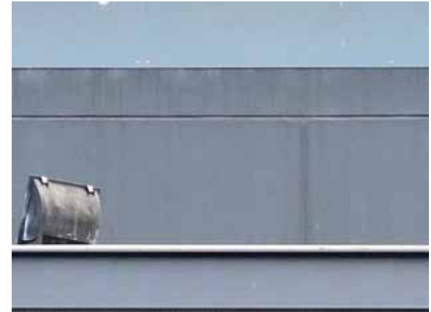
54. Sporadic areas of discolouration to the upper-level horizontal concrete wall panels and emitting from the joint.
