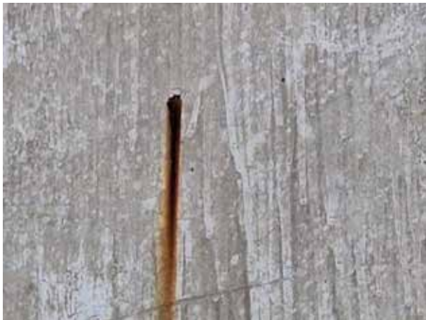
34. Sporadic areas of corrosion staining to the concrete wall panels. The corrosion staining appears to be leaching from the reinforcement bars of the concrete wall panels.
