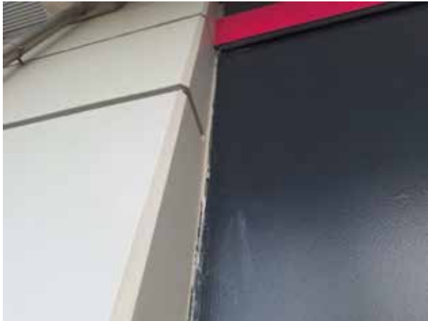
19. Localised separation to the concrete wall panels and the fibre-cement sheets.
