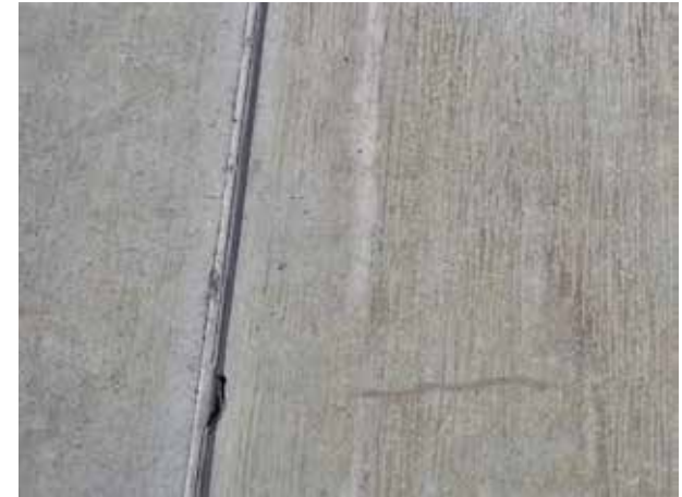
27. Sporadic areas of debonding and cracking to the sealant at the control joints of the concrete wall panels.
