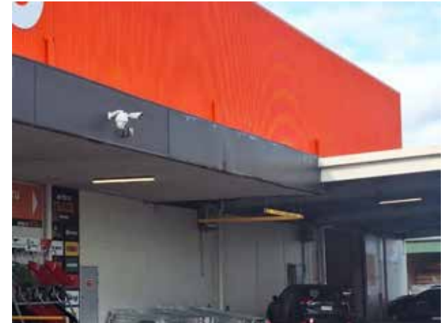
153. Sporadic areas of impact damage and distortion to the metal fascia canopy sheets.
