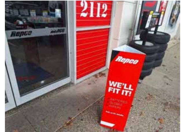
51. Sporadic areas of environmental staining to the aluminium shop front units.
