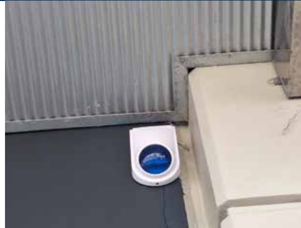
2. Localised moisture run-mark to the concrete wall panel as a result of a leak from the security alarm.
