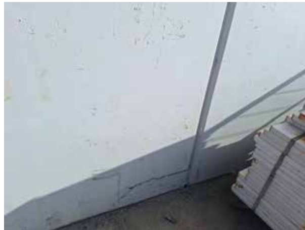
119. Sporadic areas of horizontal surface cracking to the base of the concrete wall panels at the northern elevation.
