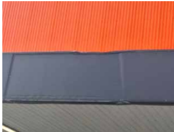
149. Sporadic areas of impact damage and distortion to the metal fascia canopy sheets.
