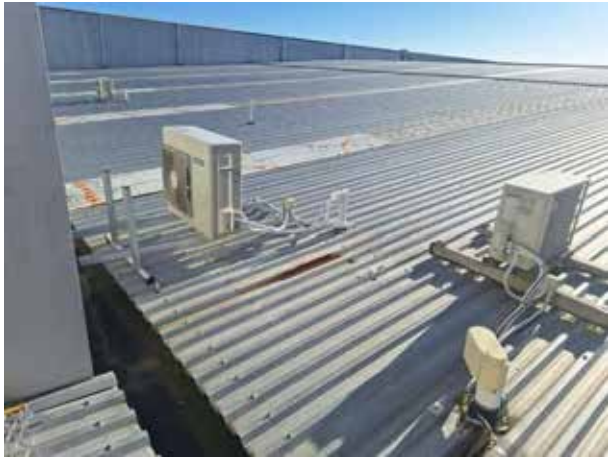
7. Localised corrosion to the profiled metal roof sheets.
