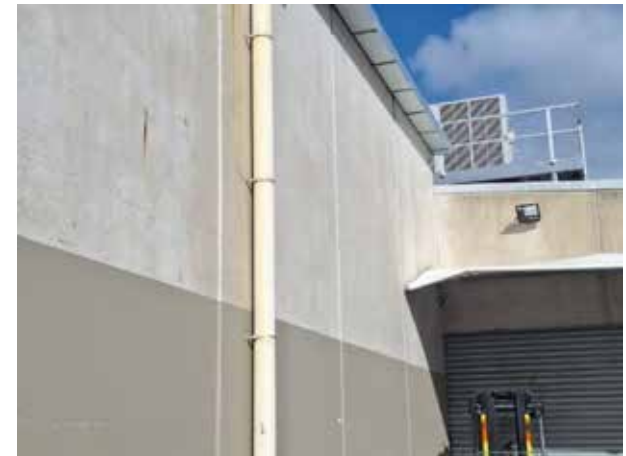
48. Widespread discoloration and staining to the concrete wall panels.
