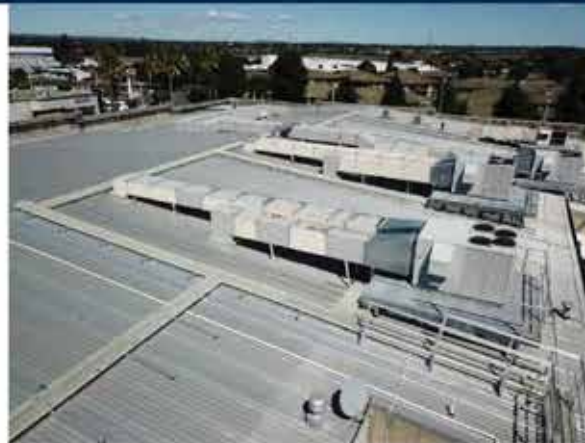
83. Corrosion and staining to the HVAC ducting.
