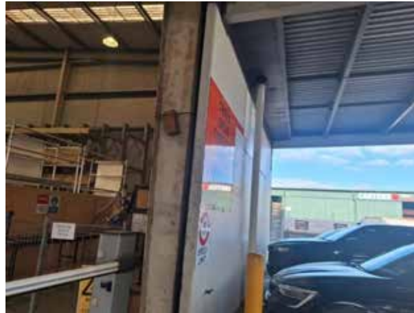
86. Sporadic areas of abrasions, deterioration and spalling to the concrete wall panels.
