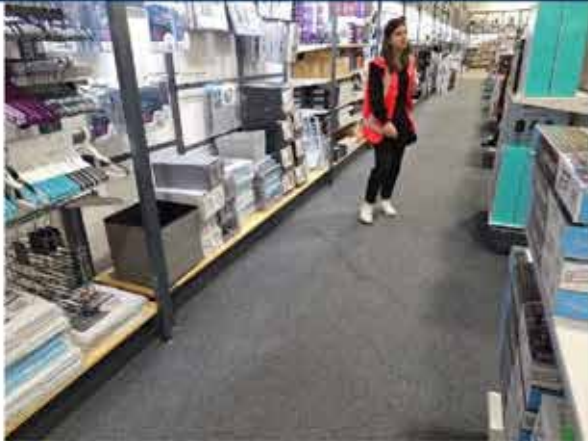
121. Minor staining on the carpet finish.
