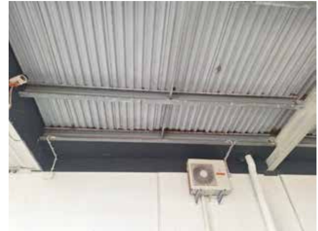
159. Widespread corrosion to the underside of the profiled metal canopy sheets.
