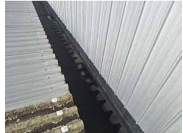
72. Widespread staining and dirt build-up to the internal gutters.
