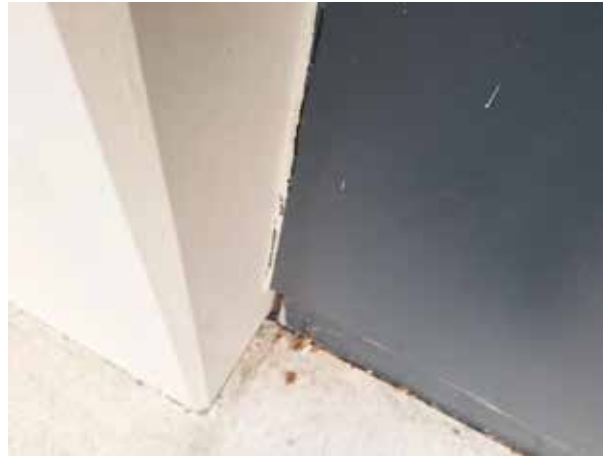
20. Localised separation to the concrete wall panels and the fibre-cement sheets.
