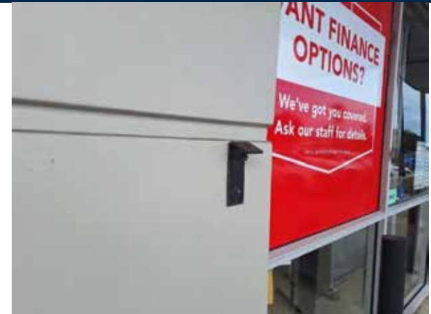
3. Localised corrosion of the fixings to the metal attachment trim of the concrete wall panels.
