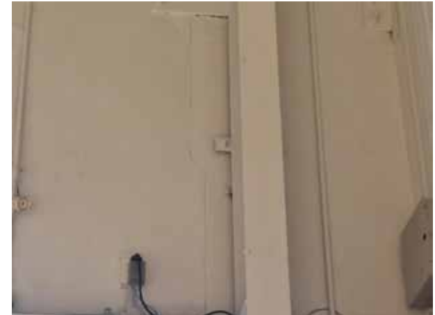
102. Localised vertical hairline cracking to the upper-level horizontal concrete wall panel.
