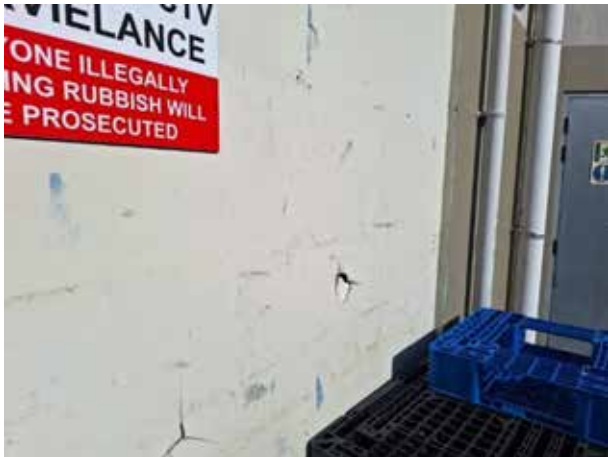
34. Localised area of extensive damage to the fibre-cement cladding sheets.
