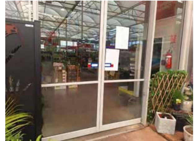
144. Sporadic areas of environmental staining to the aluminium shop front units.
