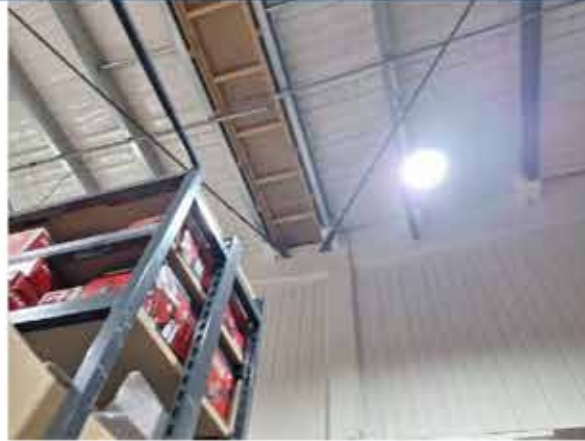
62. Localised staining to the plywood substrate (RepcO).
