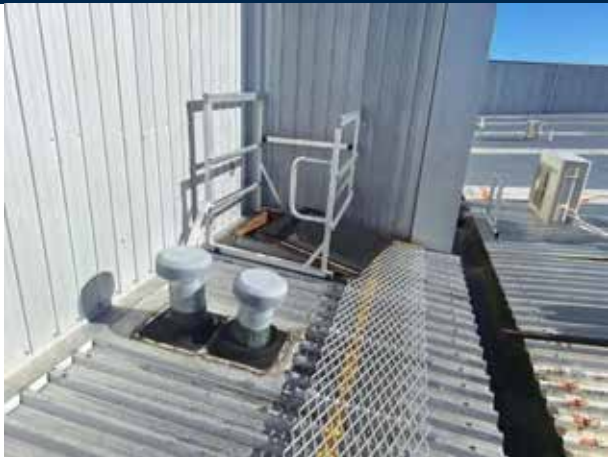
1. Localised partial detachment to the roof hatch.
