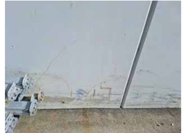
111. Sporadic areas of diagonal surface cracking to the base of the concrete wall panels at the northern elevation.
