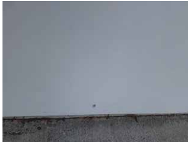
11. Sporadic areas of popping or recessed fixings to the fibre-cement cladding sheets.
