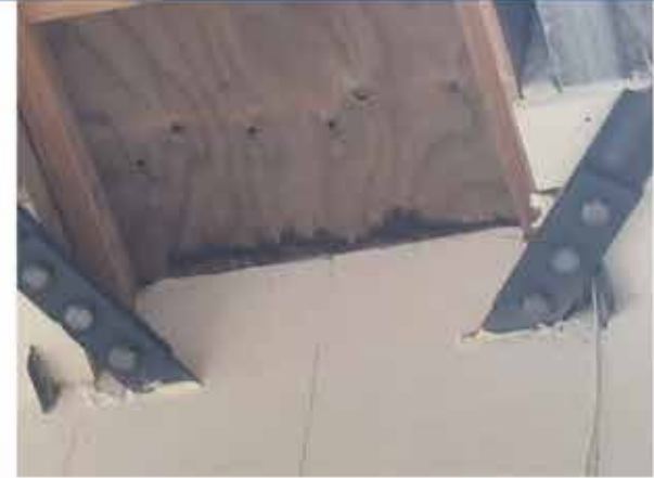
63. Localised staining to the plywood substrate (RepcO).
