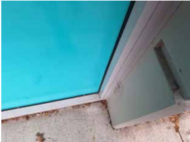
49. Sporadic areas of environmental staining to the aluminium shop front units.
