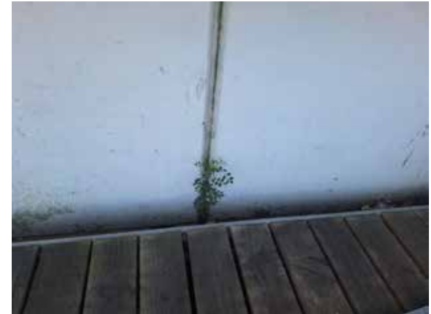
93. Sporadic areas of lichen and vegetation growth to the concrete wall panels at the eastern elevation. The Tenant's racking was installed at this location.
