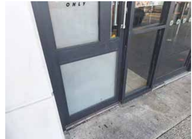
54. Sporadic areas of scuff marks and discoloration to the aluminium shop front units.
