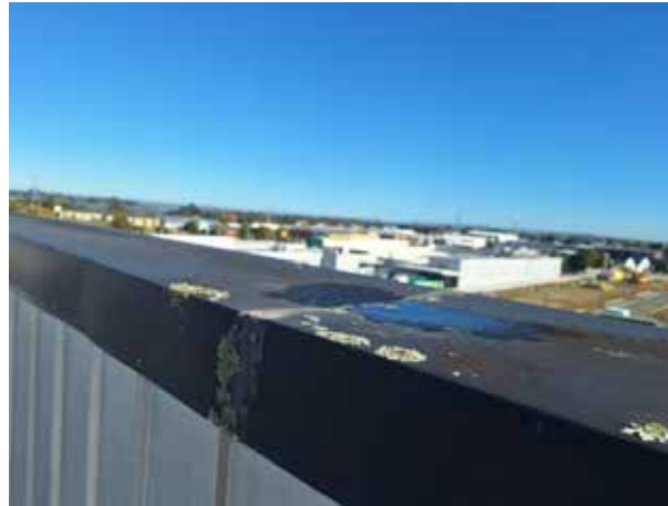
56. Sporadic areas of distortion and discolouration to the metal cappings to the parapet walls.
