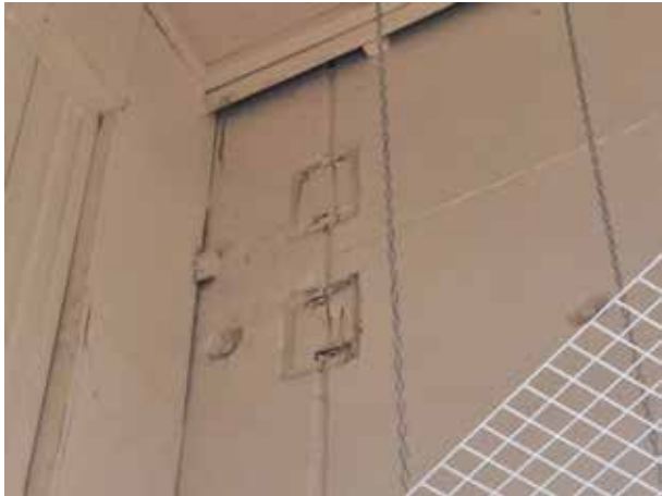
97. Widespread corrosion to the steel embedded plates of the concrete wall panels.
