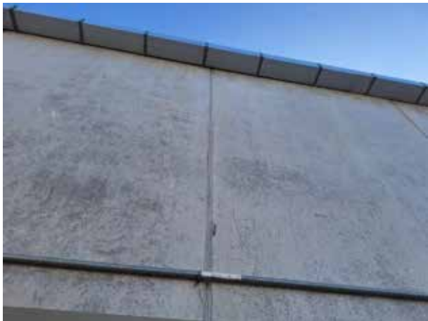
40. Widespread staining and discolouration to the concrete wall panels.
