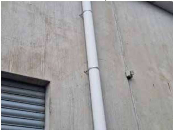
40. Widespread discolouration and staining to the concrete wall panels.
