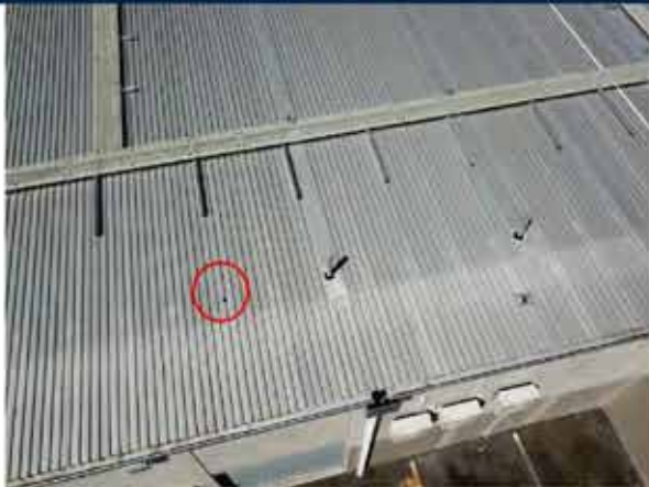
82. Previous repairs which appear to be carried out with sealant to the roof sheets.
