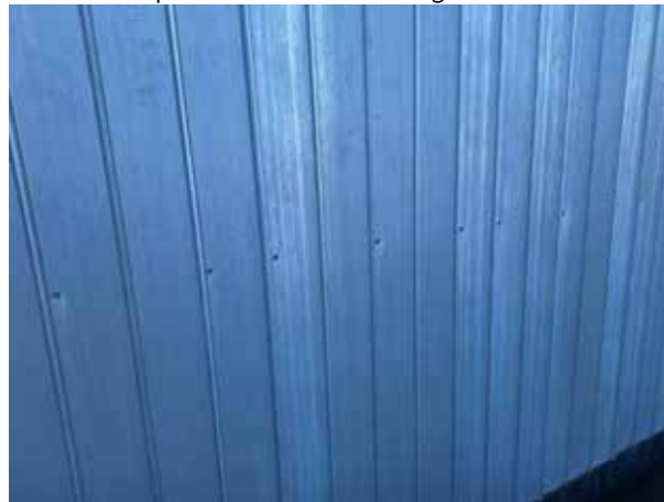
29. Sporadic areas of discolouration to the profiled metal internal parapet sheets.
