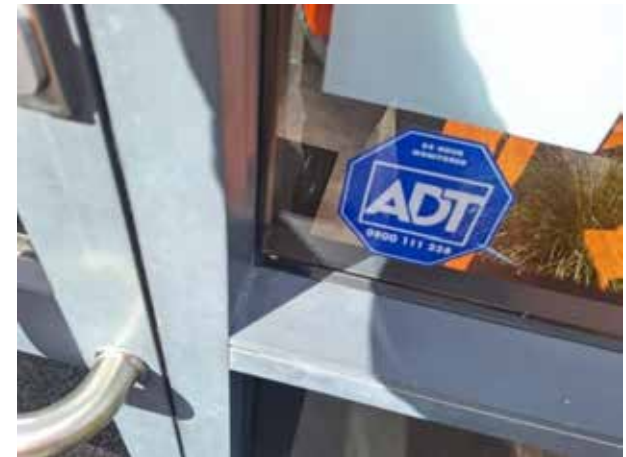
18. Sporadic areas of minor shrinkage to the glazing seals of the aluminium shop front units.
