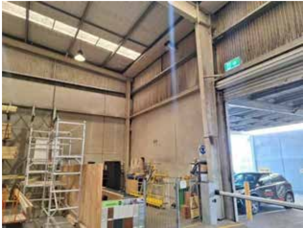
196. Widespread soil staining to the internal side of the elevations.
