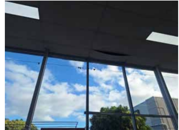
189. Localised bowing to the ceiling grid tiles below the entrance canopy.
