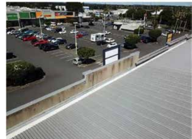
93. Extensive staining on the internal face of the concrete wall panels.
