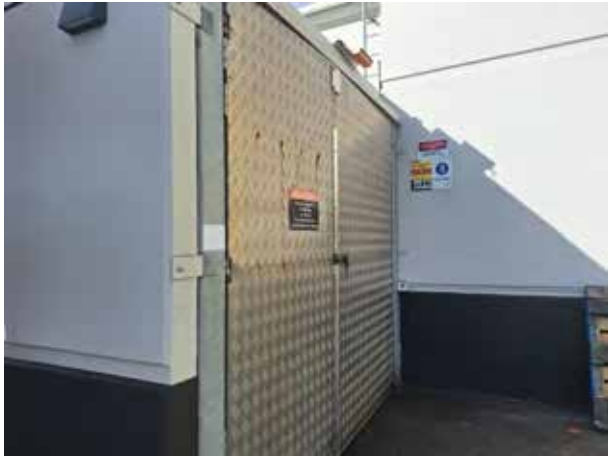
7. Sporadic areas of minor scuff marks and deterioration of the finish to the concrete wall panels.
