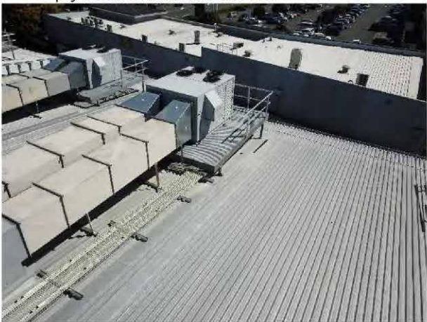
97. Extensive sealant applied to the fit-over flashings and adjacent profile metal roof sheets.
