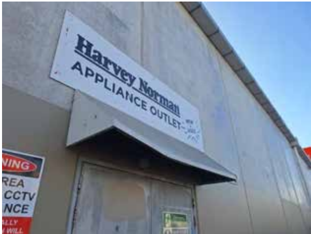
73. Sporadic areas of distortion to the metal door awnings.
