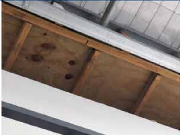
115. Minor discolouration to the timber box frame of the plywood substrate.
