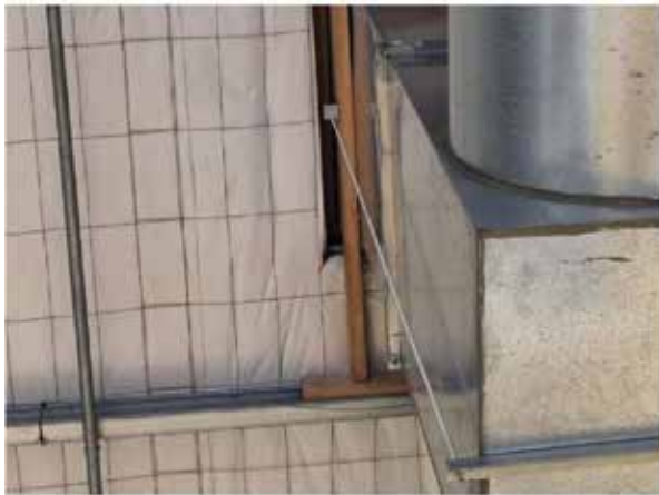
46. Minor wrinkling of the roof underlay adjacent to a large penetration (Bed Bath and Beyond).
