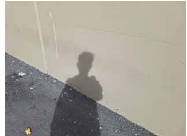
45. Sporadic areas of deterioration and spalling to the concrete wall panels.
