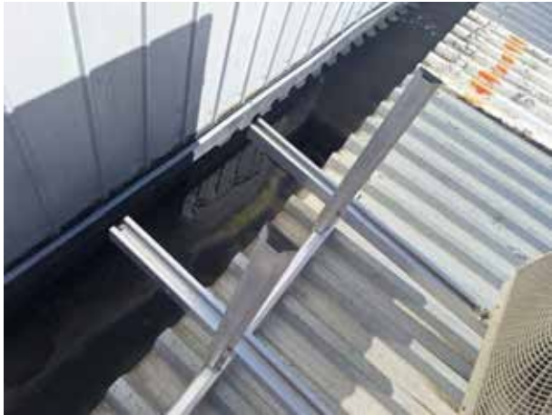
67. Localised ponding surface moisture to the internal gutters.
