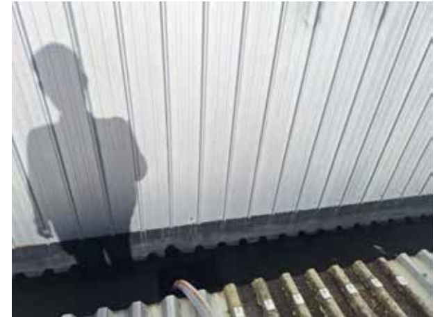
39. Localised extensive corrosion to the profiled metal internal parapet sheets adjacent to a fixing centre.
