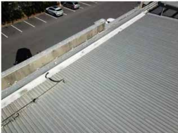
10. Staining on the single-plywood membranes at the internal gutters.
