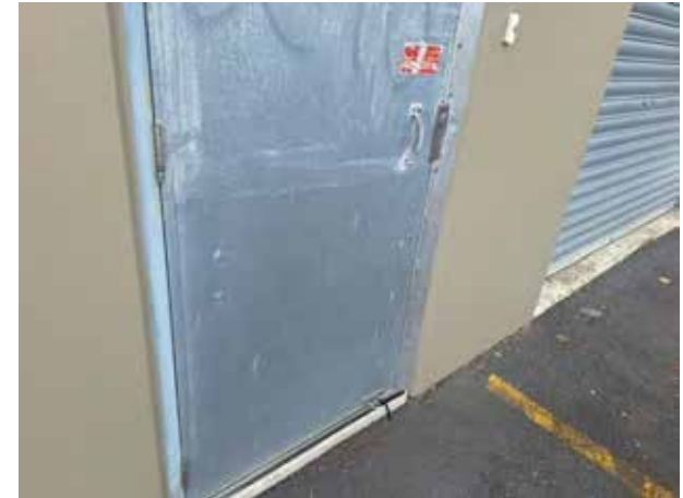
63. Sporadic areas of corrosion and discoloration to the galvanised steel hinged doors.
