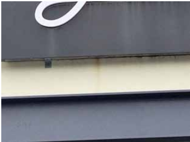
16. Localised corrosion run-off staining to the upper-level horizontal concrete wall panels emitting from the store signage .
