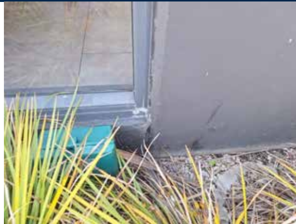
2. Sporadic areas of minor deterioration and spalling to the external face of the concrete base.
