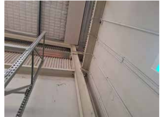
177. Sporadic areas of unsealed fixing or penetration centres to the profiled metal cladding sheets.
