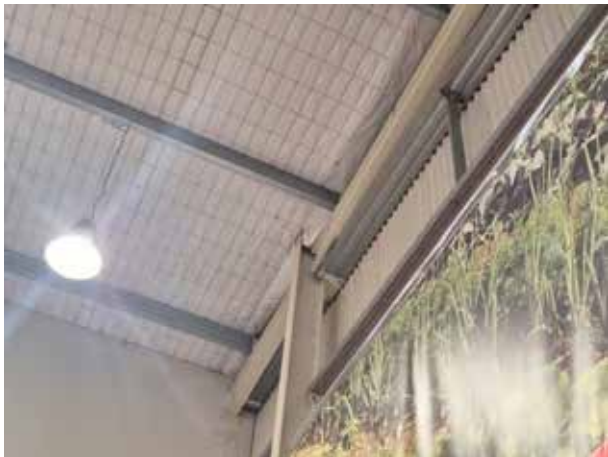
172. Sporadic areas of wrinkling to the building paper underlay.
