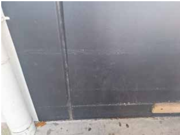
82. Widespread deterioration of the finish to the lower half of the concrete wall panels.
