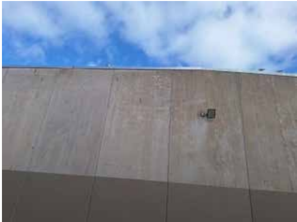
31. Widespread discoloration and staining to the concrete wall panels.
