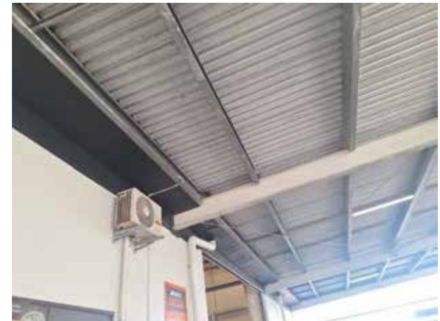
162. Widespread corrosion to the underside of the profiled metal canopy sheets.
