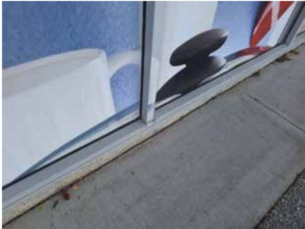
73. Localised scuff marks and abrasions to the aluminium shop front units.
