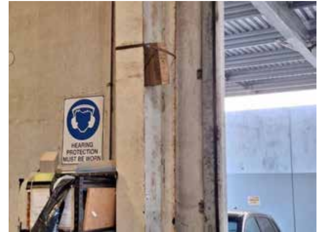
198. Localised area of corrosion to the painted steel column adjacent to an opening.
