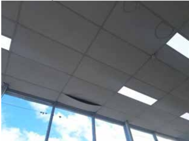
190. Sporadic areas of moisture staining to the ceiling grid tiles below the entrance canopy.
