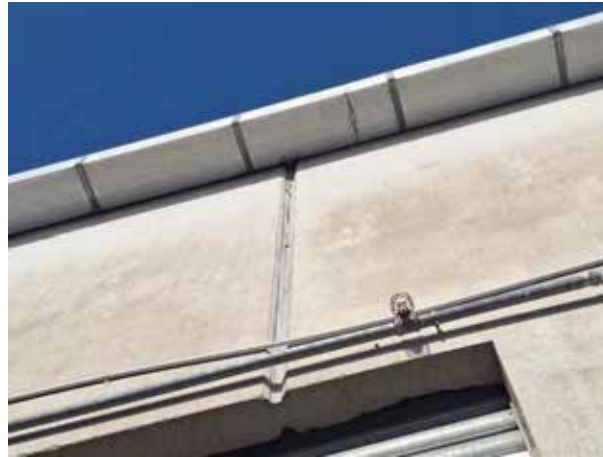
32. Sporadic areas of debonding of the sealant to the control joints of the concrete wall panels.
