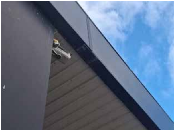
151. Sporadic areas of deterioration of the finish to the metal fascia sheets.
