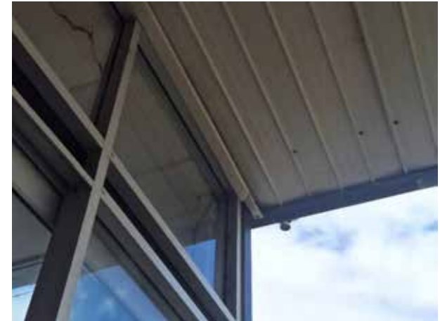
147. Localised distortion of the metal trim to the underside of the canopy.
