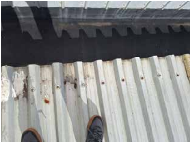
61. Widespread corrosion to the fixings of the profiled metal roof sheets.
