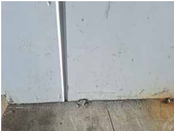
118. Sporadic areas of horizontal surface cracking to the base of the concrete wall panels at the northern elevation.
