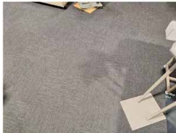
125. Staining on the carpet.
