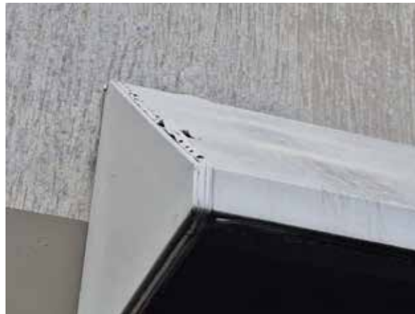
77. Sporadic areas of distortion to the metal door awning.
