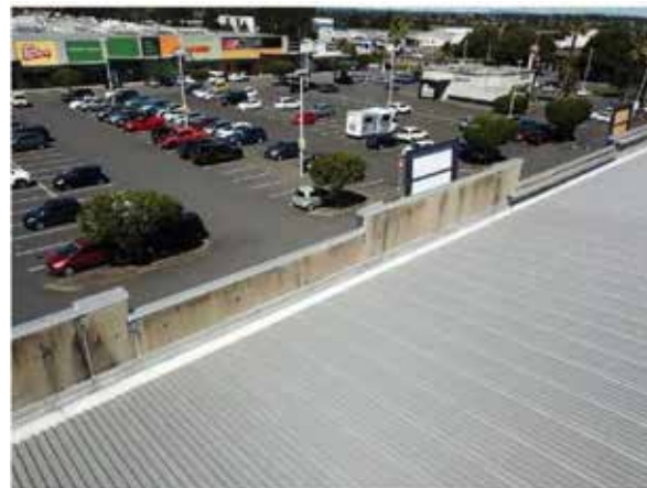
92. Corrosion on the metal anchor plates and extensive staining on the internal face of the concrete wall panels.
