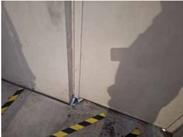
175. Sporadic areas of separation between the concrete floor slabs and concrete wall panels at the metal panelled hinged doors.
