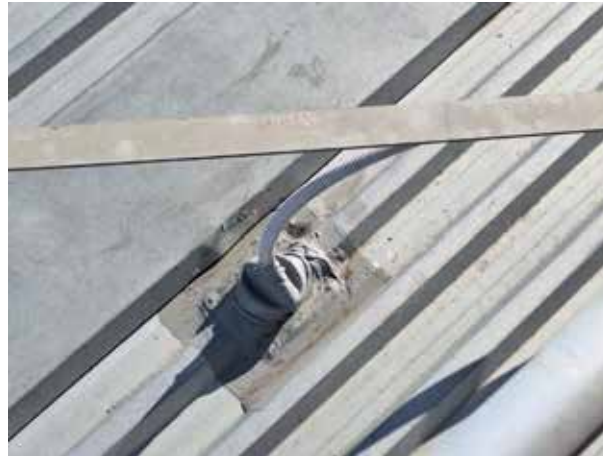
14. The spiral conduit pipe was well sealed.
