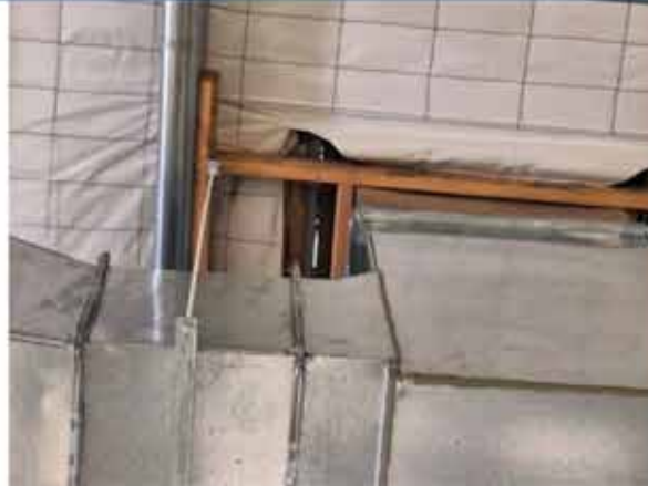
50. Minor separation to the vent housing. (The Baby Factory).
