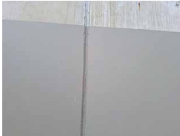
38. Sporadic areas of debonding and cracking to the sealant at the control joints of the concrete wall panels.
