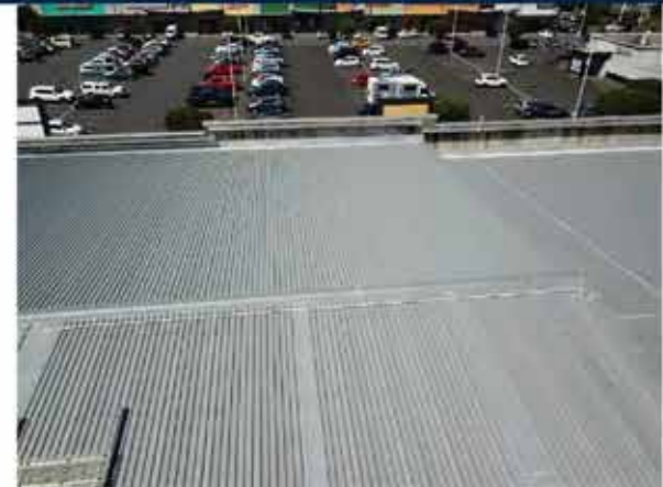
84. Extensive sealant applied to the ridge cappings and fit-over flashings.
