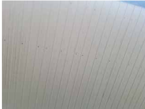
152. Widespread environmental staining to the underside profiled metal canopy sheets.
