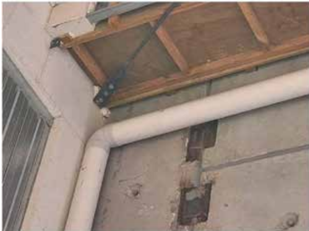
70. Minor staining on the concrete wall panels (Tool Shed).
