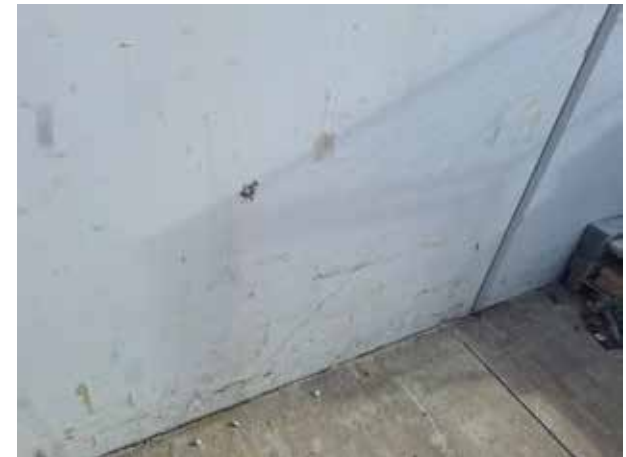
126. Sporadic areas of diagonal surface cracking to the base of the concrete wall panels at the northern elevation.
