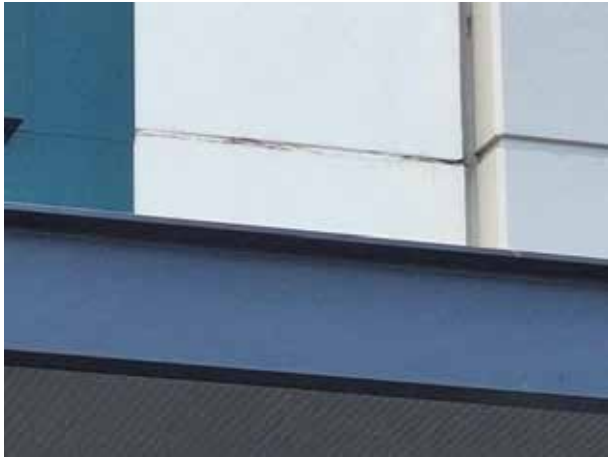
19. Sporadic areas of debonding and discoloration to the joint of the upper-level horizontal concrete wall panels.
