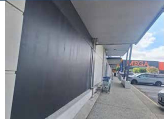
3. Sporadic areas of popping or recessed fixings to the fibre-cement cladding sheets.
