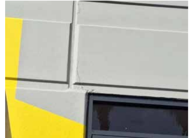
9. Localised minor surface cracking to the concrete wall panels emitting from the corner of the aluminium shop front units.
