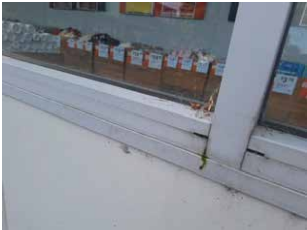
136. Localised mould staining to the aluminium shop front units.
