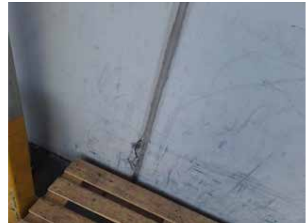
102. Sporadic areas of abrasions, deterioration and spalling to the concrete wall panels.
