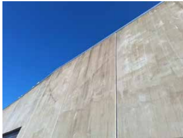
29. Localised area of diagonal surface cracking to the concrete wall panels.
