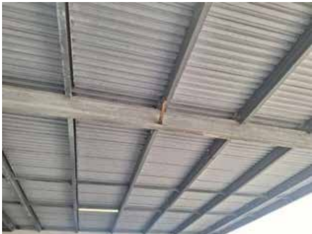
160. Sporadic areas of discolouration and corrosion to the steel canopy frame.
