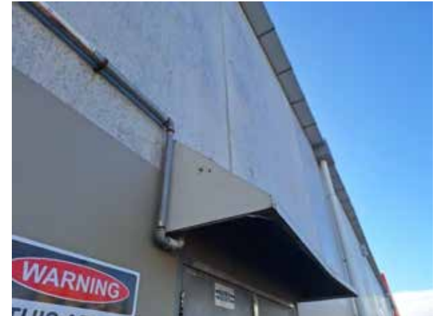
72. Sporadic areas of distortion to the metal door awnings.
