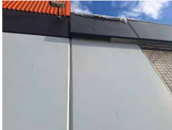
128. Widespread debonding of the sealant to the control joints of the concrete wall panels.
