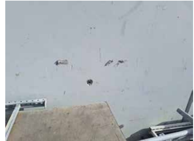
114. Sporadic areas of unsealed penetration centre to the concrete wall panels.
