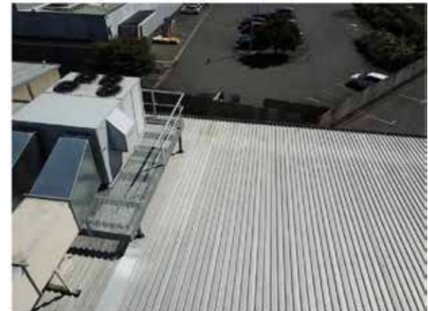
87. Environmental staining on the profiled metal roof sheets.
