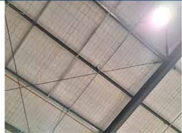
123. A localised tear was observed roof underlay adjacent which appears to be a post for the services platform. Fire sprinklers were also noted within the area.
