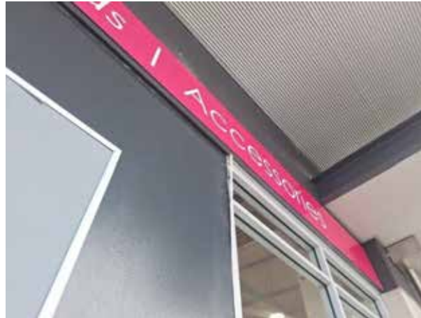
59. Localised partial detachment to the frame of the jamb of the aluminium shop front units.
