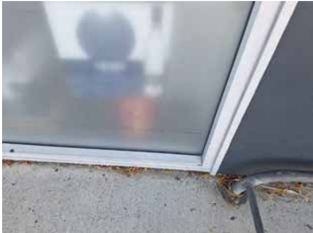
58. Localised deterioration of the glazing film to the aluminium shop front units.
