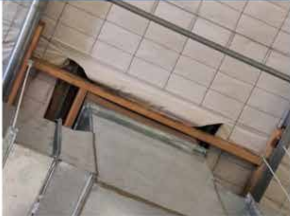
49. Minor wrinkling of the roof underlay adjacent to a large penetration (The Baby Factory).
