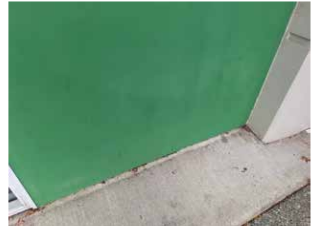
6. Sporadic areas of deterioration of the paint finish to the elevations.
