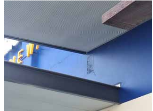
21. Localised residue staining to the upper-level horizontal concrete wall panels from a removed fixture.
