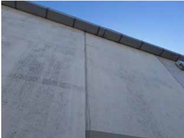
43. Widespread staining and discolouration to the concrete wall panels.
