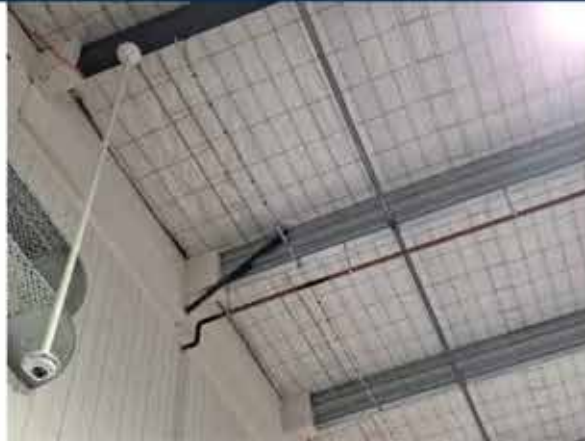
122. Staining observed below a copper pipe, sprinkler and the exposed roof structure. No obvious visual signs of water ingress were present to the roof structure.
