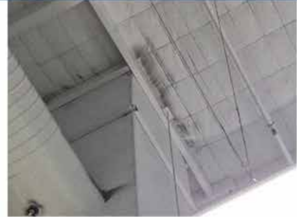
114. Environmental staining on the roof underlay.
