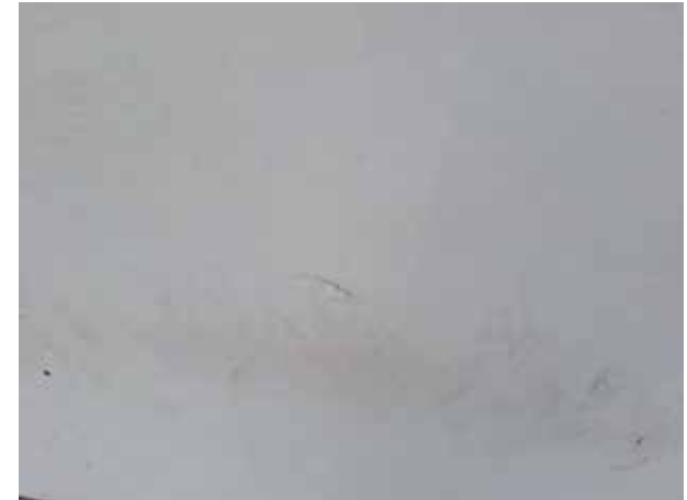
15. Localised impact damage to the fibre-cement cladding sheets.
