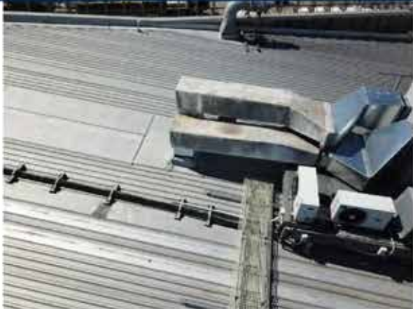
7. Extensive sealant applied to the fit-over flashings and kerb penetrations.
