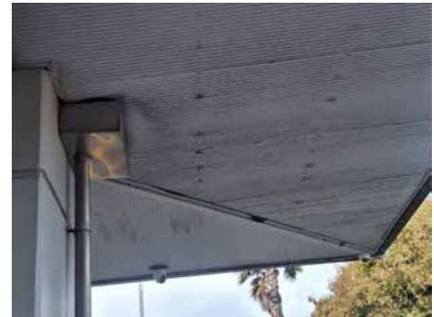
84. Localised corrosion to the underside of the canopy.
