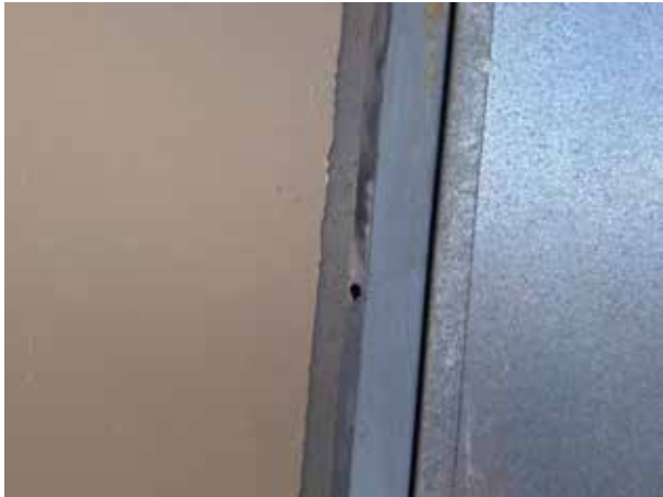
67. Localised debonding to the sealant to the perimeter of the galvanised steel hinged doors.
