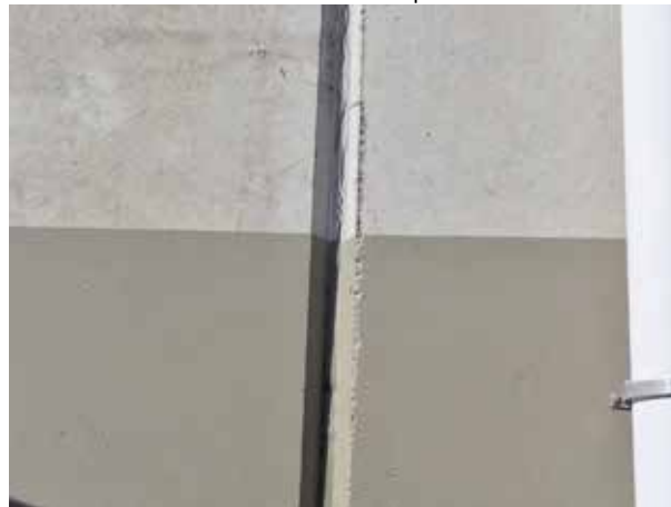
47. Sporadic areas of debonding and cracking to the sealant at the control joints of the concrete wall panels.
