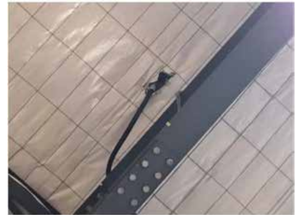
66. Minor tears to the roof underlay adjacent to a penetration (Harvey Norman).
