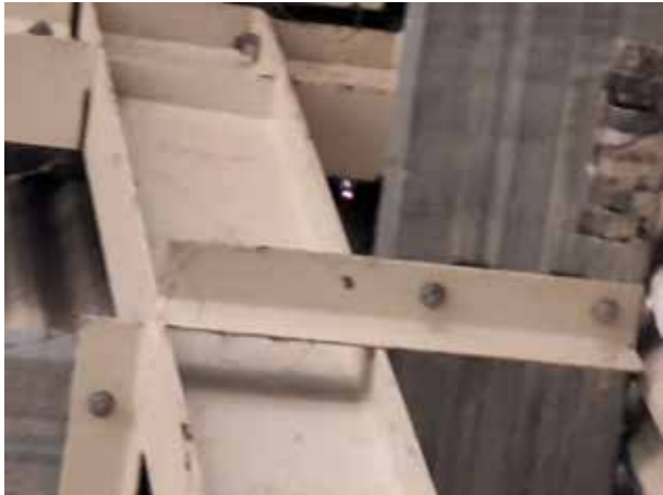
178. Sporadic areas of unsealed fixing or penetration centres to the profiled metal cladding sheets.
