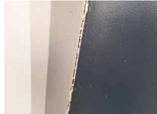
18. Localised separation to the concrete wall panels and the fibre-cement sheets.
