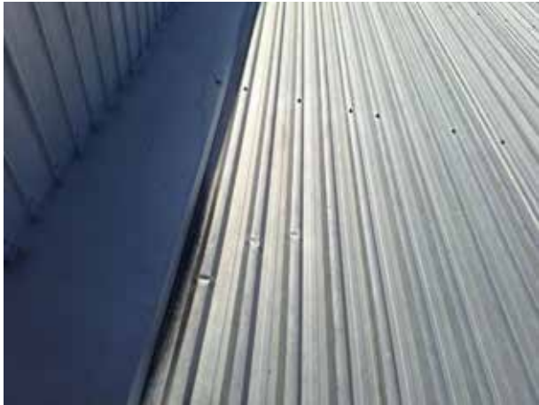
55. Sporadic areas of indentations to the profiled metal roof sheets.
