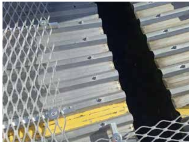
5. Widespread corrosion to the fixings of the profiled metal roof sheets.
