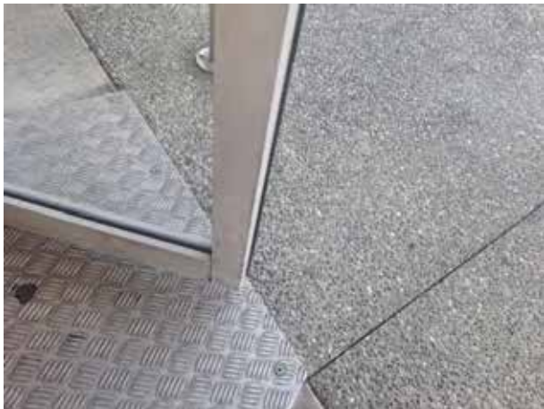
82. Sporadic areas of scuff marks and abrasions to the aluminium shop front units.
