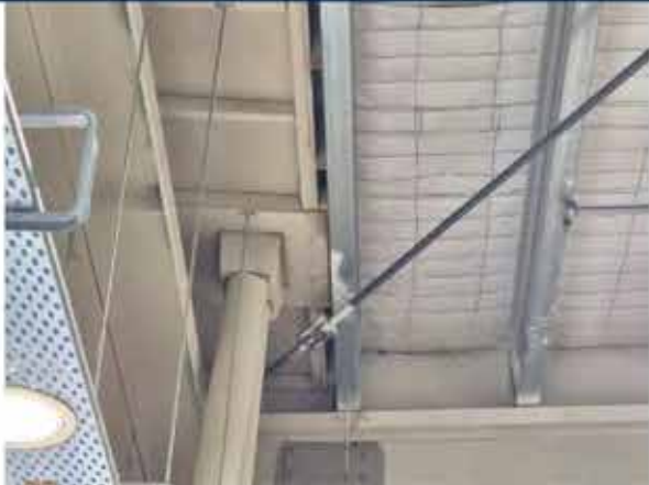
106. Staining on discolouration to the painted external cutters.
