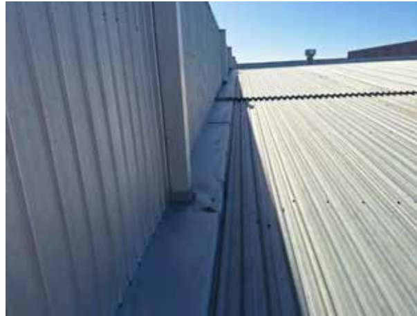
50. Sporadic areas of distortion to the apron flashings.
