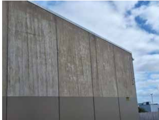
32. Widespread discoloration and staining to the concrete wall panels.
