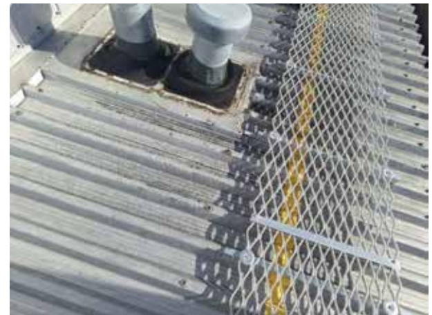
6. Widespread corrosion to the fixings of the profiled metal roof sheets.
