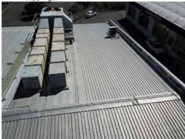
91. Extensive sealant applied to the ridge cappings and fit-over flashings.
