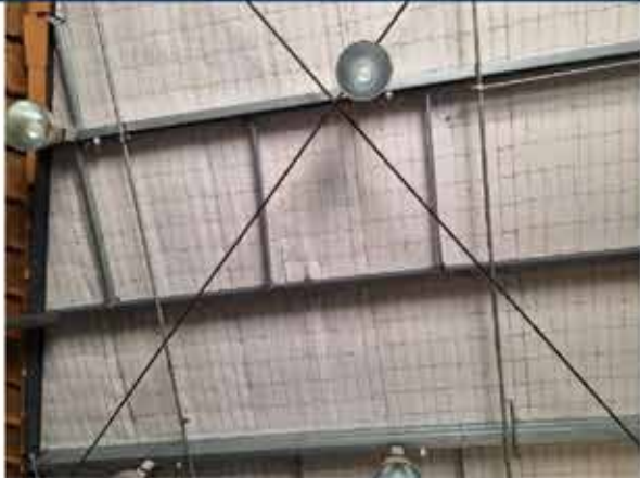
31. Minor discoloration and tears to the roof underlay (Fruit World).
