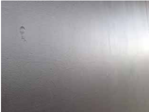
7. Localised former signage markings to the fibre-cement cladding sheets.
