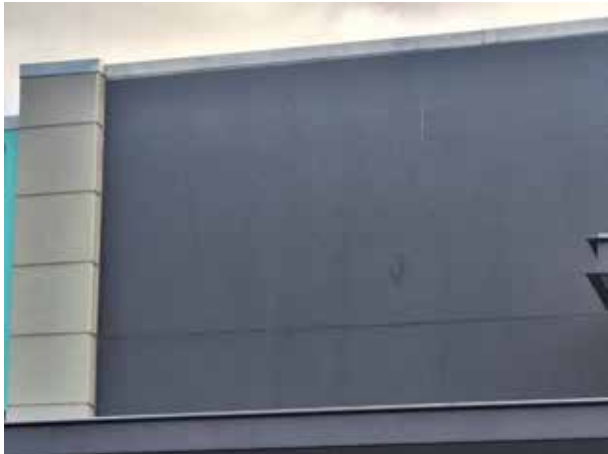
22. Localised blistering of the paint finish to the upper-level horizontal concrete wall panels.
