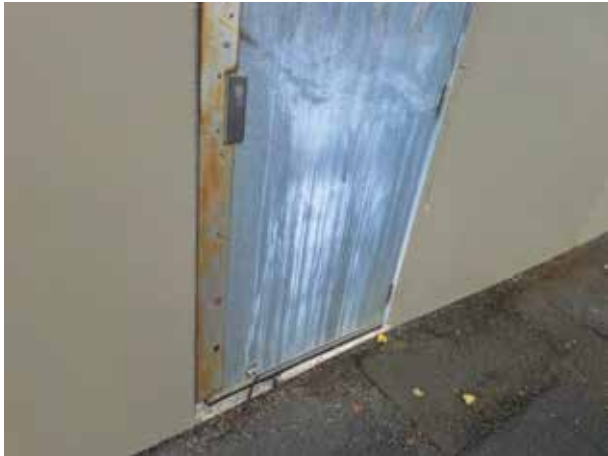
61. Sporadic areas of corrosion and discoloration to the galvanised steel hinged doors.
