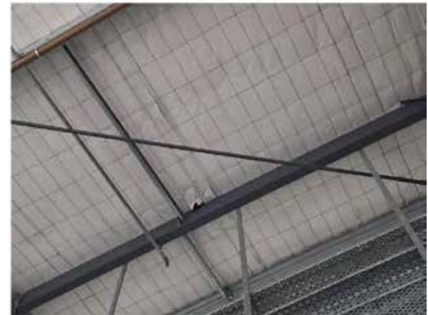
42. A localised tear to the roof underlay, adjacent to a external services platform post. (RepcO).
