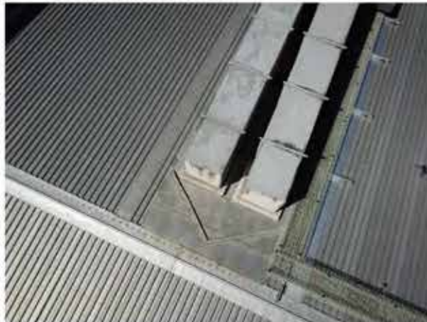
23. Deterioration of the finish and staining to the HVAC trunking.
