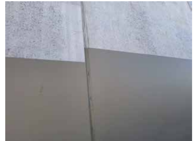
42. Sporadic areas of debonding of the sealant to the control joints of the concrete wall panels.
