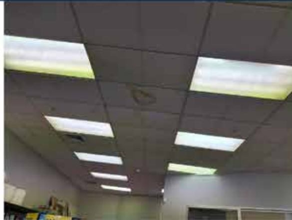
38. Moisture-related staining to the ceiling grid tiles (Western Union).
