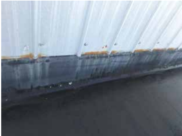
25. Sporadic areas of corrosion to the base of the profiled metal internal parapet sheets. The base of the sheets was in close proximity to the upstand of the internal gutter.
