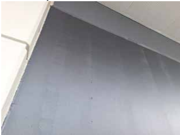
4. Sporadic areas of popping or recessed fixings to the fibre-cement cladding sheets.
