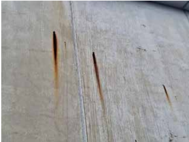
37. Sporadic areas of corrosion staining to the concrete wall panels. The corrosion staining appears to be leaching from the reinforcement bars of the concrete wall panels.
