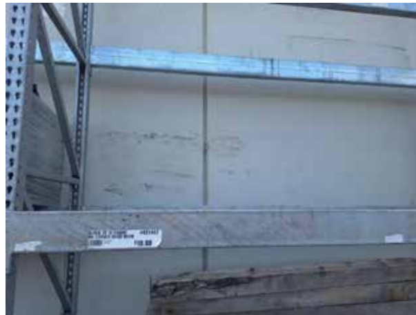
89. Widespread deterioration of the finish to the lower half of the concrete wall panels.
