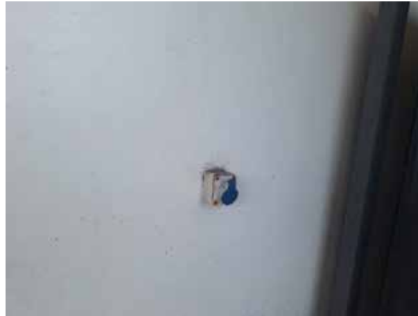
170. Widespread corrosion to the fixings of a wall-mounted power outlet.
