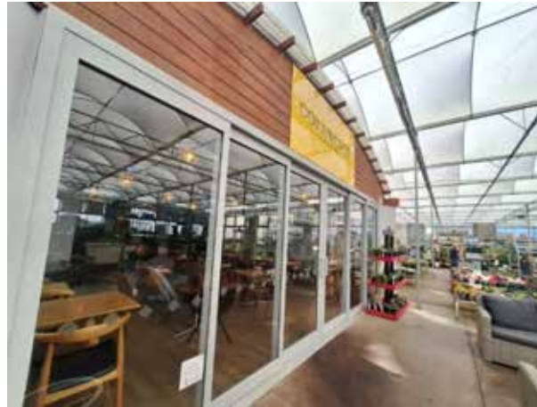
143. Sporadic areas of environmental staining to the aluminium shop front units.
