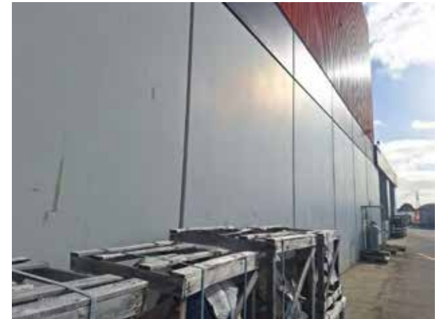
123. Widespread deterioration of the finish to the lower half of the concrete wall panels.
