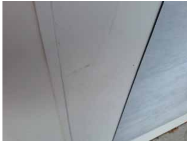
11. Sporadic areas of deterioration of the paint finish to the elevations.
