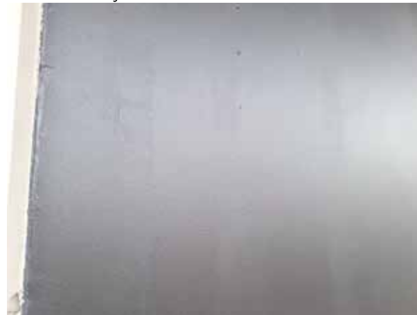
5. Sporadic areas of popping or recessed fixings to the fibre-cement cladding sheets.
