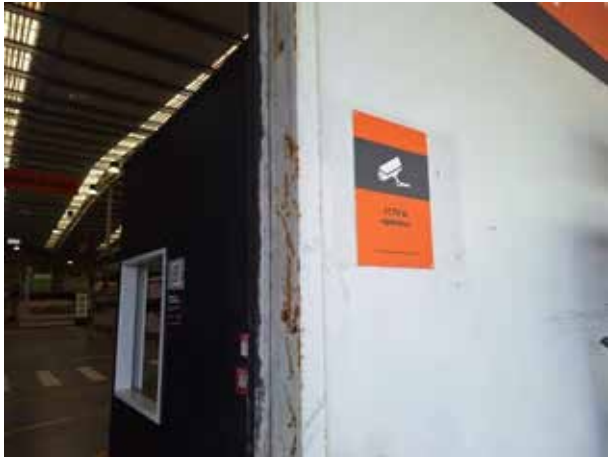
139. Widespread corrosion to the metal opening cappings.
