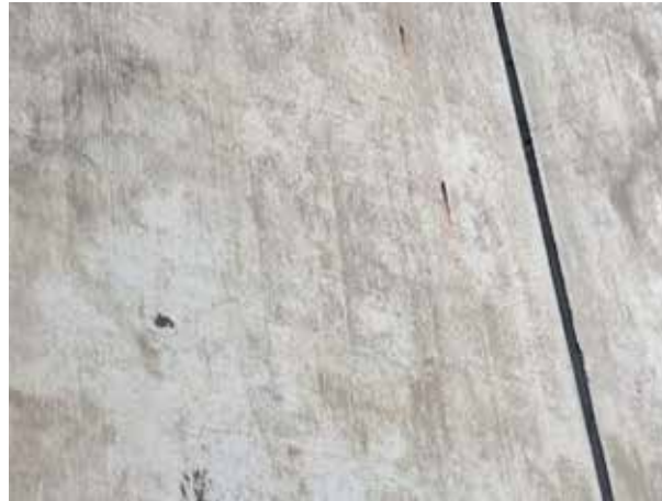
26. Sporadic areas of corrosion staining to the concrete wall panels. The corrosion staining appears to be leaching from the reinforcement bars of the concrete wall panels.
