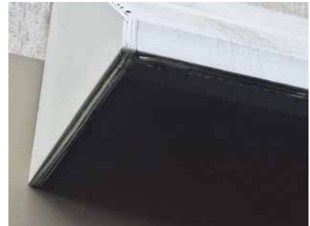
78. Sporadic areas of distortion to the metal door awning.
