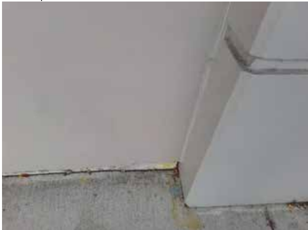
4. Sporadic areas of deterioration of the paint finish to the elevations.
