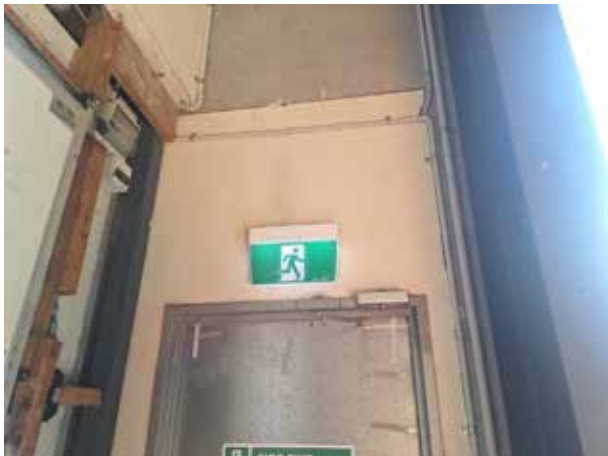
94. Localised removed door hardware with redundant fixing centres to the galvanised steel hinged door.
