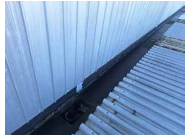
30. Sporadic areas of corrosion to the base of the profiled metal internal parapet sheets.
