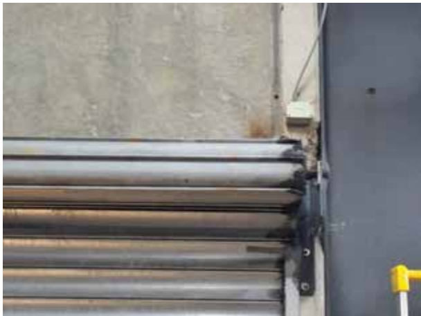
94. Widespread corrosion to the steel embedded plates of the concrete wall panels.
