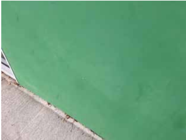
7. Sporadic areas of deterioration of the paint finish to the elevations.
