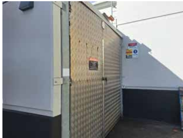
17. Sporadic areas of corrosion to the diamond checker plates of the hinged doors.
