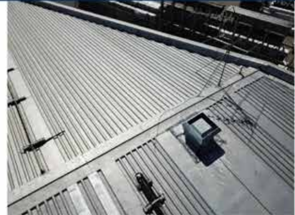
9. Extensive sealant applied to the fixings of the ridge cappings.
