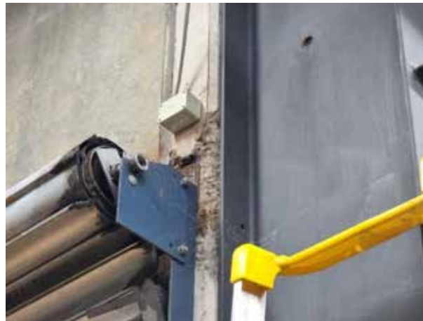
95. Localised corrosion and extensive abrasions to the concrete wall panel within a tenancy which is adjacent to a metal roller shutter door.
