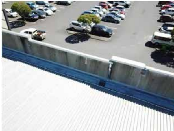
71. Deterioration of the sealant at the control joints of the concrete parapet walls. Flashing tape and extensive sealant applied to the metal capping and concrete parapet walls.
