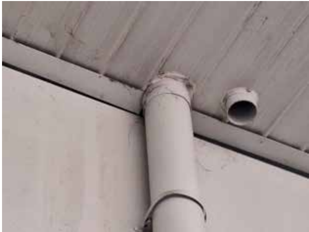
145. Localised debonding to the sealant applied between the underside of the canopy and the downpipe.
