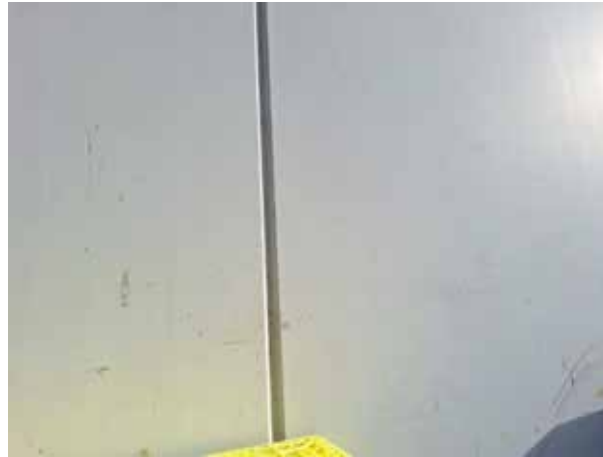
104. Widespread debonding of the sealant to the control joints of the concrete wall panels.
