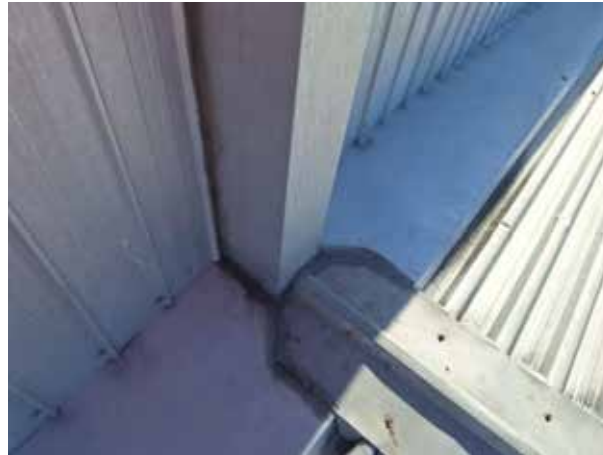
53. Widespread sealant applied to the joints of the apron flashings to metal ridge cappings.
