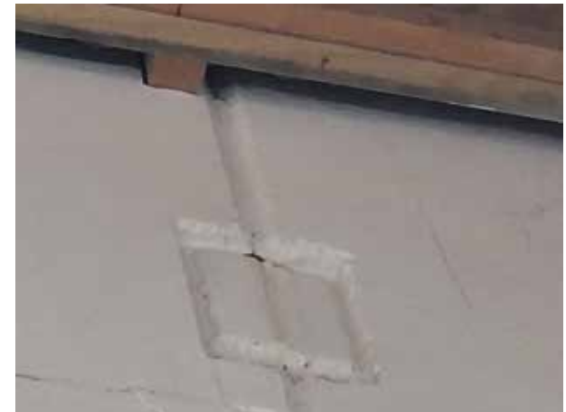
96. Widespread corrosion to the steel embedded plates of the concrete wall panels.
