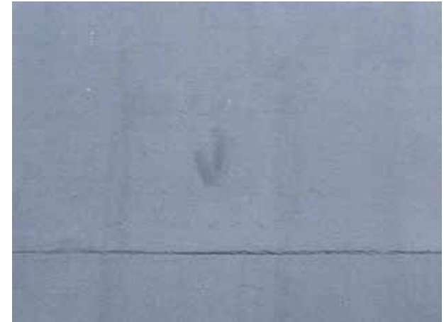
24. Localised blistering of the paint finish to the upper-level horizontal concrete wall panels.
