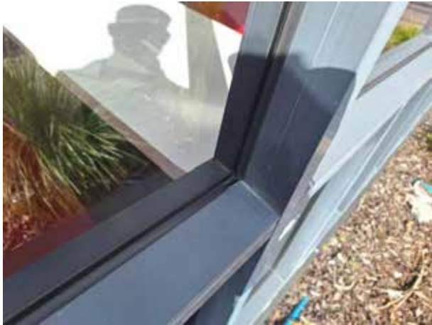
19. Sporadic areas of minor shrinkage to the glazing seals of the aluminium shop front units.
