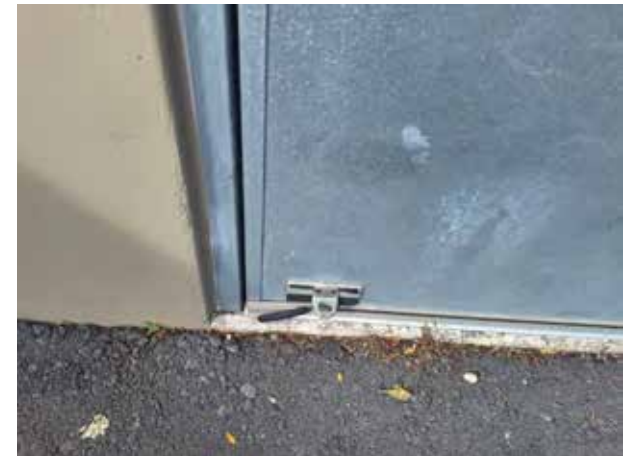
66. Sporadic areas of corrosion and discoloration to the galvanised steel hinged doors.
