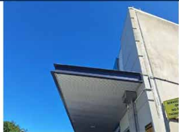
75. Minor deterioration of the finish to the steel perimeter frame.
