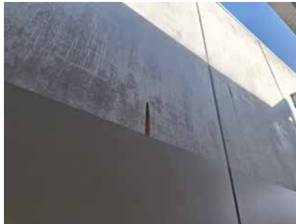
47. Sporadic areas of corrosion staining to the concrete wall panels. The corrosion staining appears to be leaching from the reinforcement bars of the concrete wall panels.
