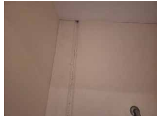
96. Sporadic areas of debonding to the sealed at the control joints of the concrete wall panels.
