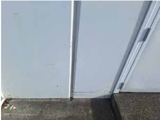
127. Sporadic areas of horizontal surface cracking to the base of the concrete wall panels at the northern elevation.
