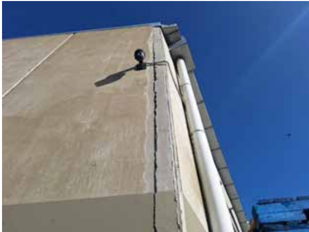
31. Localised vertical cracking to a joint to the concrete wall panels.
