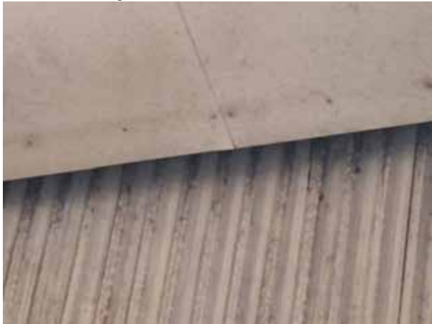
202. Widespread soil staining to the internal side of the elevations.
