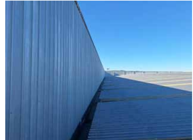
27. Sporadic areas of discolouration to the profiled metal internal parapet sheets.
