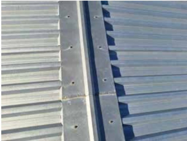
19. Widespread corrosion to the fixings of the metal ridge cappings.
