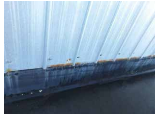
24. Sporadic areas of corrosion to the base of the profiled metal internal parapet sheets. The base of the sheets was in close proximity to the upstand of the internal gutter.
