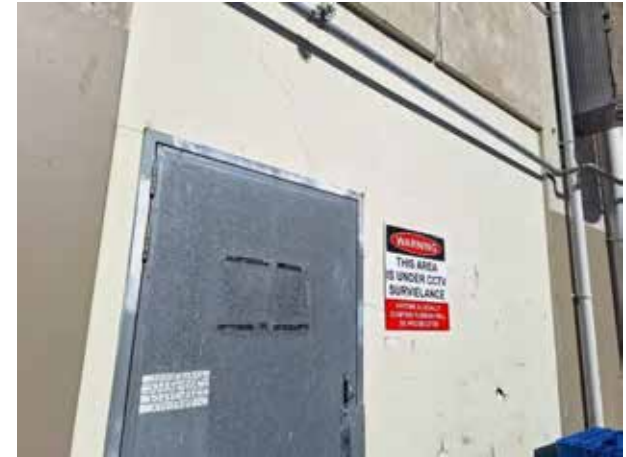
63. Sporadic areas of discolouration and corrosion to the galvanised steel hinged doors.
