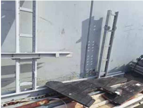
109. Widespread deterioration of the finish to the lower half of the concrete wall panels.
