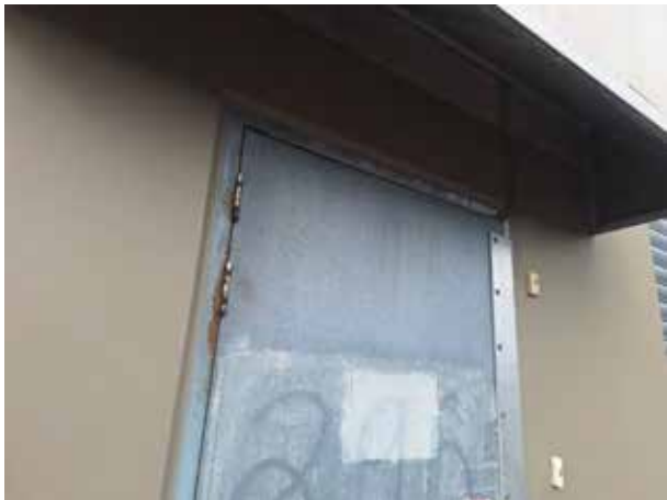
64. Sporadic areas of corrosion and discoloration to the galvanised steel hinged doors.
