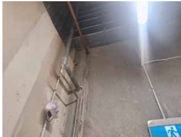
83. Localised moisture run-marks staining to the concrete wall panels emitting from the pipe penetration.
