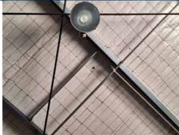
32. Minor discoloration and tears to the roof underlay (Fruit World).
