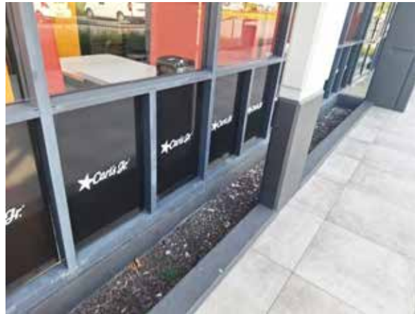
14. Widespread fading to the powder coated finish of the aluminium shop front units.
