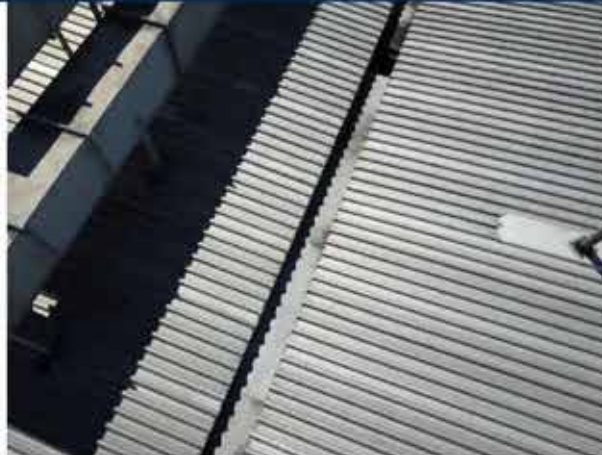
20. Staining and uplift at the sheet joints of the single-plywood membranes.
