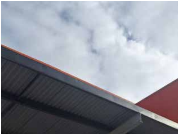
166. Sporadic areas of distortion to the metal barge cappings of the canopy.
