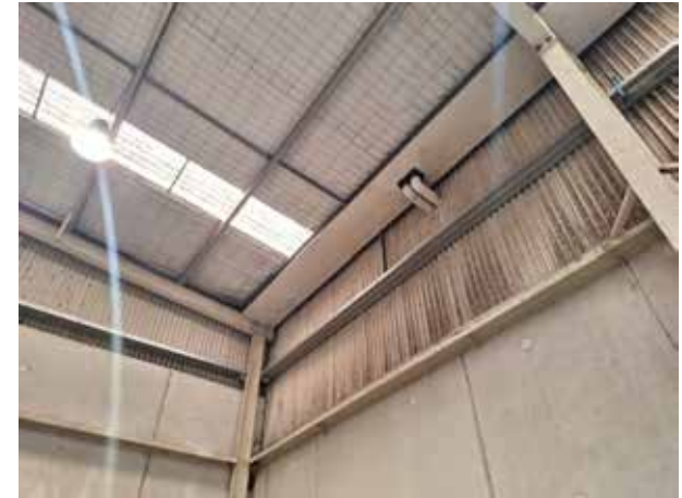
201. Widespread soil staining to the internal side of the elevations.
