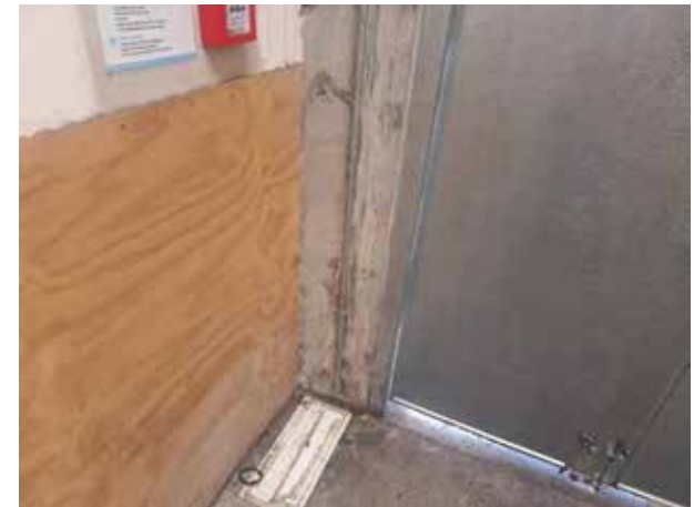
84. Localised moisture run-marks staining to the concrete wall panels emitting from the pipe penetration.
