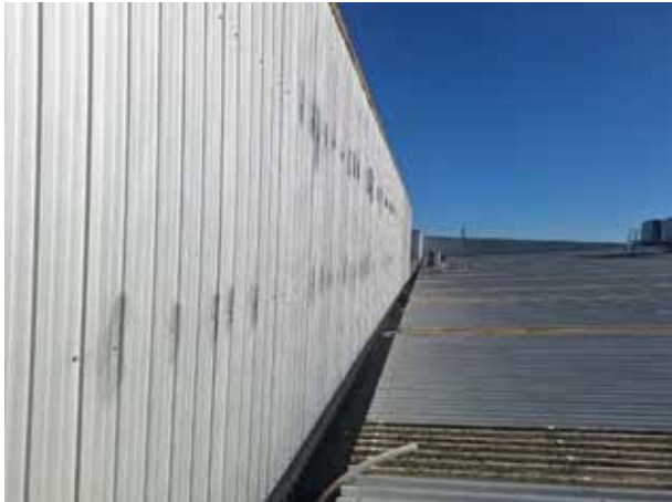
40. Localised area of discolouration to the profiled metal internal parapet sheets.
