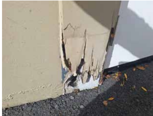
68. Localised swelling and damage to the timber liners at the western elevation.
