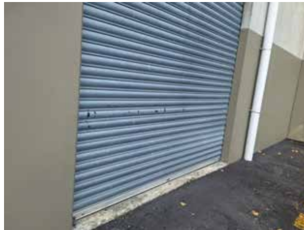
65. Sporadic areas of discoloration to the metal roller doors.
