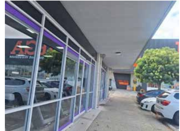
60. Sporadic areas of environmental staining to the aluminium shop front units.
