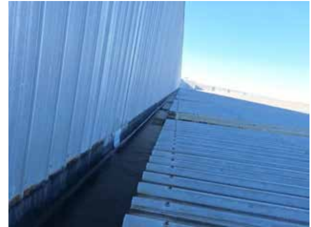
69. Widespread moisture run-marks and discoloration to the upstand of the synthetic rubber sheets.
