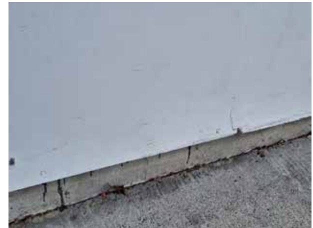
12. Sporadic areas of popping or recessed fixings to the fibre-cement cladding sheets.
