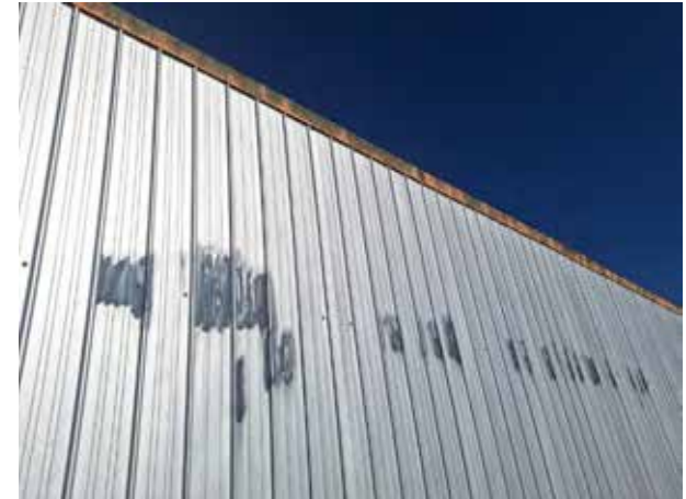
45. Localised area of discoloration to the profiled metal internal parapet sheets.
