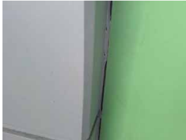
8. Localised separation and debonding of the sealant between the concrete wall panels.
