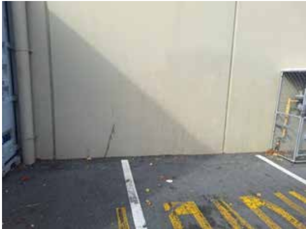
49. Localised surface corner cracking to the base of the concrete wall panels at the western elevation.
