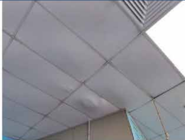
26. Moisture-related damage to the ceiling gird tiles (Takanini Fish Mart).
