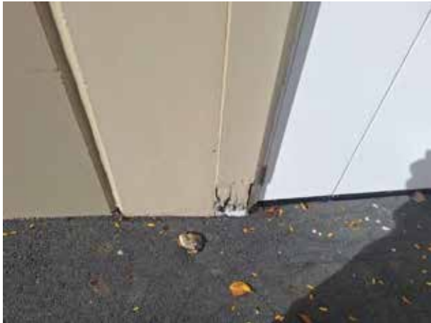
67. Localised swelling and damage to the timber liners at the western elevation.
