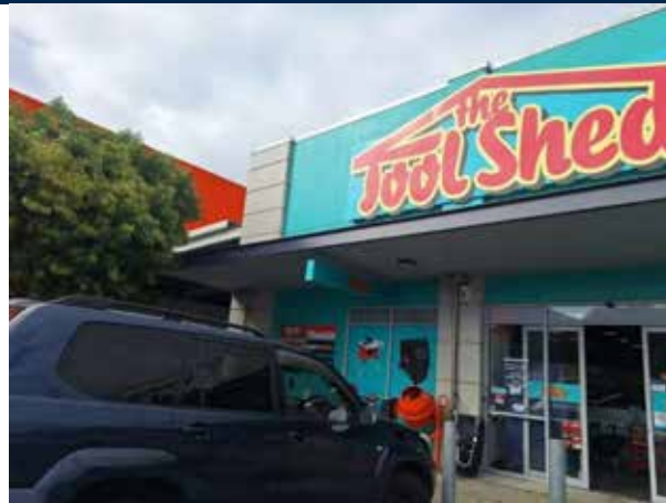
2. Sporadic areas of redundant fixing centres to the upper-level horizontal concrete wall panels.
