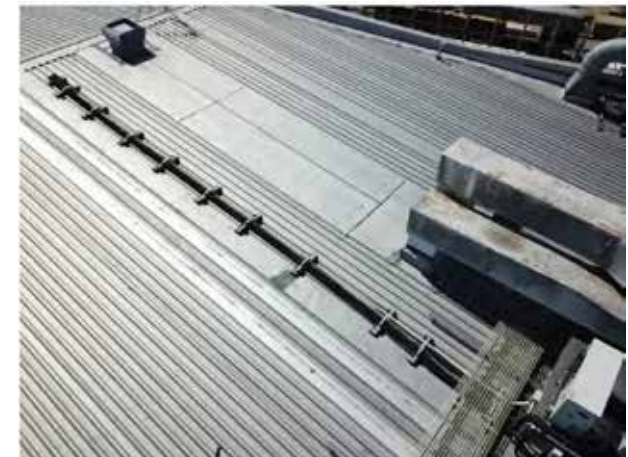
6. Extensive sealant applied to the fit-over flashings and kerb penetrations.
