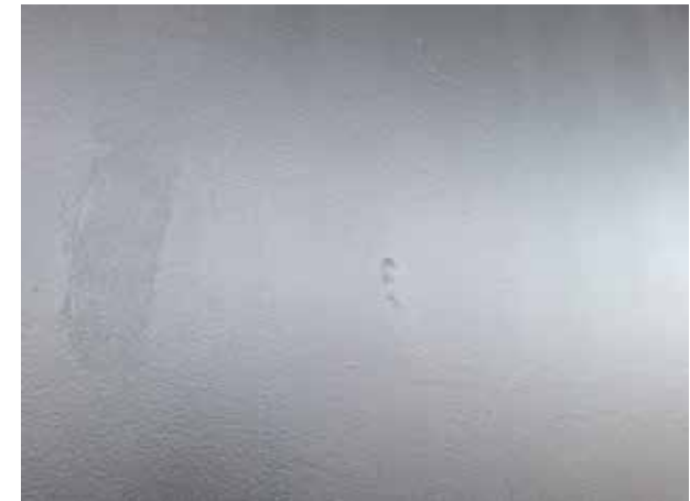
6. Localised blistering of the paint finish to the fibre-cement cladding sheets.
