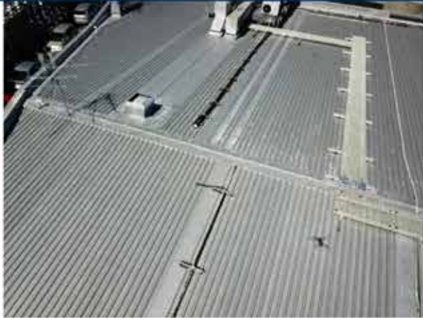
1. Areas of staining on the profiled metal roof sheets.
