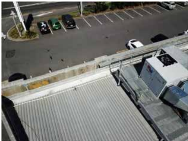
4. Staining and darkening on the internal face of the concrete parapet walls.
