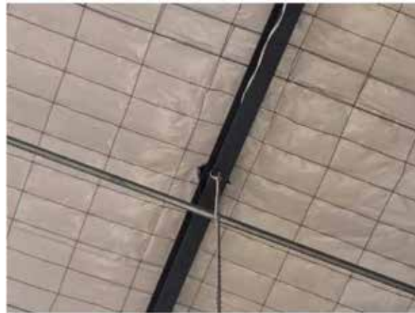
65. Minor tears to the roof underlay (Harvey Norman).
