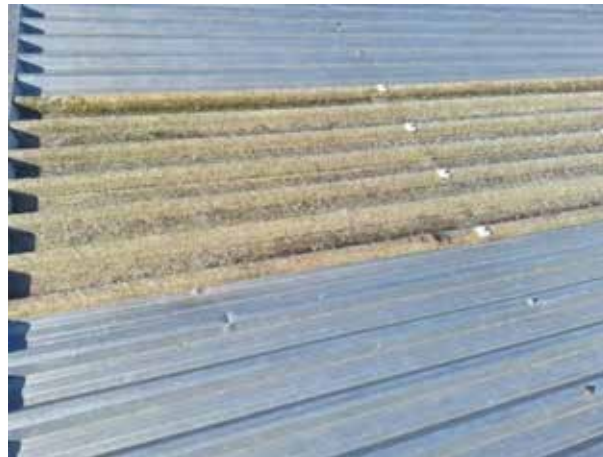
35. Sporadic areas of indentations to the profiled metal roof sheets.
