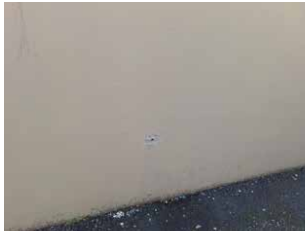
41. Localised unsealed penetration to the concrete wall panels.
