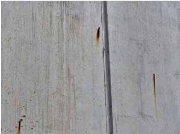
28. Sporadic areas of corrosion staining to the concrete wall panels. The corrosion staining appears to be leaching from the reinforcement bars of the concrete wall panels.
