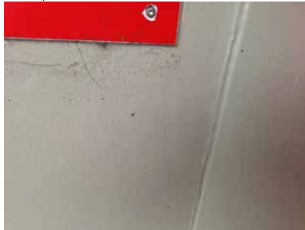
5. Sporadic areas of redundant fixing centres to the fibre-cement cladding sheets.
