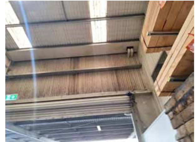
195. Widespread soil staining to the internal side of the elevations.
