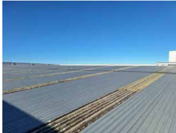
32. The fibreglass sheets were in an aged condition.
