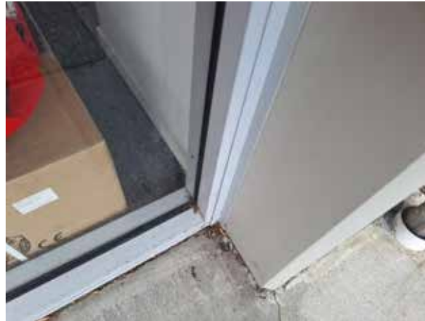
50. Sporadic areas of minor shrinkage to the glazing seals of the aluminium shop front units.
