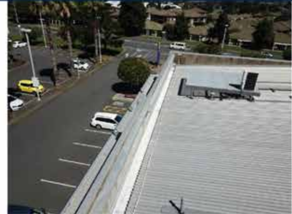
102. Staining and minor uplift to the single-plywood membrane sheets.
