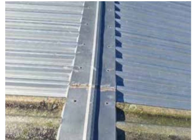
36. Localised corrosion to the joint of the metal ridge cappings.
