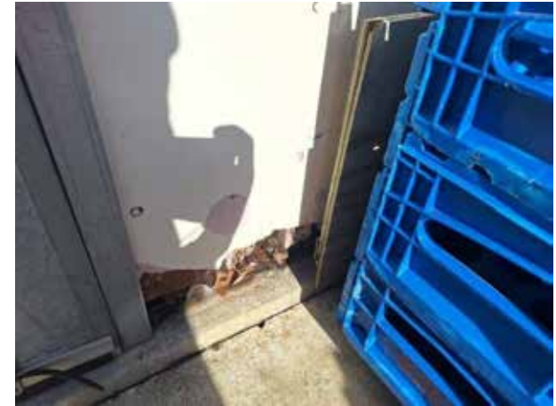
33. Localised area of extensive damage to the fibre-cement cladding sheets.
