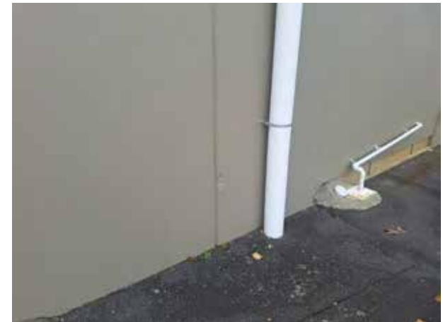
36. Sporadic areas of deterioration and spalling to the concrete wall panels.
