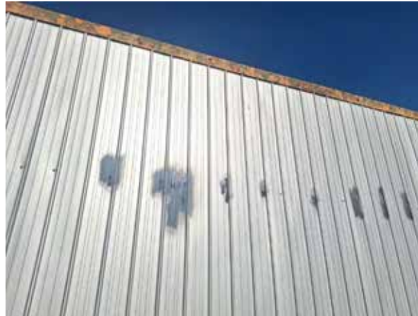
38. Localised area of discolouration to the profiled metal internal parapet sheets.
