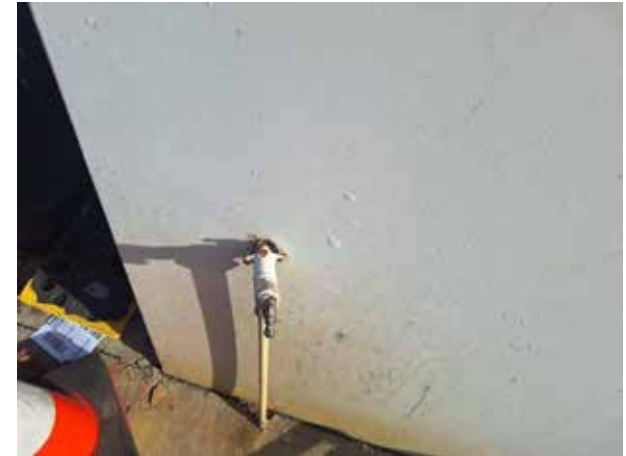
171. Localised partial detachment and corroded fixings to the tap outlet.
