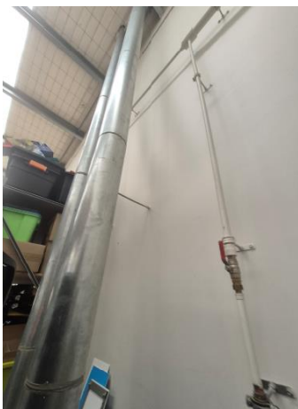
M23 – Block C tenancy WC and Kitchen extract ductwork
