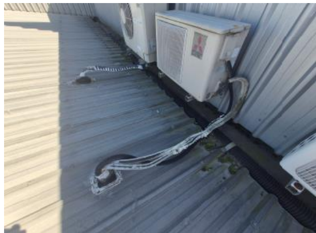
M10 – AC outdoor units with split insulation at seam leaving refrigerant pipework exposed
