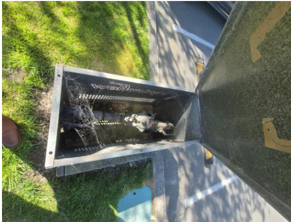
H1 – Block A & B mains incoming water complete with high hazard backflow prevention unit.
