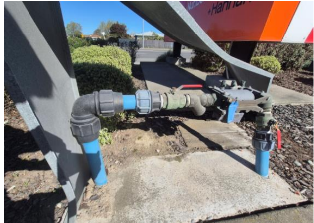
H2– Block C mains incoming water complete with high hazard backflow prevention unit. Note damaged vandal proof enclosure
