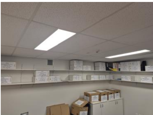
M17 – Block A & B Level 1 Admin return diffuser
