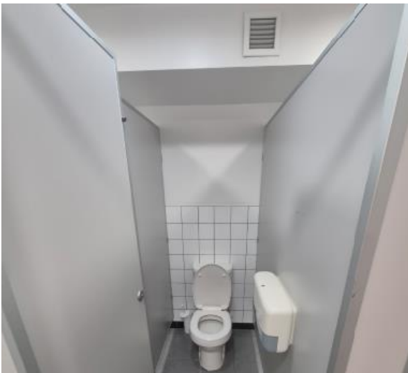
M15 – Block A & B WC extract linear diffuser
