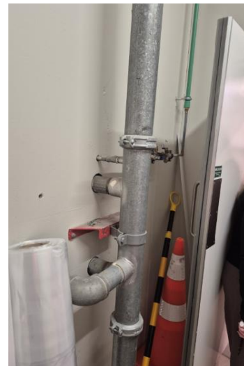
F4 – Hydrant Riser
