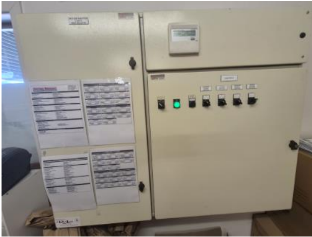
E1 – Mechanical Services DB
