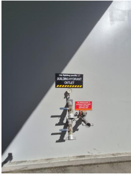
F7 – Building Hydrant Inlet at rear of Block C
