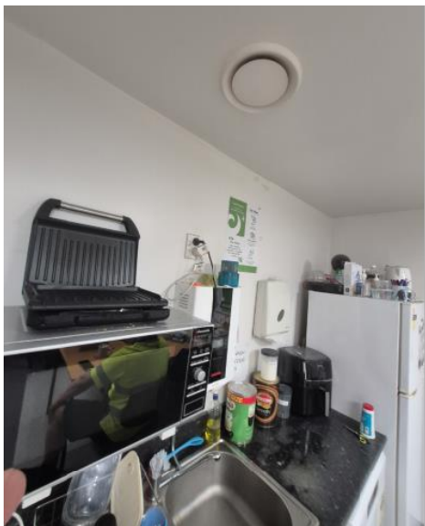
M21 – Block C tenancy staff kitchenette extract diffuser
