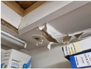
57. Block C - Moisture damage to plasterboard ceiling to 'Pet Central' mezzanine level.
