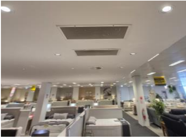
M13 – Block A & B tenancy typical return diffuser
