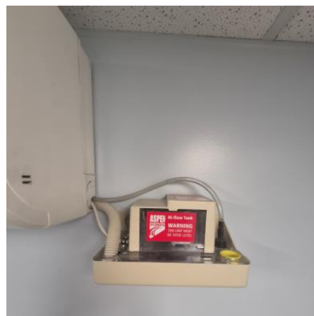
M12 – Block A & B tenancy Comms Room Hi-wall condensate pump
