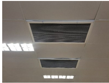
58. Block A - Reported area of moisture ingress between ventilation grilles.
