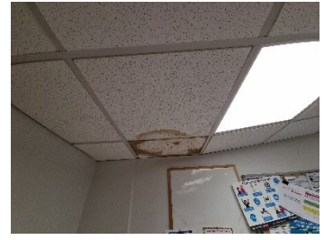
56. Block C - Moisture staining to the ceiling tiles to 'Carpet Court', mezzanine level.
