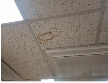
51. Block A - Moisture staining to ceiling tiles adjacent to roof access hatch.
