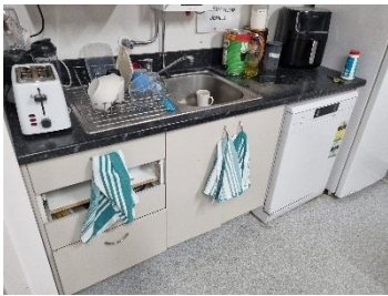
81. Block C - Typical view of kitchenette cabinetry. General wear and tear. Some cabinets damaged and reaching end of serviceable life.
