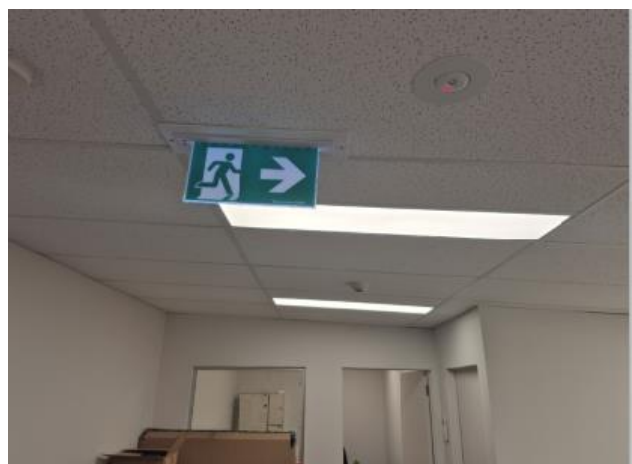
E17 – Luminated exit sign and emergency lighting
