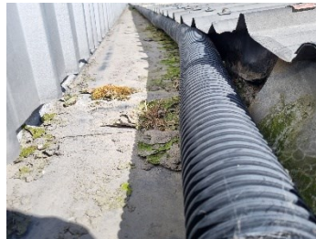
34. Block C - Coil drain installed to base of roof sheets at membrane upstand.
