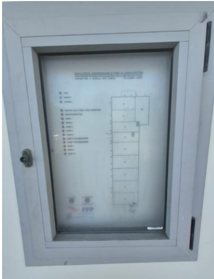
F1- Fire Alarm panel
