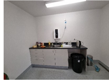
80. Block C - Typical view of kitchenette cabinetry. General wear and tear.
