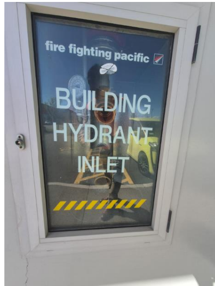
F8 – Building Hydrant Outlet
