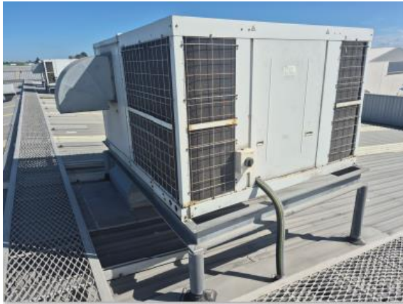
M1 – Typical Block C PAC unit
