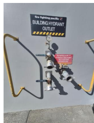
F6 – Building Hydrant Outlet – Block C
