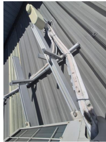
M8 – AC outdoor units with split insulation at seam leaving refrigerant. exposed
