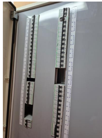
E4 – Pole fillers missing in DB
