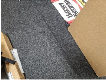
75. Block A & B - Crevices between concrete slabs to blocks are detectable beneath floor coverings, resulting in expediated wear.
