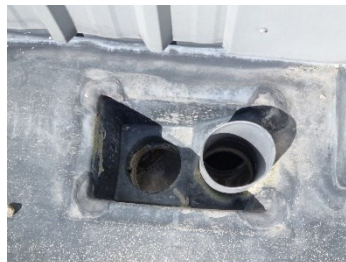
37. Block C - Lack of covers to downpipe outlets. No debris observed.
