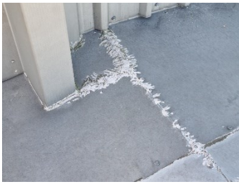
39. Block C - Sealant applied to flashing junctions in several locations across roofs.
