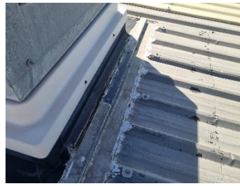
40. Block C - Sealant utilised to flashings to perimeter of service penetrations. Moisture ingress reported internally.
