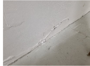
68. Block A - Moisture blistering and efflorescence to the base of the concrete wall to warehouse corridor to east.
