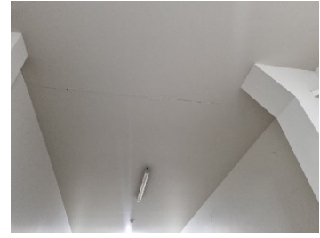
53. Block A - Hairline crack across plasterboard ceiling lining to toilet corridor.
