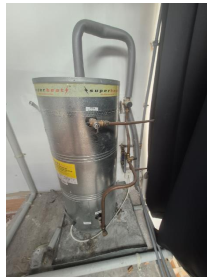
H4 – Typical hot water cylinder to each Block C tenancy
