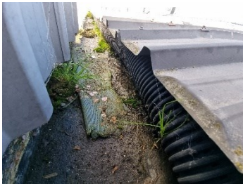
33. Block C - Vegetation and silt build-up in internal gutters throughout.
