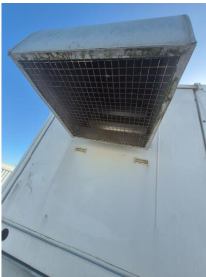
M3 – Economiser section of PAC unit
