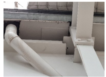
62. Block C - Moisture spotting to the underside of the internal gutter to west (Photograph, retail space 3).
