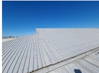
31. Block A - General view of central pitched roof covering. No anchor points sighted.
