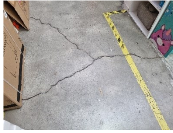
76. Block C - Cracking in concrete slabs noted to several units.
