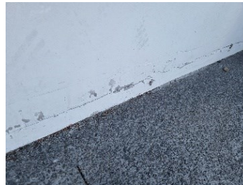
43. Block A - Peeling of painted finish and cracking to the panels.
