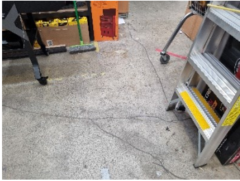
78. Block C - Cracking in concrete slabs noted to several units.
