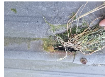
23. Block C - Roof sheets have corroded through. Vegetation growth in hole.
