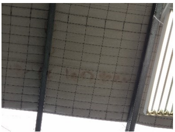
60. Block C - Moisture staining to the underside of roofing underlay to some units (photograph, 99 Bikes).
