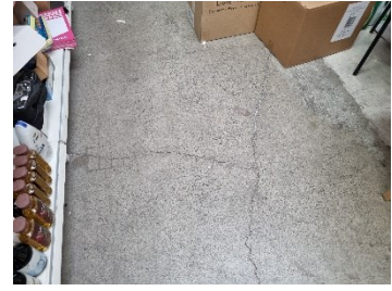
77. Block C - Cracking in concrete slabs noted to several units.
