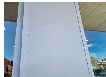
50. Block C - Hairline cracking adjacent to the windows.
