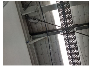
59. Block C - Moisture staining to the underside of roofing underlay to some units (photograph, Carpet Court).
