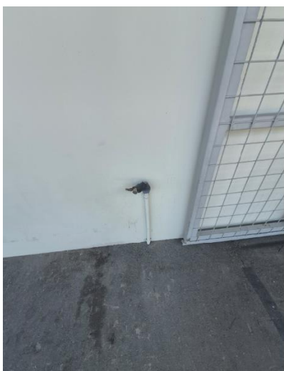
H11 –External hosetap without vacuum breaker
