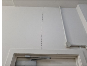
67. Block A - Vertical cracking above doorway to rear hallway.
