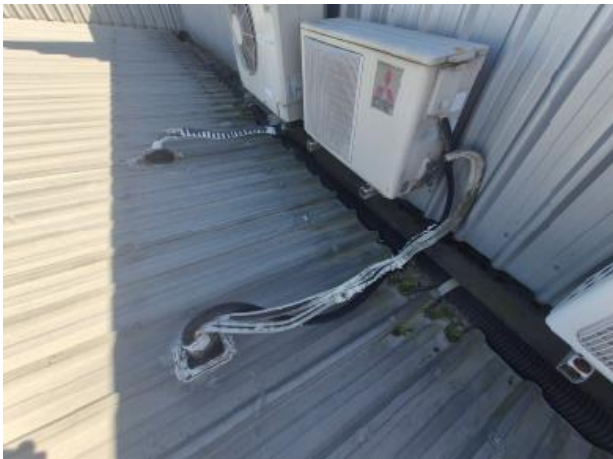
M7 – AC outdoor units with split insulation at seam leaving refrigerant. exposed
