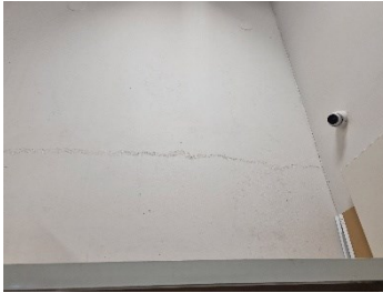
66. Block A - Cracking across interior face of east wall to warehouse corridor.
