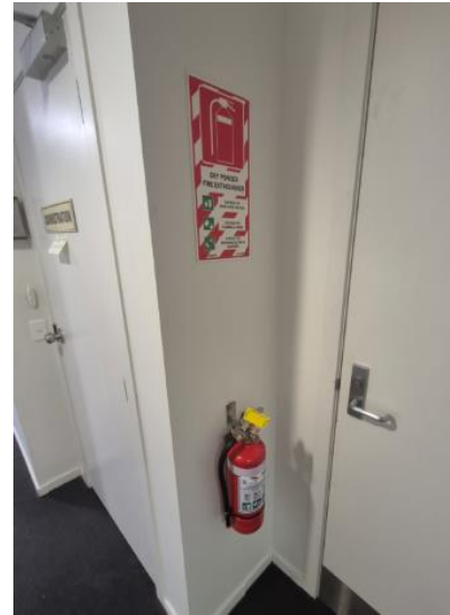
F2 –Fire Extinguisher
