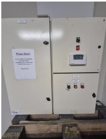
E3 - Mechanical Services DB
