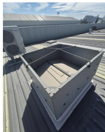
M6 – Smoke extract fan missing bird/vermin mesh
