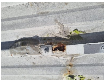
24. Block C - Roof sheets have corroded through.
