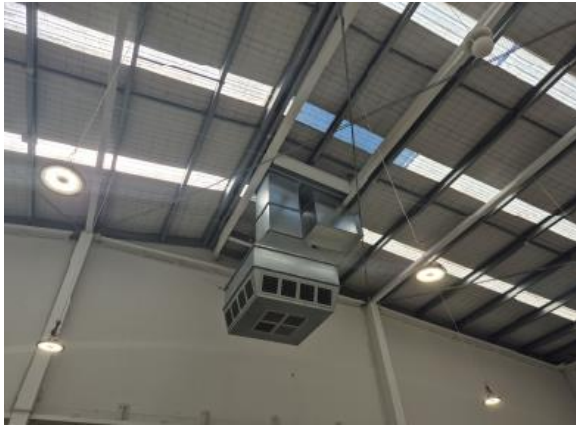
M19 – Block C tenancy typical PAC unit downward supply and return plenum diffuser
