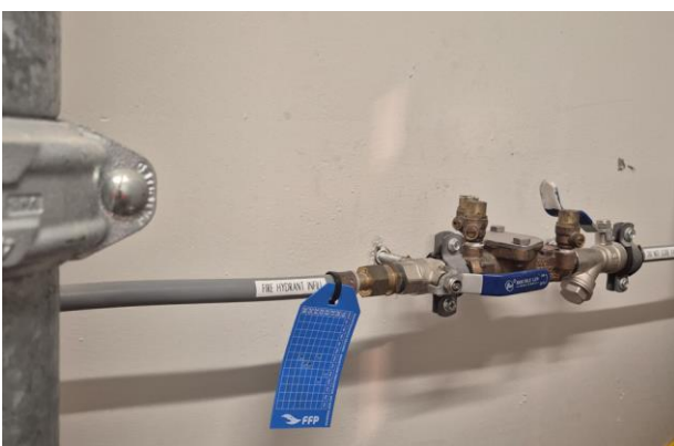
F5 – Building Hydrant water infill. Note BFP test tag due to test
