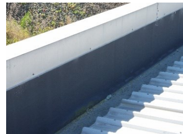
38. Block A - Vegetation growth within internal gutter.
