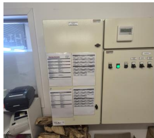
M18 – Block A & B mechanical services switchboard with Mitsubishi Lossnay controller and various fan controls
