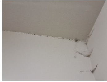
64. Block A - Cracking to the wall and ceiling junction in the rear service corridor.
