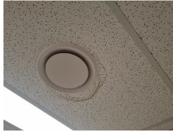
52. Block A - Moisture staining to ceiling tile adjacent to extractor fan in first level toilet.
