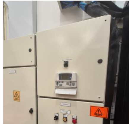
M20 – Block C PAC controller and WC extract fan controls
