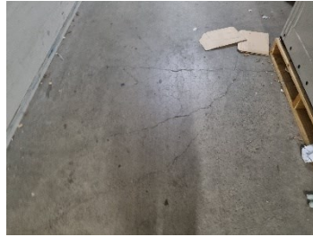
79. Block C - Cracking in concrete slabs noted to several units.
