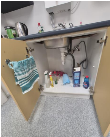
H9 – Typical plumbing within Block C staff kitchenette
