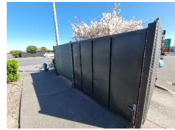
17. Impact damage to the bin storage panels.
