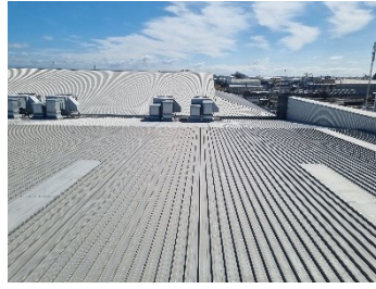
28. Block B - General view of the standing seam roofing looking from south to north.
