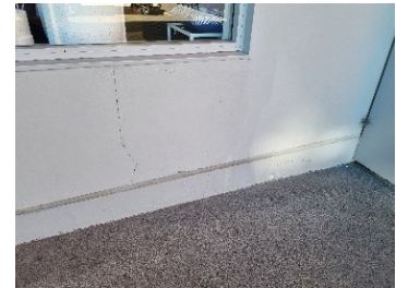
44. Block A - Cracking to the concrete panels below the windows.
