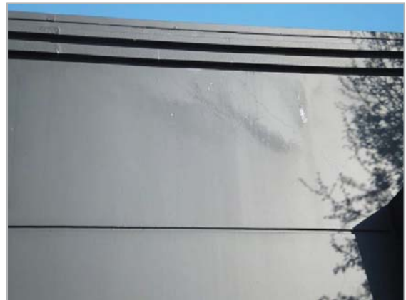
24. Deteriorated Finish to Parapet Walls, Unit 4
