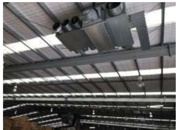
108. Cooling equipment (redundant?)
