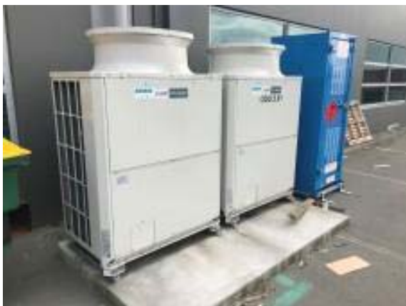
65. Air conditioning condensers
