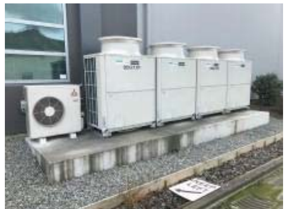
66. Air conditioning condensers
