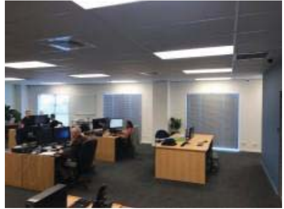
34. Ceiling diffuser air distribution
