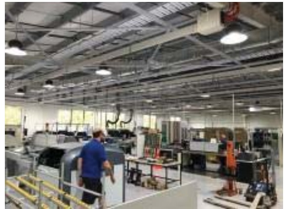
88. Power distribution rail and air conditioning
