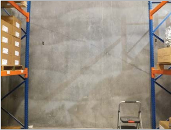
27. Diagonal Cracking to Pre-Cast Walls, Unit 6
