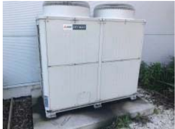
82. Main condensing unit
