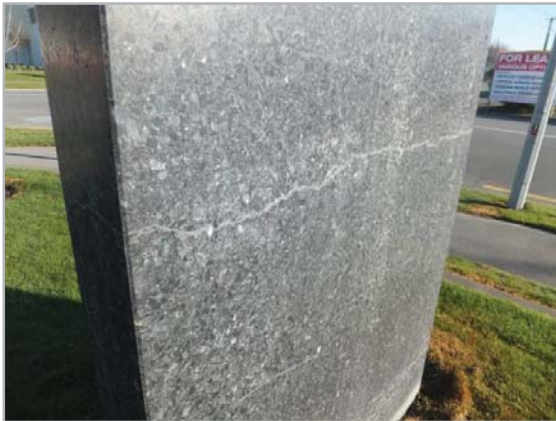
45. Horizontal Cracking to Tenant Directory Sign
