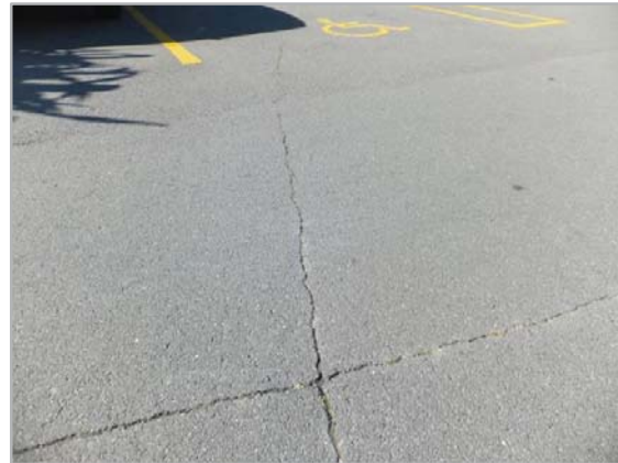
46. Cracking to Asphalt Car Park, Unit 15
