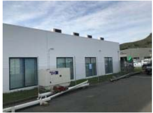
32. Air conditioning condensers
