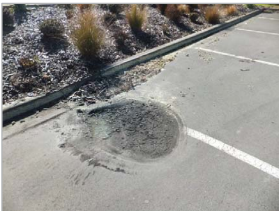
47. Settlement to Car Park, Unit 15
