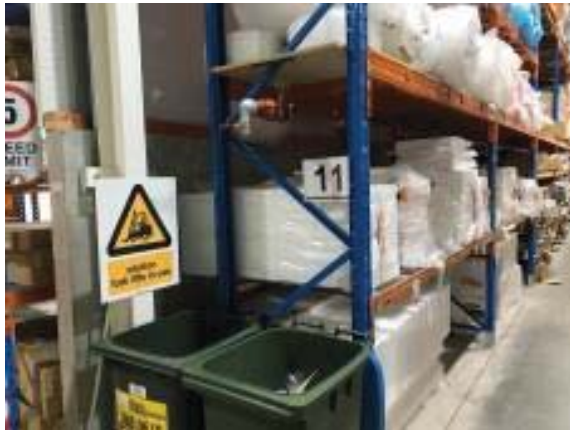
91. In rack sprinklers
