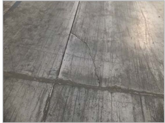
32. Typical Wear & Tear to Slab, Unit 15
