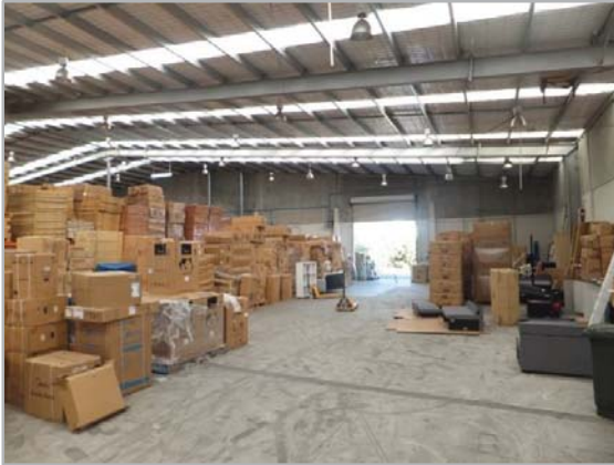
19. Typical Steel Portal Frame to Warehouse
