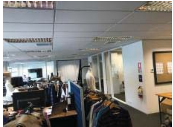
64. Office – lighting and air distribution
