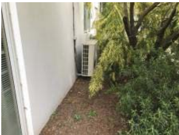
17. Air conditioning condenser
