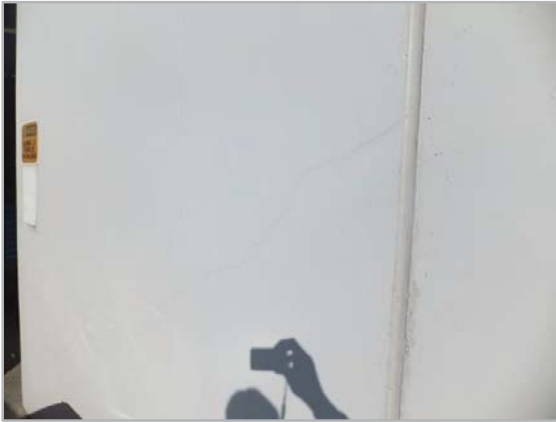
25. Diagonal Cracking to Pre-Cast Walls, Unit 4
