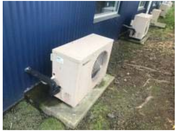
2. Air conditioning condensers
