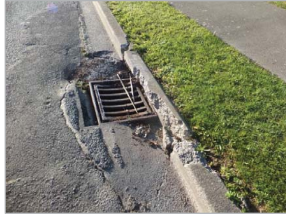
44. Example of Damaged Kerb at Drainage Gully
