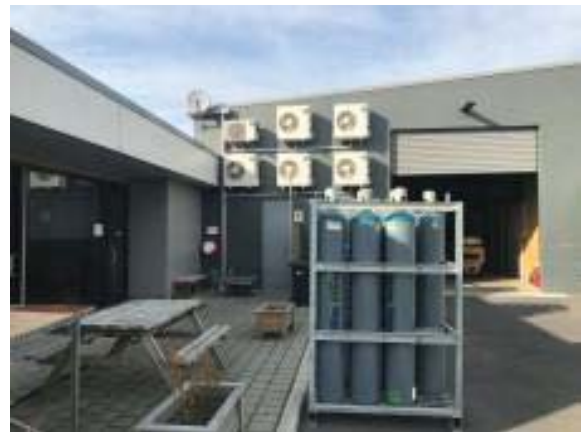
52. Air conditioning condensers
