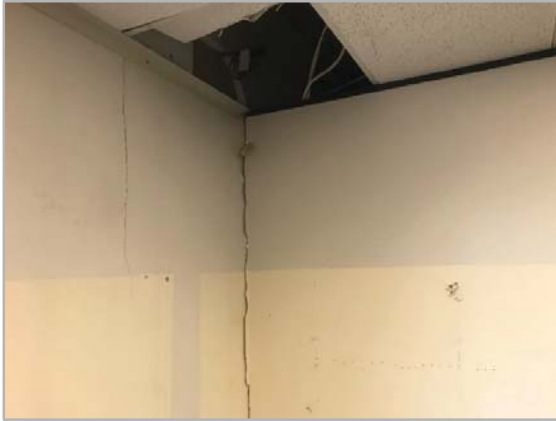
43. Cracking at Wall Junction, Unit 10A Chapmans Road
