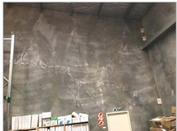
30. Cracking to Internal Face of Pre-Cast, Unit 9
