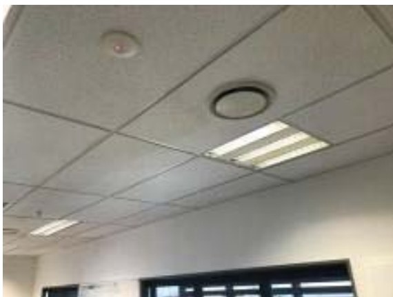
41. Air conditioning & emergency light
