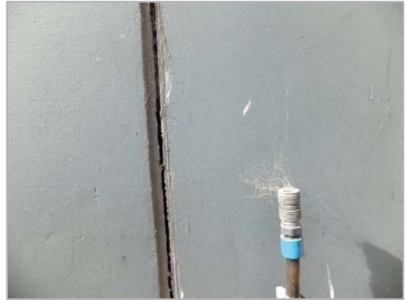
28. Failed Sealant to Pre-Cast Panels, Unit 9
