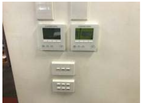
54. Air conditioning controls
