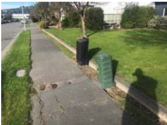
5. Power pit box
