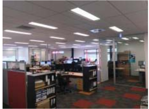
56. Swirl diffusers, sprinklers, and lighting
