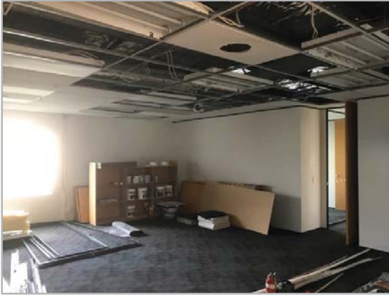
37. Internal Area Requiring Refurbishment, Unit 10A Chapmans Road
