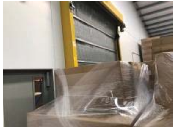
102. Non fire rated door between tenancies
