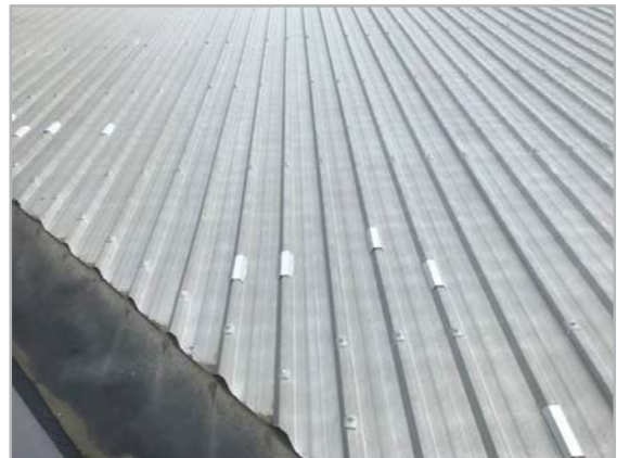
22. Unit 11 Roof Sheetting with Evidence of Repairs
