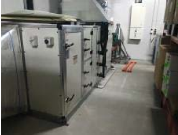
73. Tenant mechanical services
