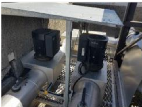
M17 – Chilled water pumps and pipe work on Roof
