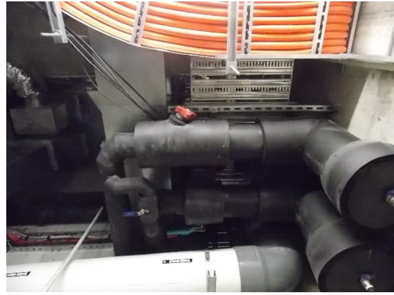
E2 – Unsupported cabling in MSB Room
