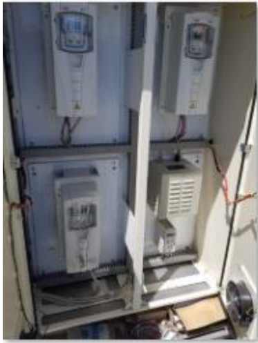
M15 – HVAC Roof mounted VSDs
