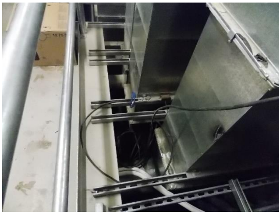
E3 – Unsupported cabling in riser
