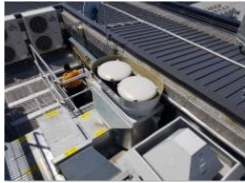
M12 – Roof Fans
