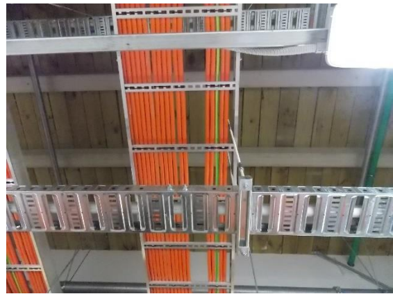
E4 – Non-compliant spacing between hanger and cable ladder
