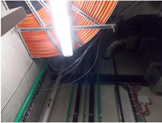
E1 – Unsupported cabling in MSB Room
