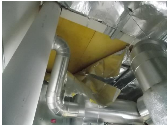
E5 – Aluminium lining above generator coming off
