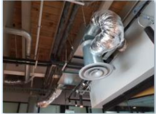
M4 – Typical exposed supply duct and Grille
