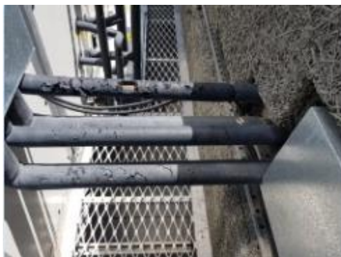
M20 –DX refrigerant pipework on Roof in need of repair and UV protection.
