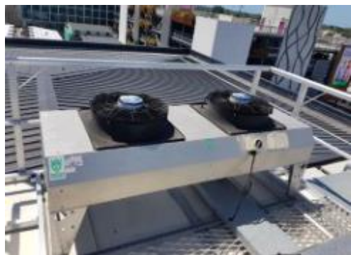
M19 –HVAC Dry cooler on top of AHU
