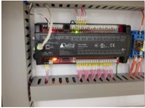
M9 – HVAC Controller
