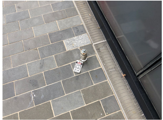
1.26. View of gas supply point
