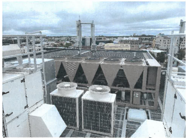
Rooftop Chiller Plant Units
