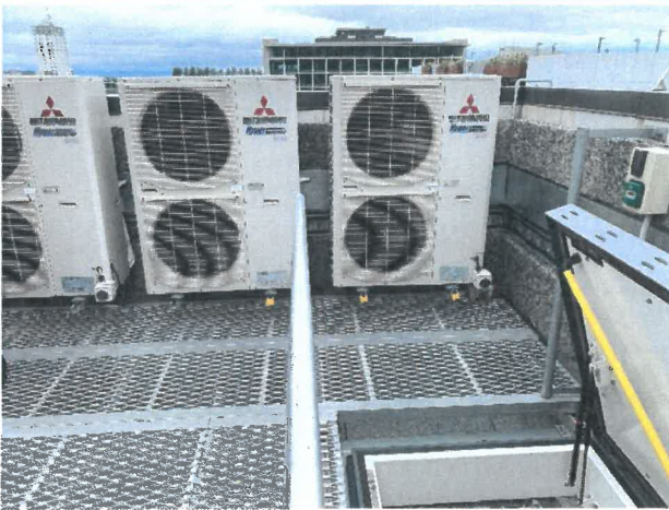
Rooftop AC Units
