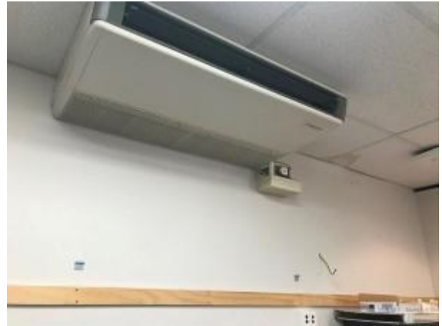
Ceiling hung split unit
