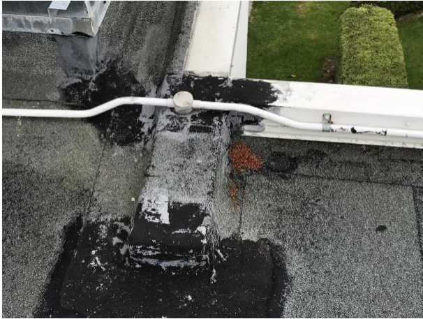
B1 – sealed junctions worn & solar degrading
