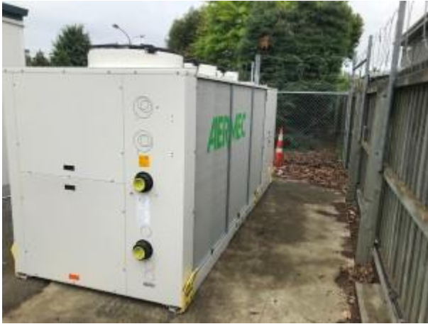
New Aermec chiller waiting to be installed
