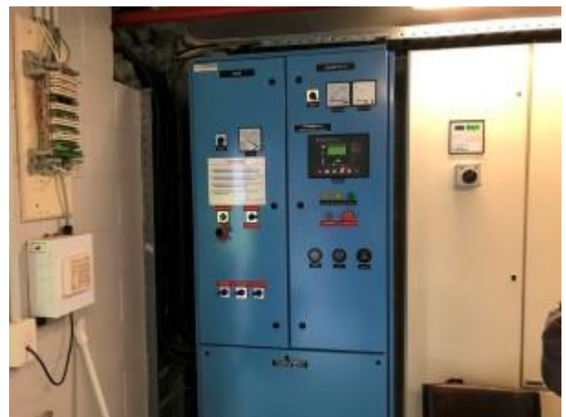
Automatic transfer switch cabinet
