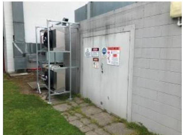
Air cooled CRAC condensers
