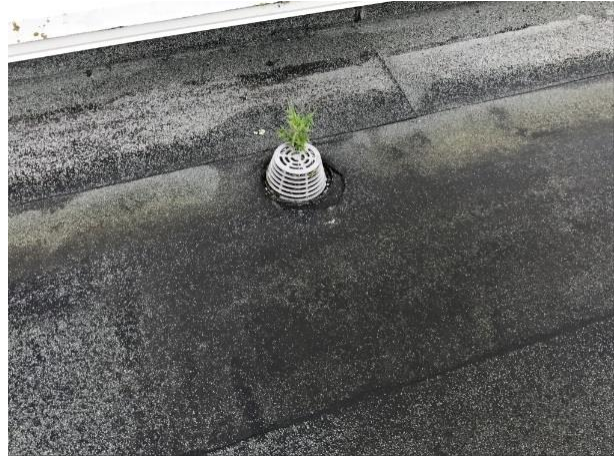
B1 – choked outlet despite grate being fitted.
