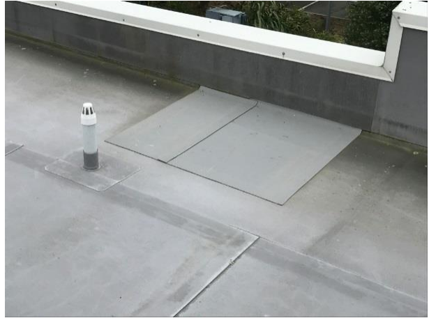
B2 – Patch repairs evident
