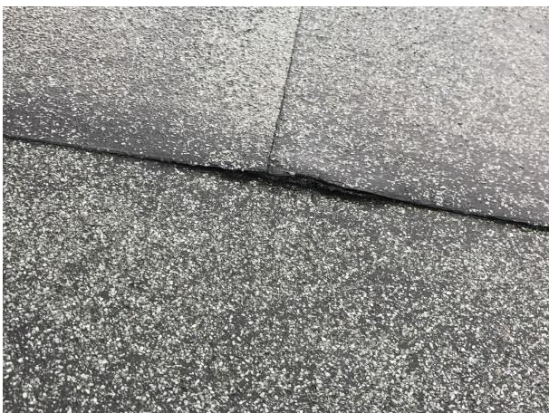
B1 – joints starting to lift at lapped edges
