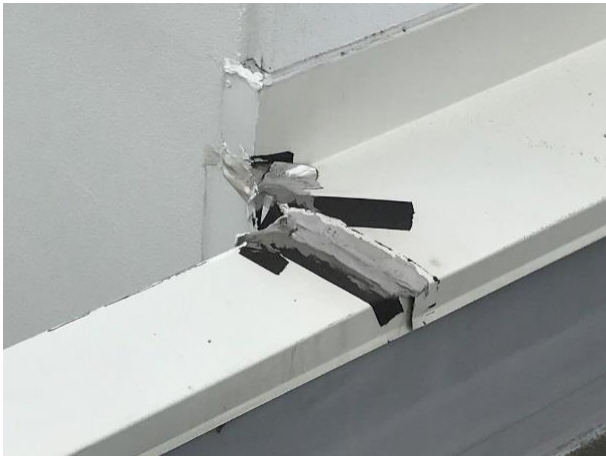
B2 – Poor patch repairs to cap flashing joint
