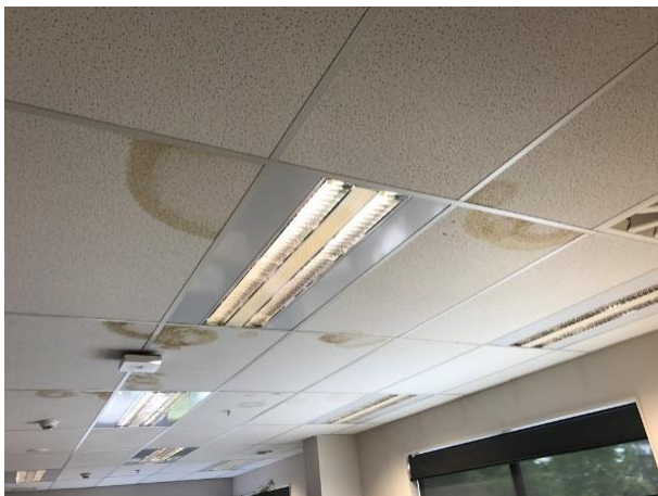
B2 – Stained & damaged ceiling tiles north end
