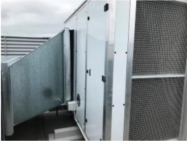
Outside air preconditioner
