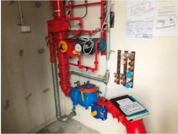
Sprinkler valve set
