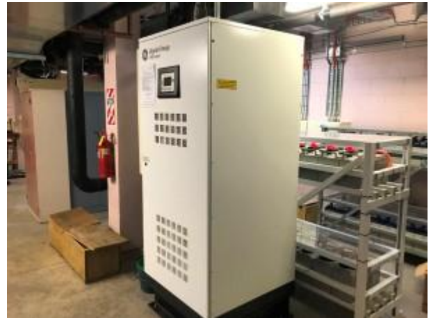
UPS and Batteries (Tanat owned)
