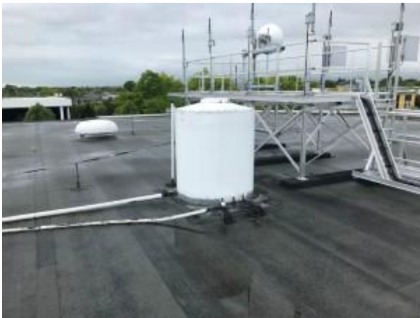
Cold water header tank
