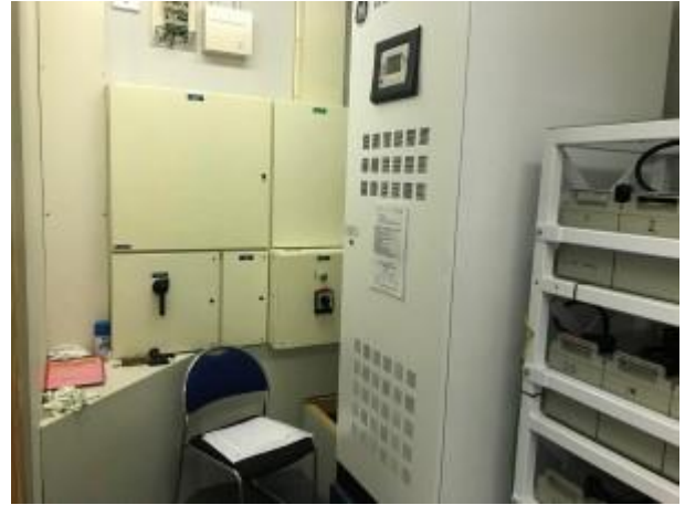
Distribution board – bespoke to the tenant
