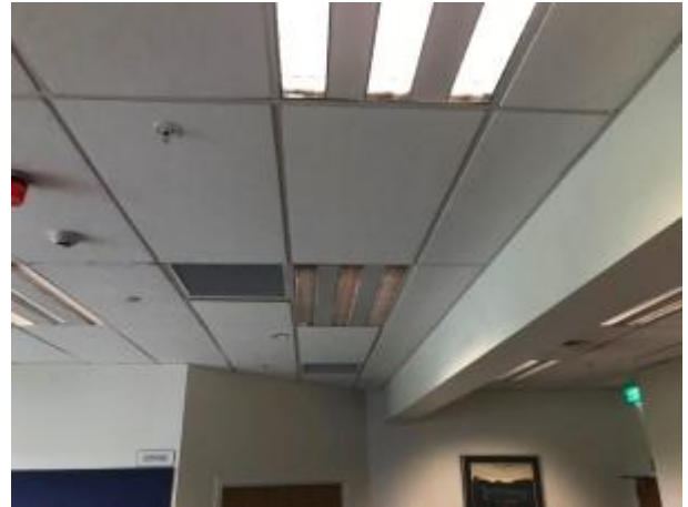
VESDA (Tenant owned)
