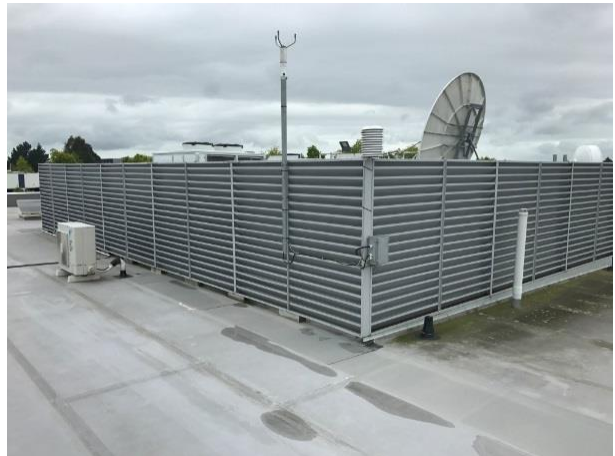
B2 – louvred plant enclosure
