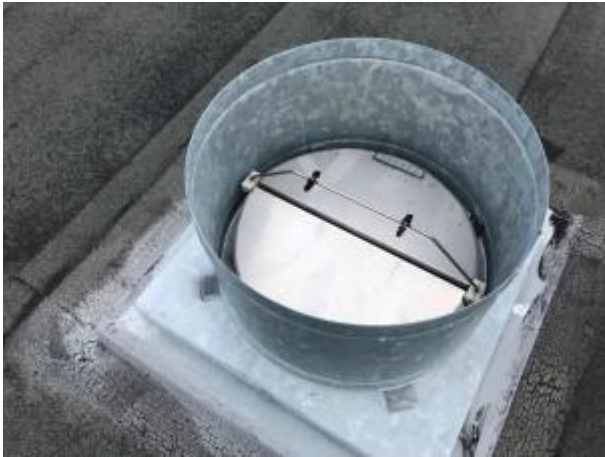
Heat relief fans – (suspected of being smoke relief)
