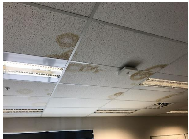
B2 – Stained & damaged ceiling tiles north end
