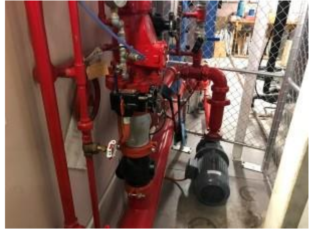
Sprinkler valve set
