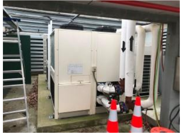
Old Multistack chillers
