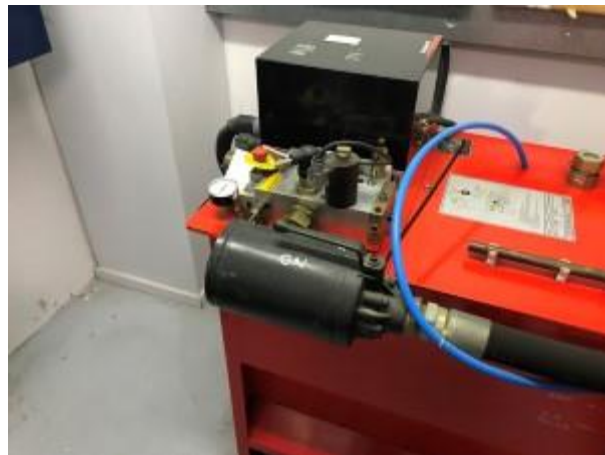
B1 - oil tank & pump
