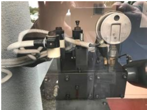
B2 - oil tank & pump
