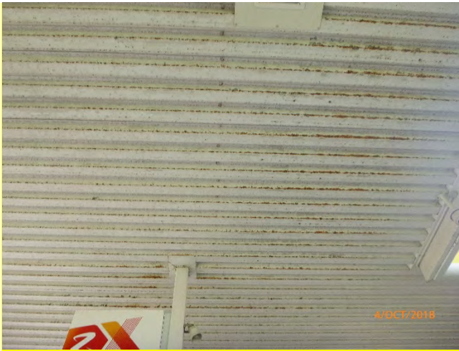
Photograph 26 Early corrosion underside of Z fuel station canopy roof.
